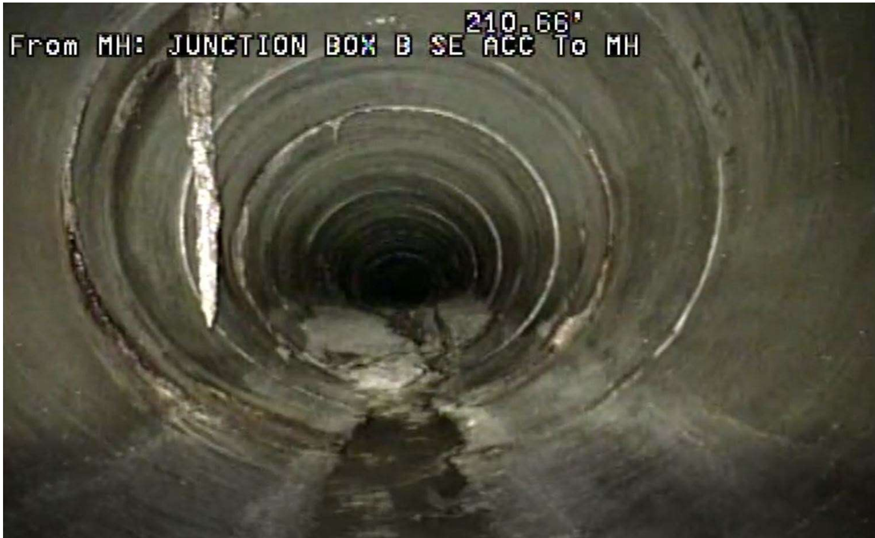
Tree roots, minimal water flow, pile of hardened concrete, 211 feet from manhole
