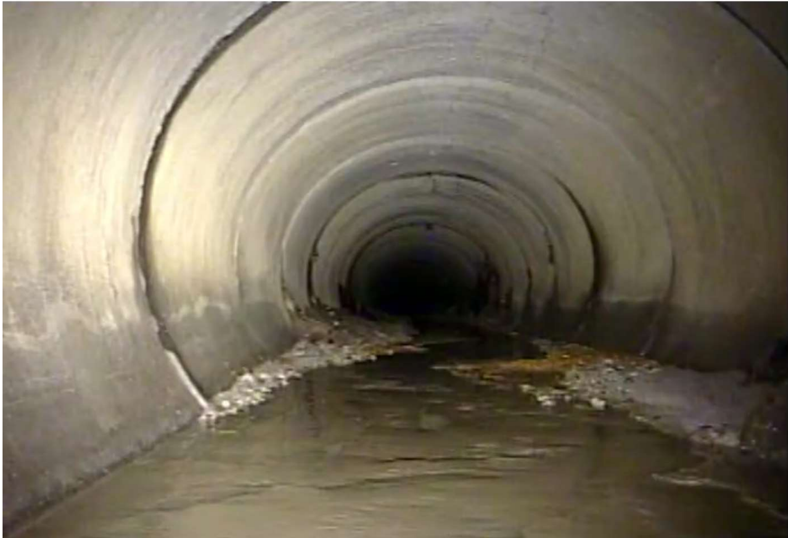
Heavy sediment accumulation, end of inspection, ~375 feet north of outfall manhole
