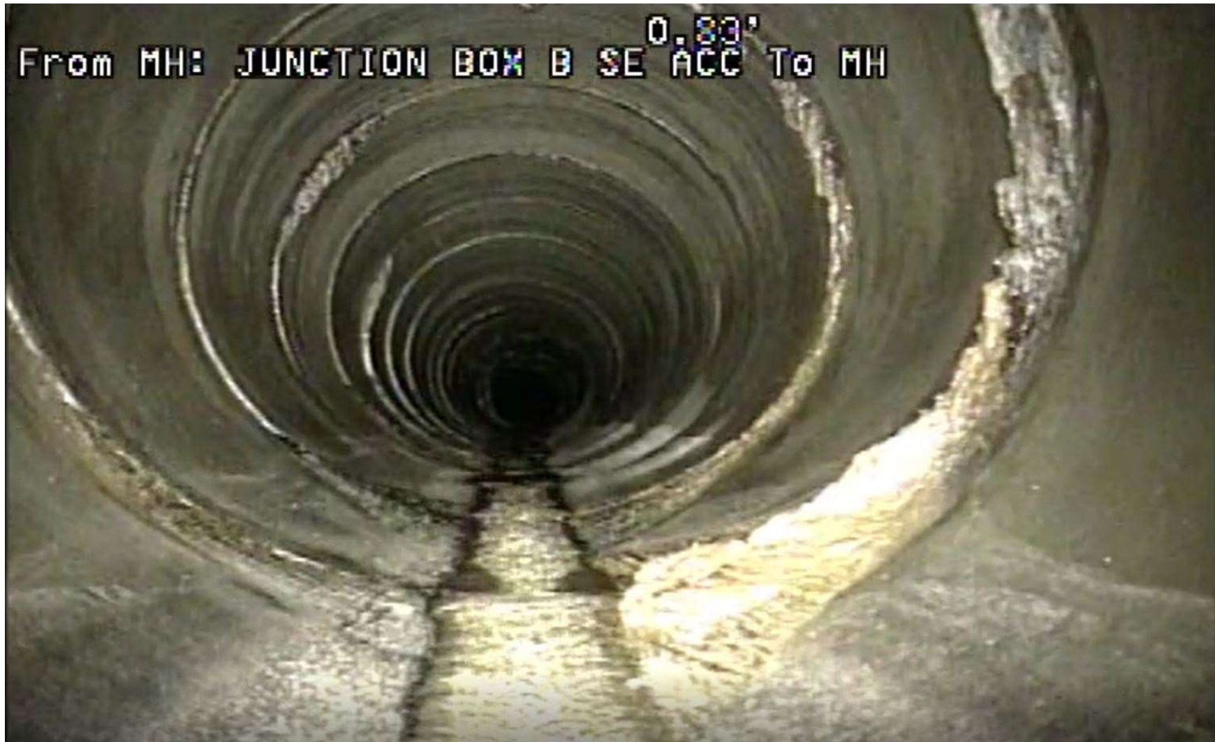
Start of inspection at Junction Box B access manhole Approximately ¼" water flow, minimal sediment, evidence of groundwater infiltration
