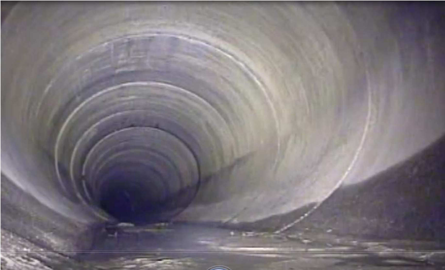
Start of inspection at entrance to 54" outfall main. Minor water flow (pre-outfall manhole fill), minor sediment
