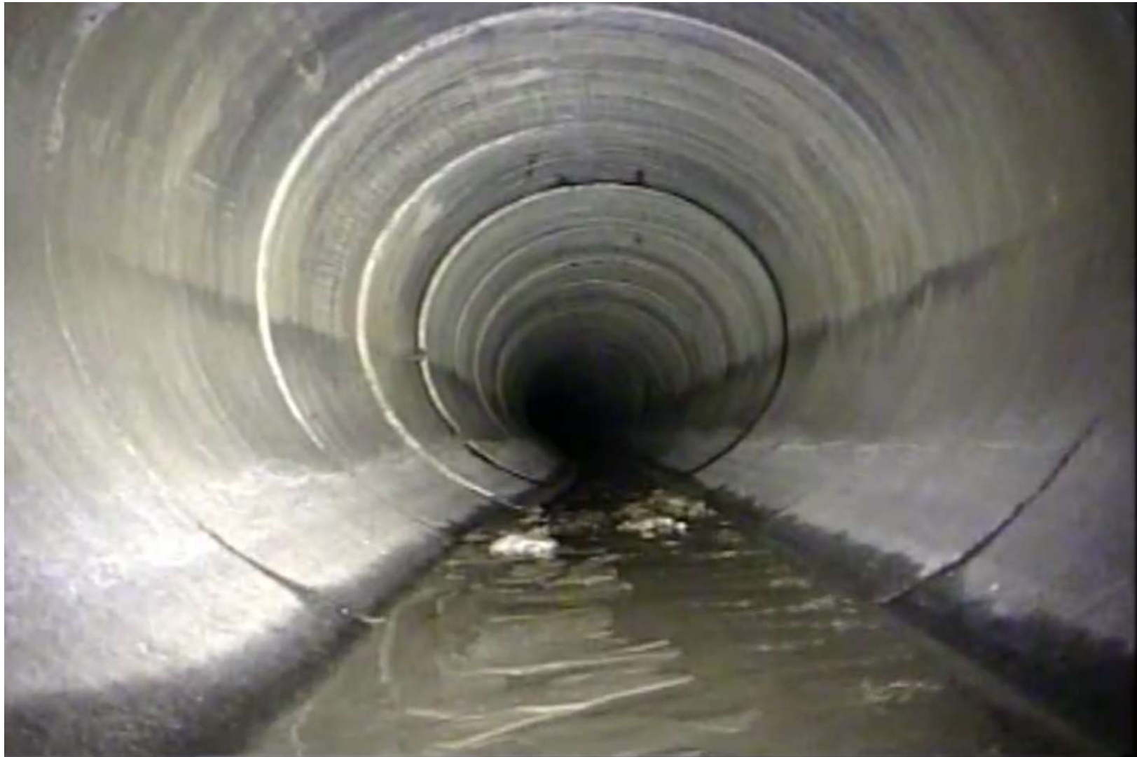
Minor sediment accumulation, evidence of infiltration through pipe joints at ~30 feet
