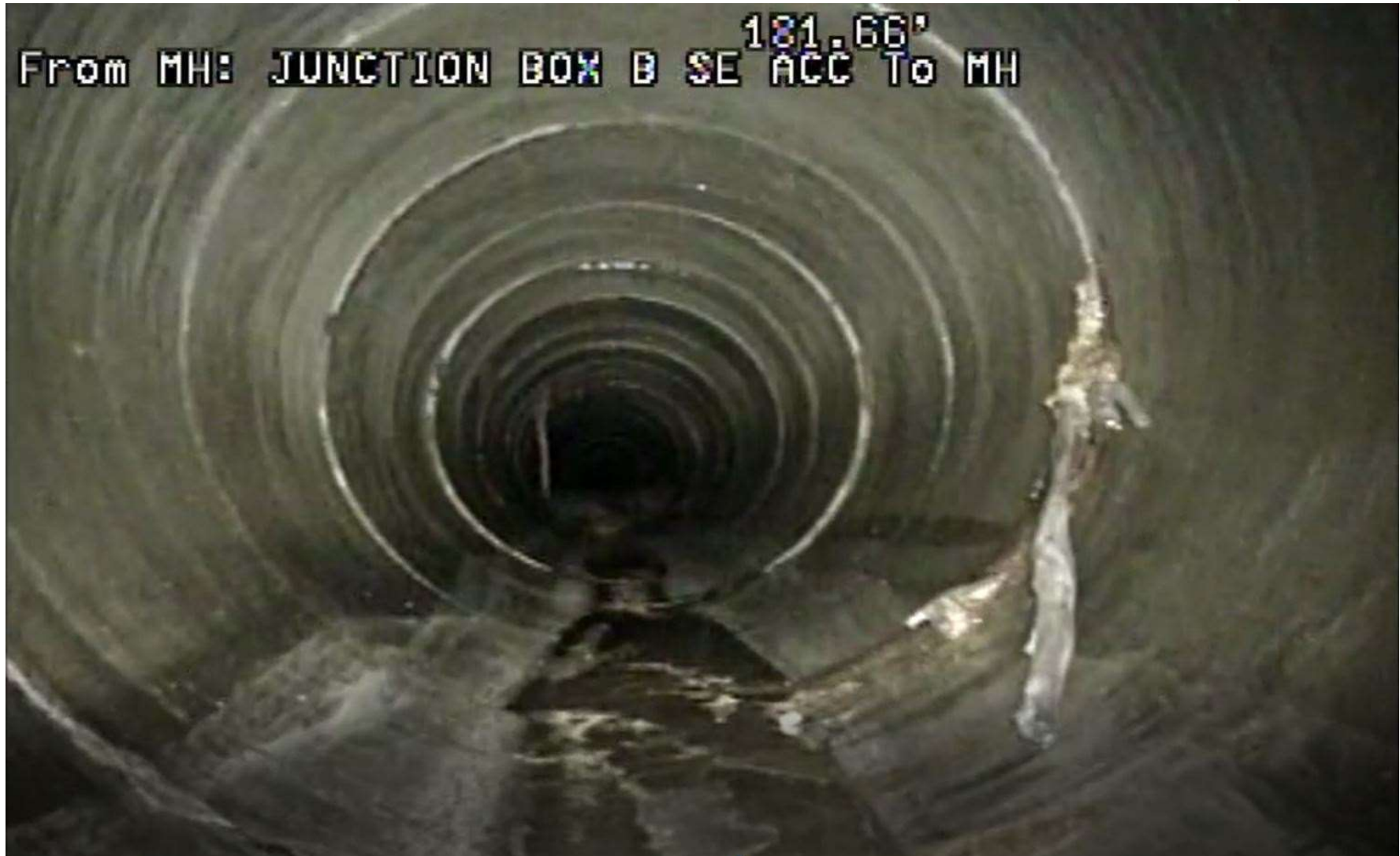
Minimal sediment, minimal water flow, possible tree roots, 182 feet from manhole
