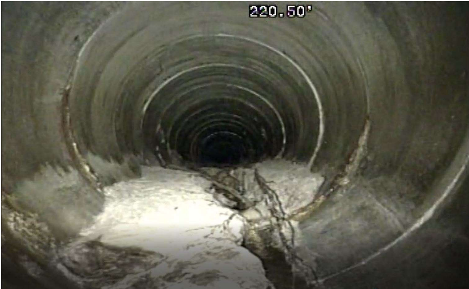
Pile of hardened concrete, end of inspection, 220 feet from manhole
