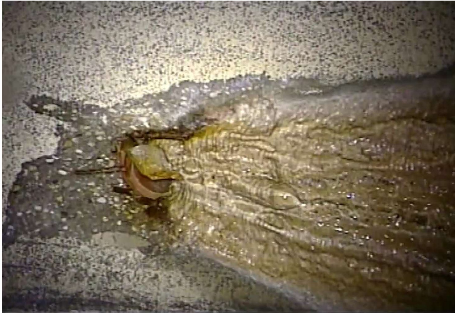
2 or 3 inch diameter pipe intrusion, ~150 feet north of outfall manhole
