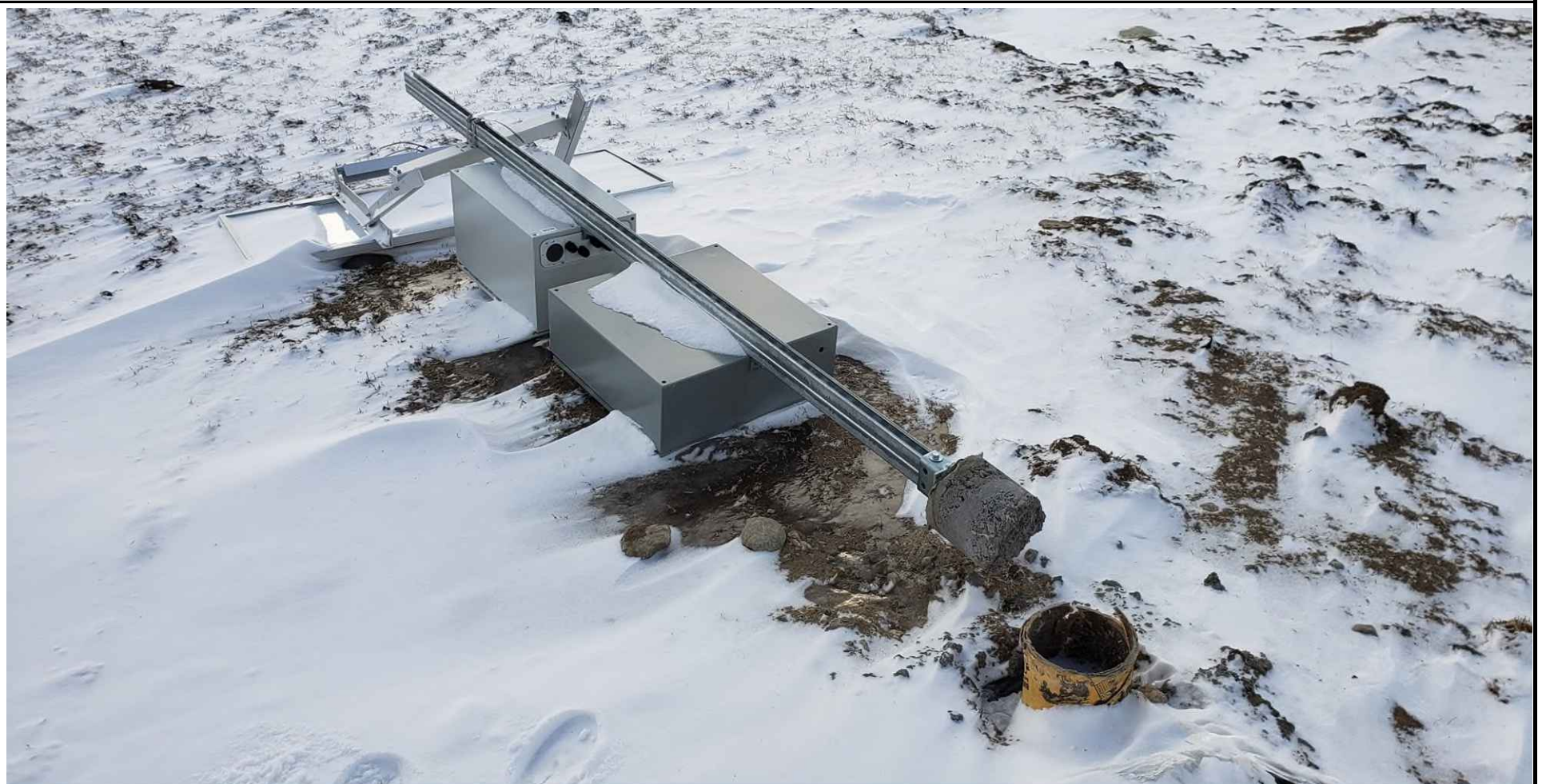
1/25/19 - Injection well pole mounted equipment that fell over.
