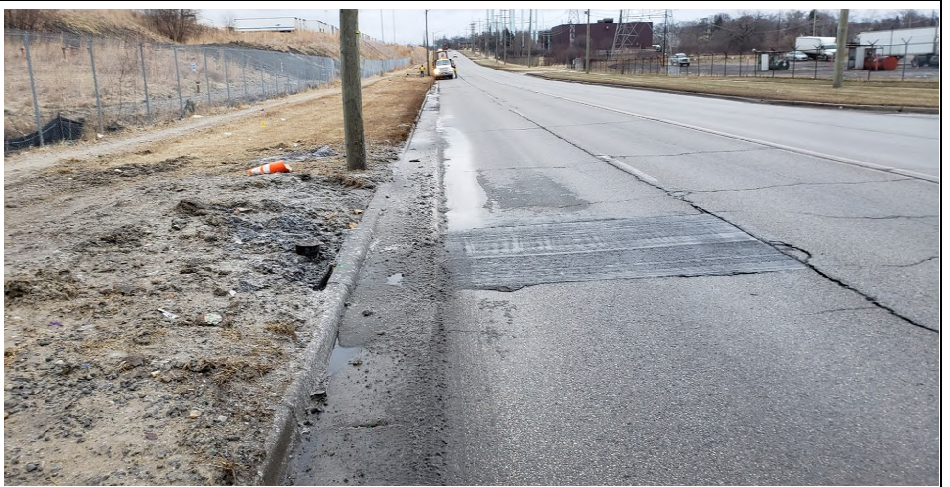
1/16/19 - Photo of Montcalm Road facing east (Oakland County WRC repair area in foreground)
