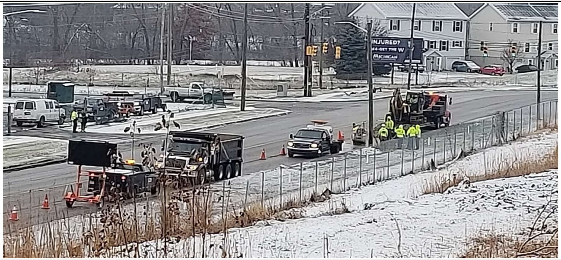
12/13/18 - Oakland County Water Resource Commission saw cutting at suspected Montcalm water main leak location.
