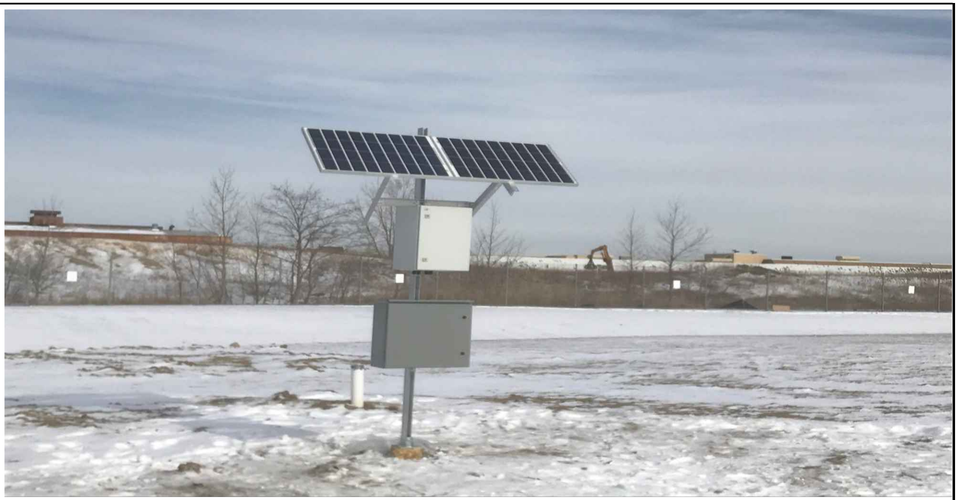
1/22/19 - Injection well pole mounted equipment.
