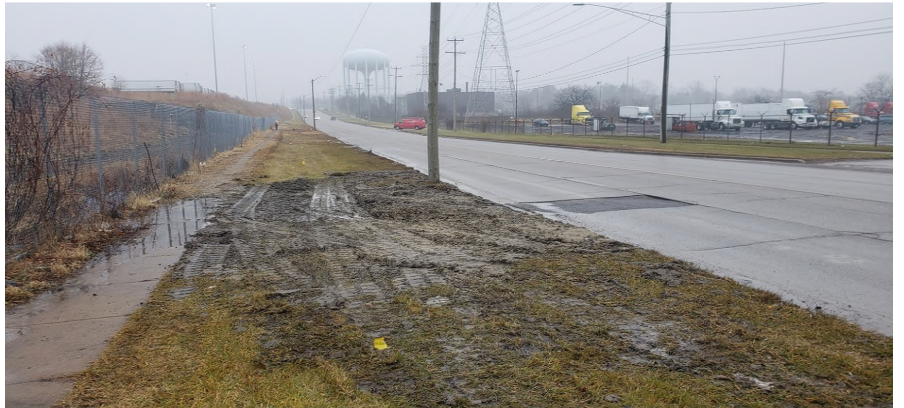
12/14/18 - Oakland County Water Resource Commission patched road and work area along Montcalm at water main leak location.
