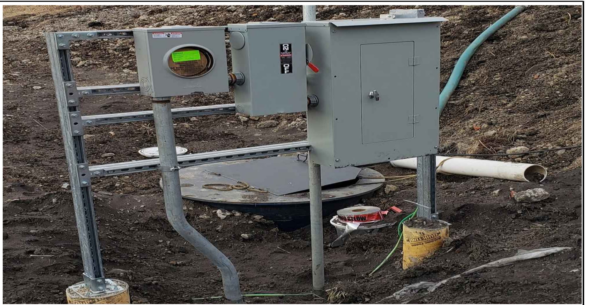
1/11/19 - Meter revisions completed.
