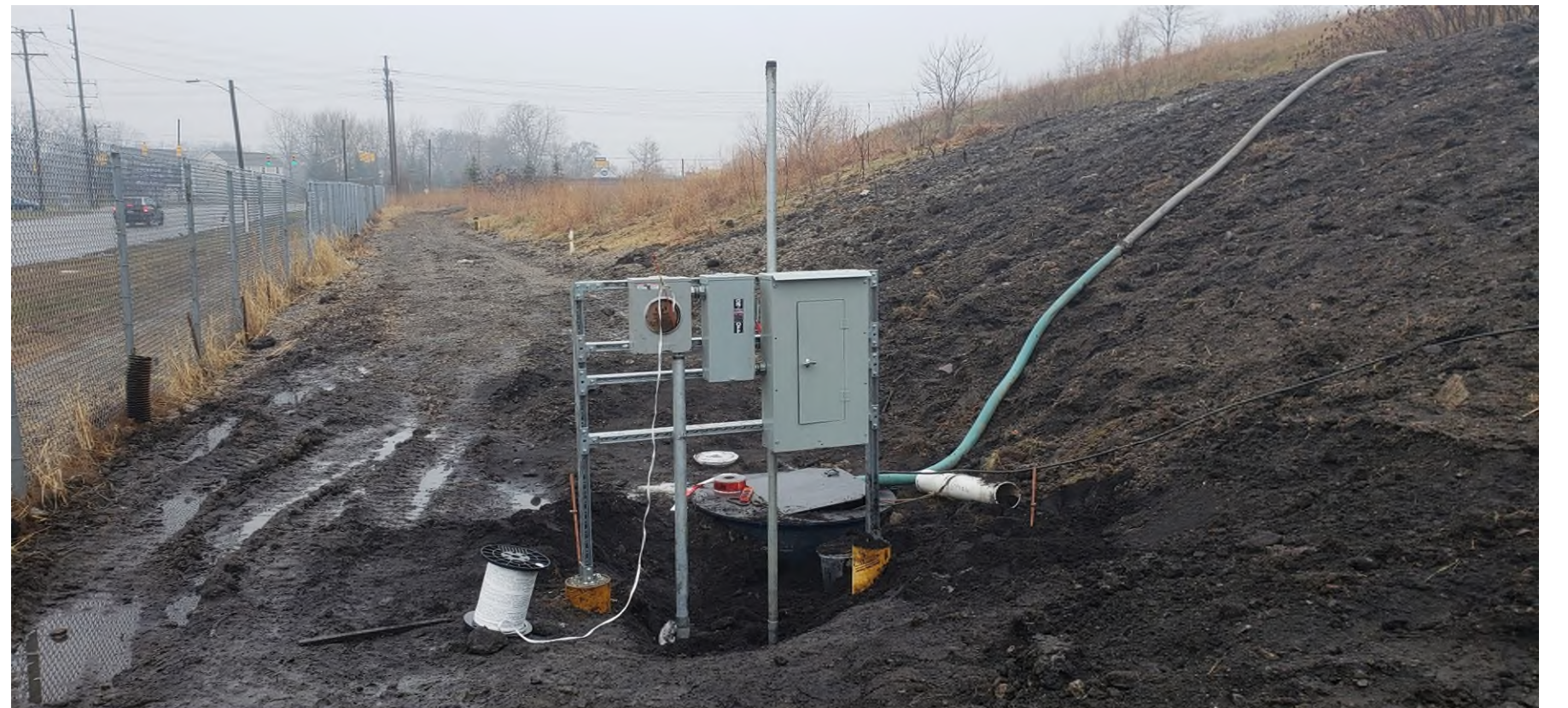
12/14/18 - Electrical rack under construction. Motor city completed conduit run, and mounted equipment to rack.
