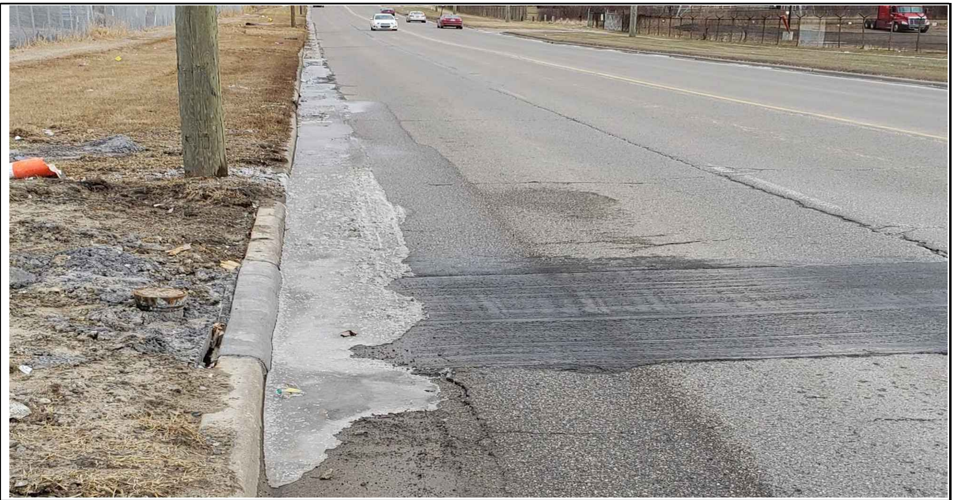
1/11/19 - Photo of Montcalm Road facing east (Oakland County WRC repair area in foreground)
