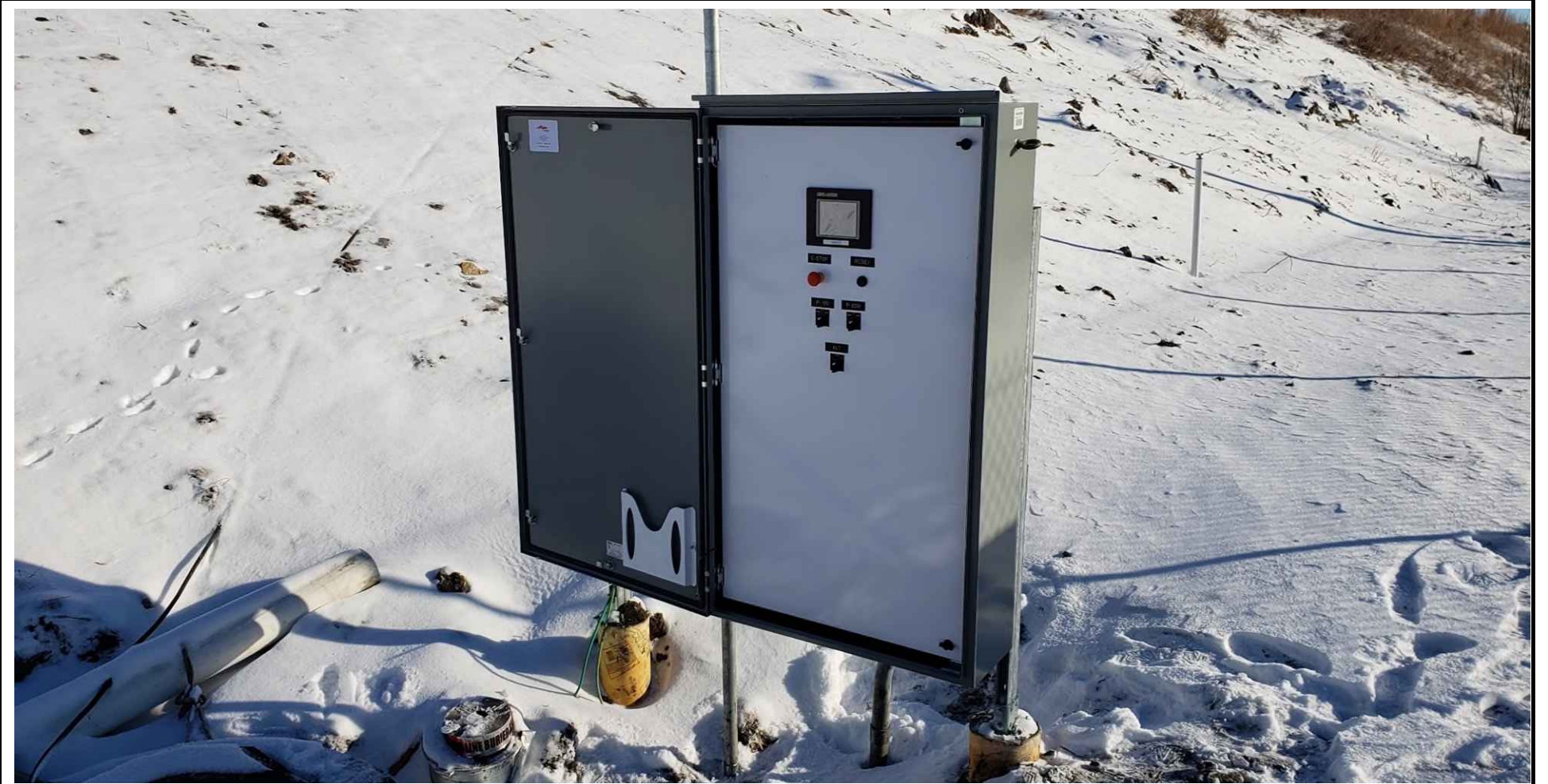
1/21/19 - Sump control panel mounted, exterior door open.
