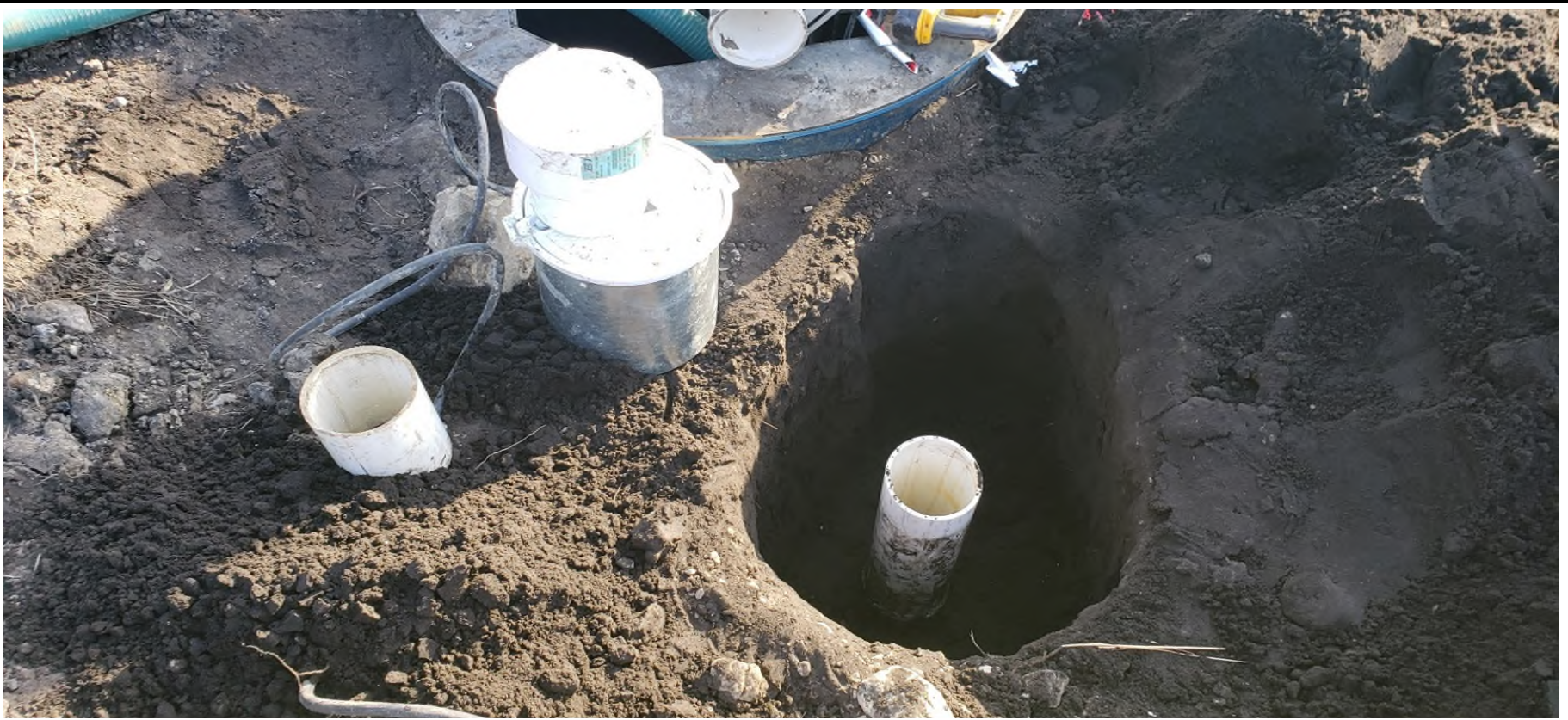
12/05/18 - Strainer cleanout at sump being finished to grade with 6"x8" transition and vault
