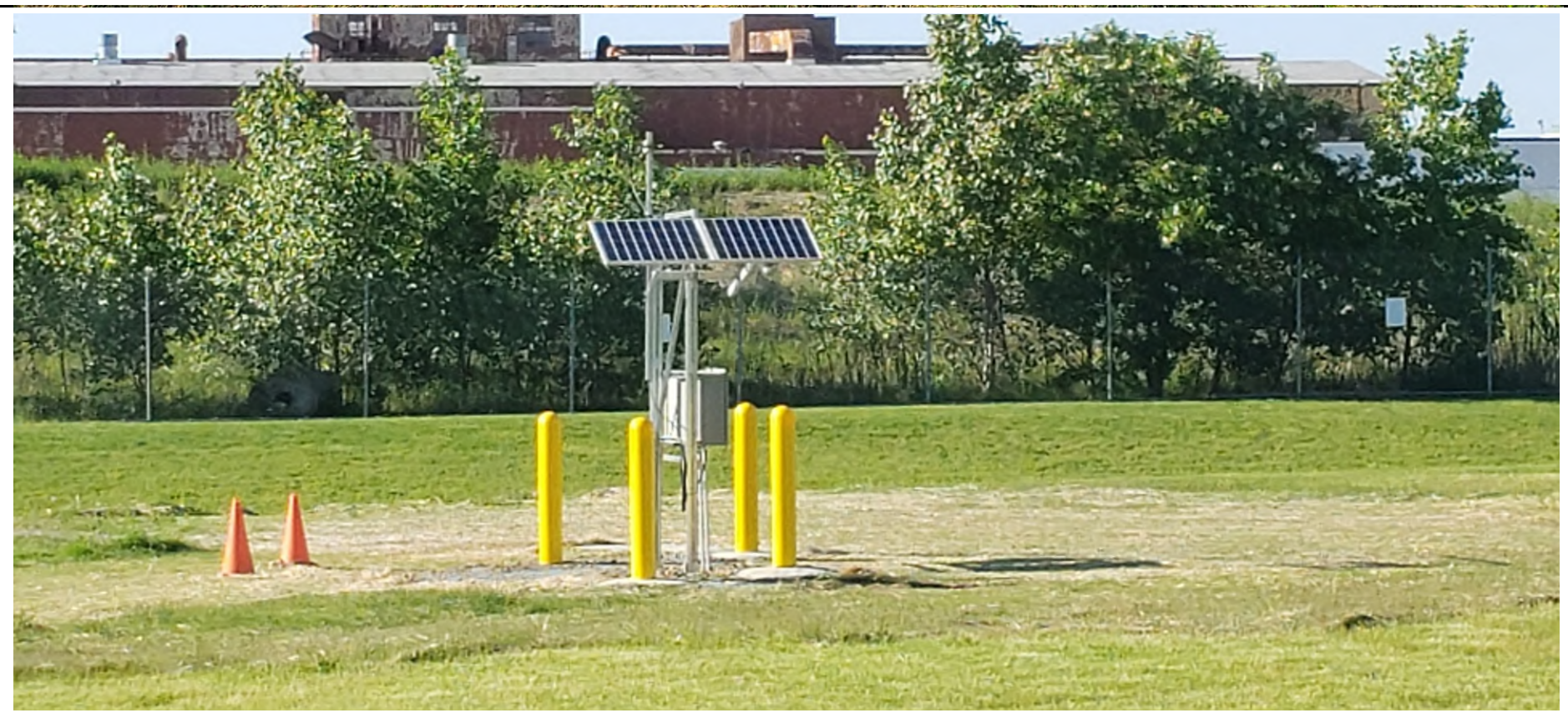
Injection control panel
