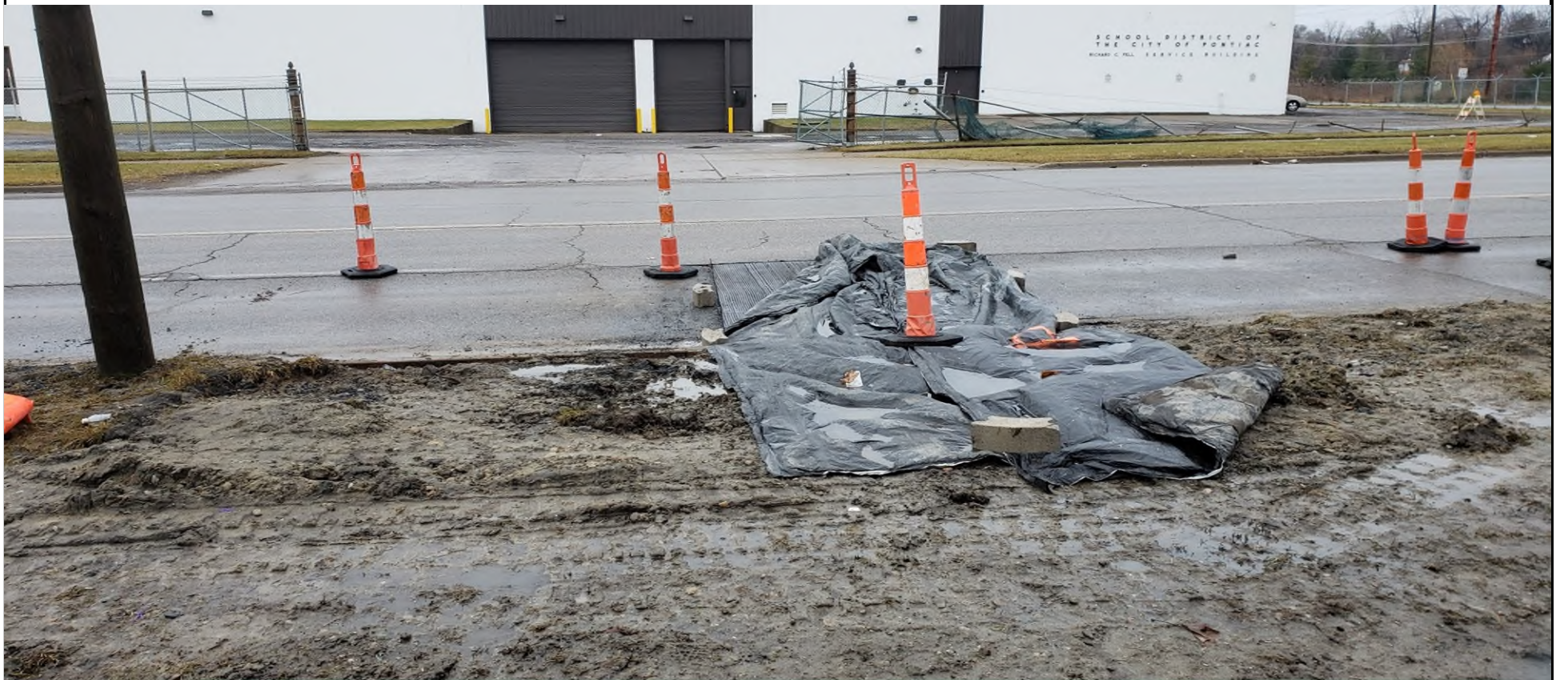
12/21/18 - Photo of isolated area along Montcalm St. where Oakland County WRC water line repair work was conducted.
