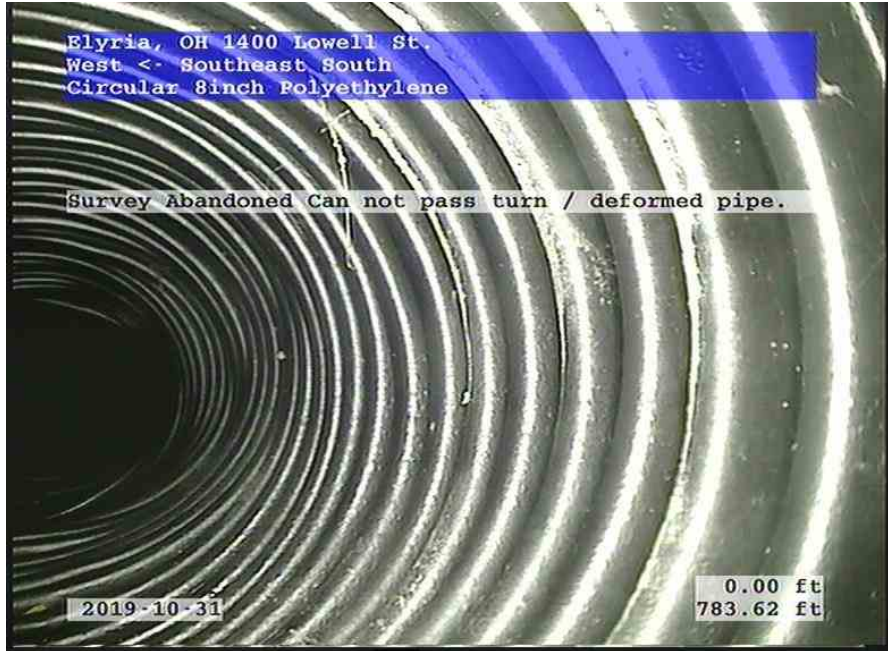
West-Southeast South_5597f453-186e-4af6-8b83-b93b28778e1e_20191031_144431_440.jpg, 00:38:32, 783.62ft Survey Abandoned
