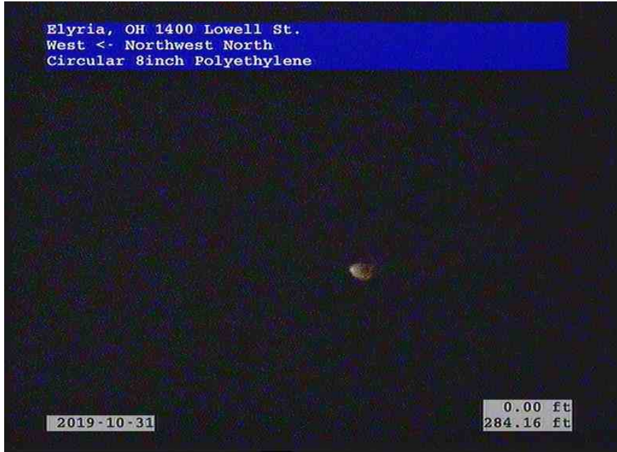
West-Northwest North_e7581d69-34c0-4206-804a-650cc7b137ea_20191031_170647_860.jpg, 00:19:25, 283.05ft Tap Factory Made at 9 o'clock, 8inch dim
