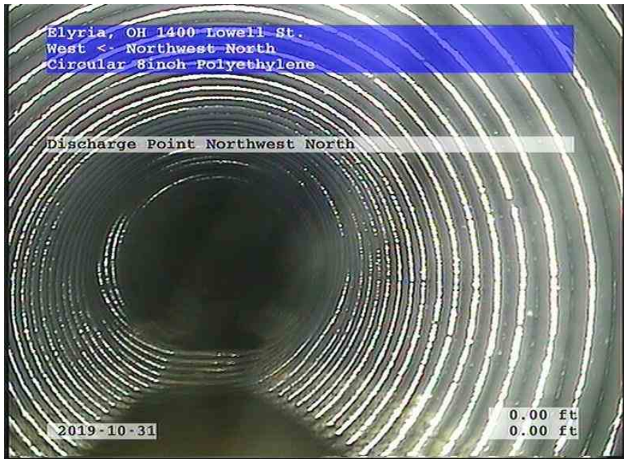
West-Northwest North_cb81c48d-c1ea-4d3c-8d46-3f402b0332e8_20191031_164420_799.jpg, 00:00:00, 0.00ft Discharge Point
