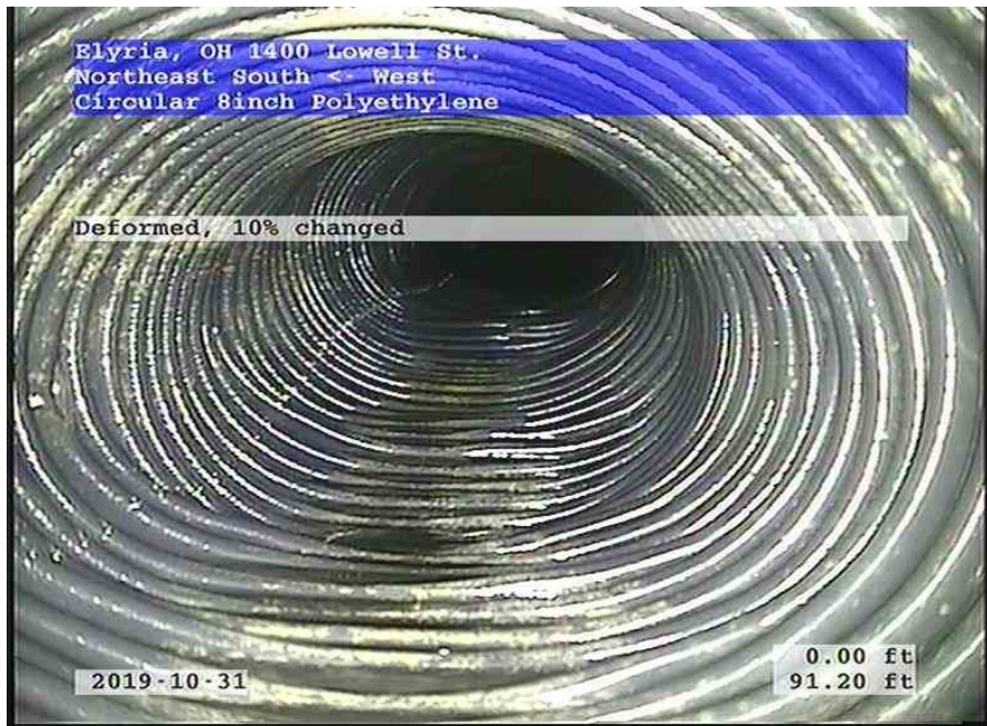
Northeast South-West_dd7d2c25-056c-4399-8c91-92227aa3ac84_20191031_113817_524.jpg, 00:06:41, 91.20ft Deformed, 10% changed
