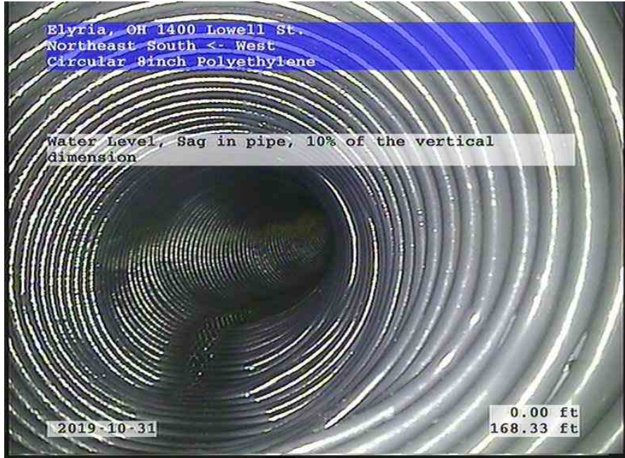
Northeast South-West_0d537fca-6a77-4f99-97fb-28a14a518e16_20191031_120305_701.jpg, 00:11:19, 168.33ft Water Level, Sag in pipe, 10% of the vertical dimension
