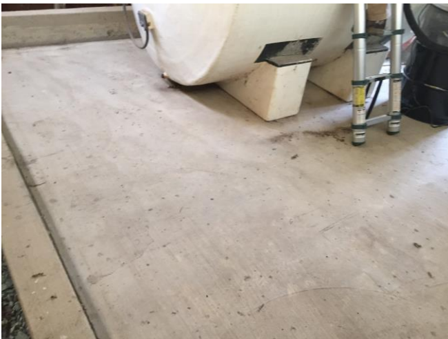
Photo #3: Concrete pad of secondary containment system
