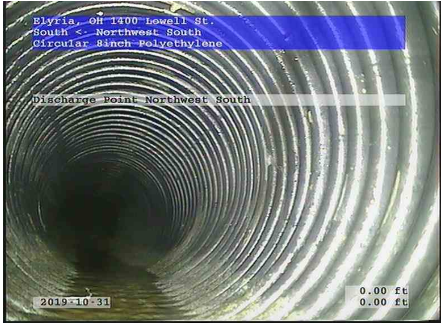
South-Northwest South_29a41f92-470a-49fc-84b0-a6887a716ff2_20191031_163045_128.jpg, 00:00:00, 0.00ft Discharge Point
