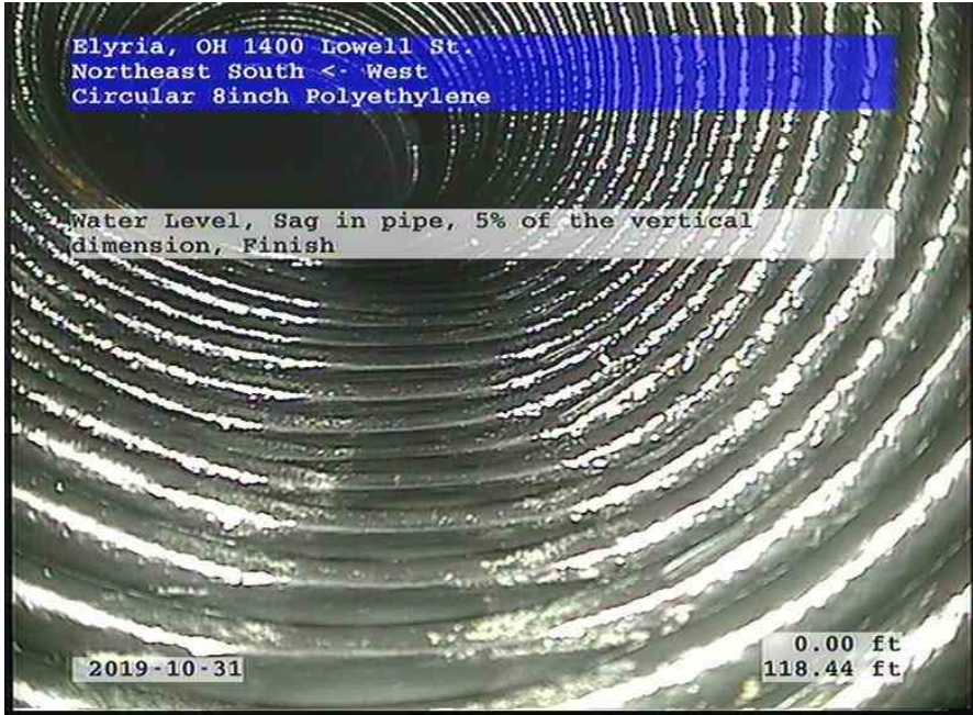
Northeast South-West_509edd4d-809f-4033-9c34-7d29da566b2a_20191031_113959_803.jpg, 00:08:12, 118.44ft Water Level, Sag in pipe, 5% of the vertical dimension, Finish
