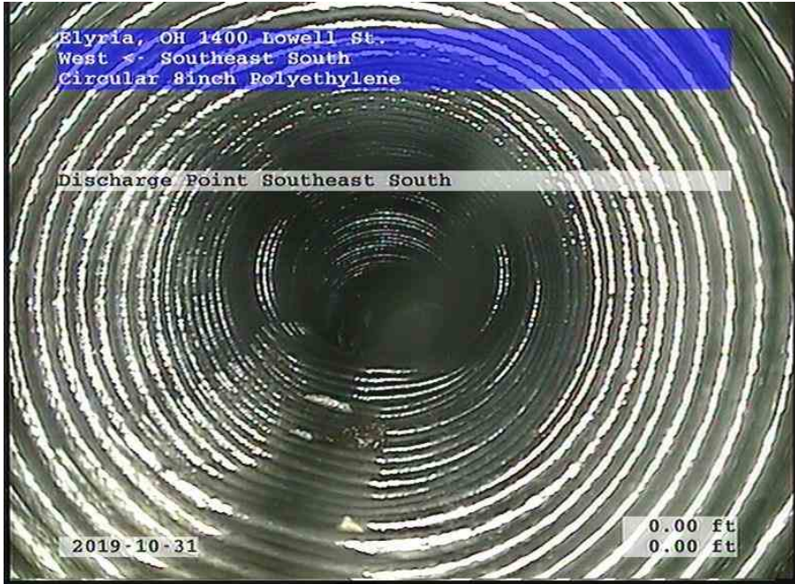
West-Southeast South_eb881e6d-939d-44af-a383-2df5479a2676_20191031_135928_110.jpg, 00:00:00, 0.00ft Discharge Point
