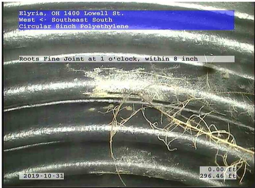
West-Southeast South_e4338f6d-811d-4af8-90f2-807dd0e63c27_20191031_141716_390.jpg, 00:13:36, 296.46ft Roots Fine Joint at 1 o'clock, within 8 inch
