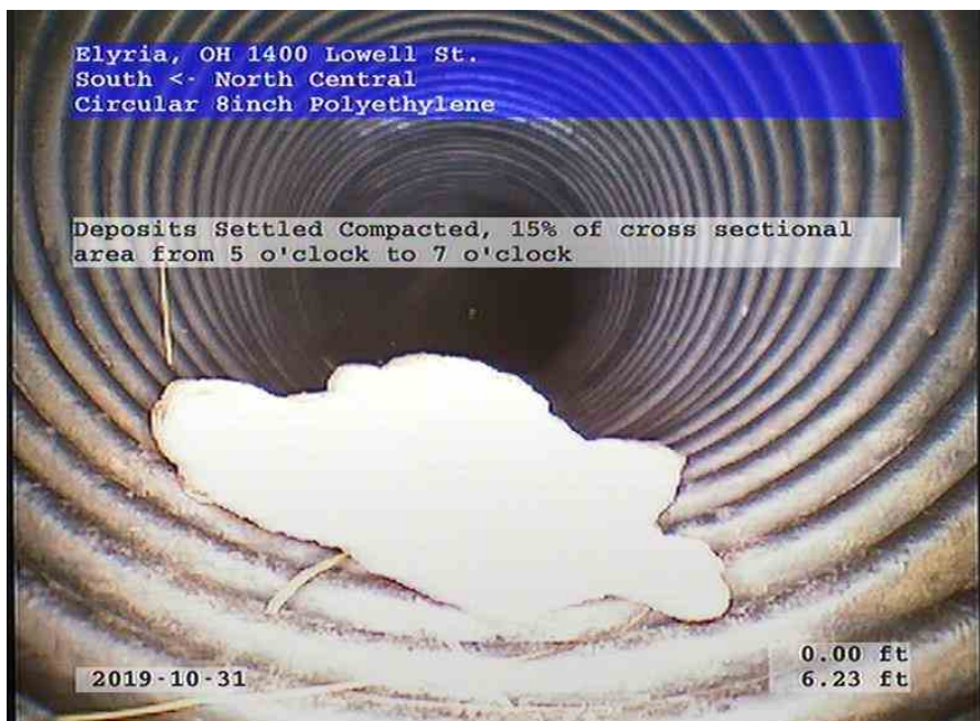
South-North Central_f308c9af-d8ca-474b-aba3-ebc824385c99_20191031_084411_735.jpg, 00:01:02, 6.23ft Deposits Settled Compacted, 15% of cross sectional area from 5 o'clock to 7 o'clock
