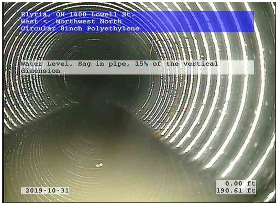
West-Northwest North_ca734e12-2f34-4ed3-a41a-3430a3983c3d_20191031_165127_672.jpg, 00:05:54, 190.61ft Water Level, Sag in pipe, 15% of the vertical dimension
