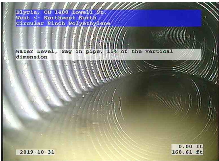
West-Northwest North_f02b48c5-eb0e-464b-b8e1-710315b35063_20191031_165051_248.jpg, 00:05:24, 168.61ft Water Level, Sag in pipe, 15% of the vertical dimension
