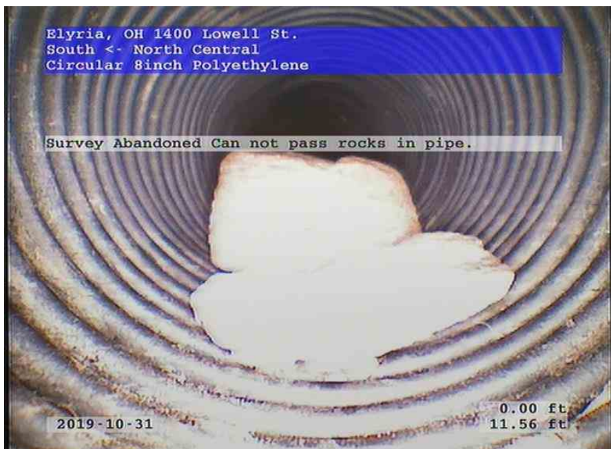
South-North Central_f0f16c76-02e4-473b-9105-7029c37c4d01_20191031_084656_395.jpg, 00:02:32, 11.56ft Survey Abandoned
