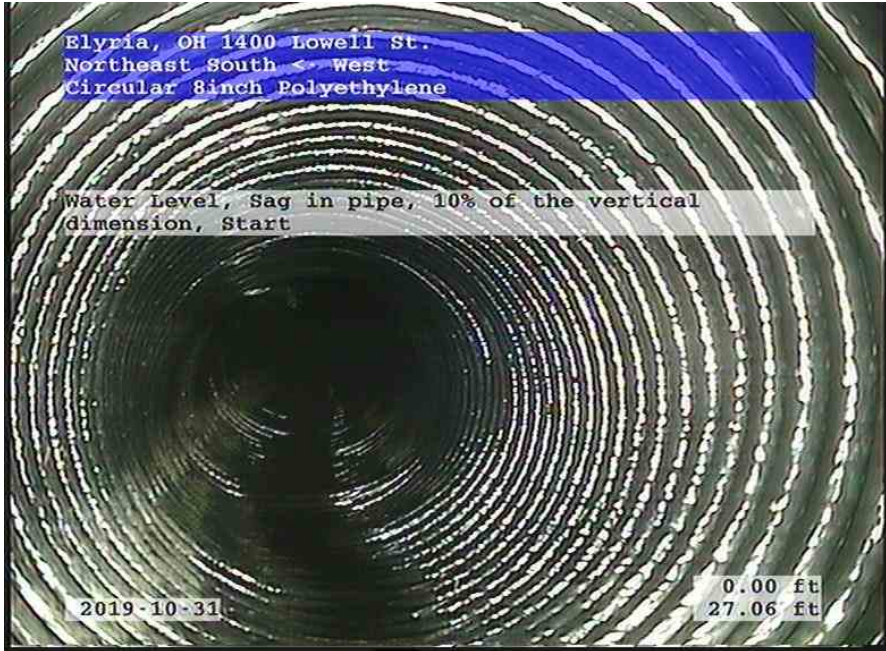
Northeast South-West_e304673e-9e59-473b-b8bb-c309b0a34e4b_20191031_113052_767.jpg, 00:01:53, 27.06ft Water Level, Sag in pipe, 10% of the vertical dimension, Start
