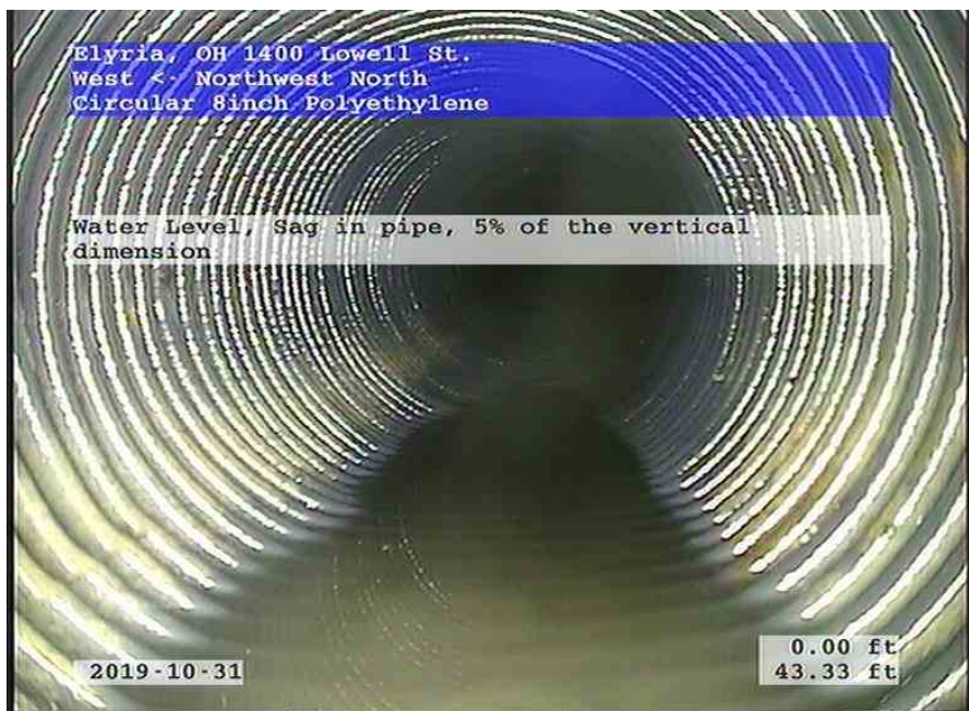
West-Northwest North_fb35bbfa-4ef4-4e11-8a5c-fd901d9f234b_20191031_164703_919.jpg, 00:01:51, 43.33ft Water Level, Sag in pipe, 5% of the vertical dimension
