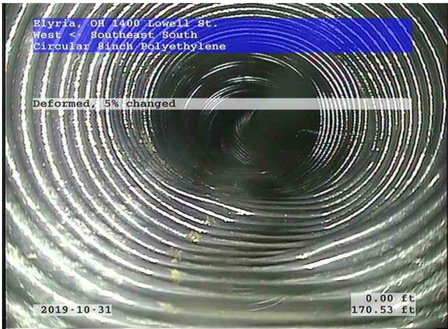
West-Southeast South_71c2953e-9455-4af4-8cbe-fc0991096e07_20191031_140830_860.jpg, 00:06:40, 170.53ft Deformed, 5% changed
