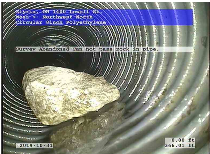
West-Northwest North_87471a83-3fa7-413f-9d93-bca947bb9266_20191031_170526_753.jpg, 00:19:19, 366.01ft Survey Abandoned
