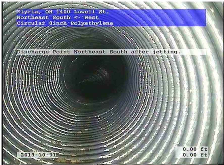
Northeast South-West_7ff63e6d-4ada-4def-a0c8-998b8147ff0e_20191031_112836_015.jpg, 00:00:00, 0.00ft Discharge Point
