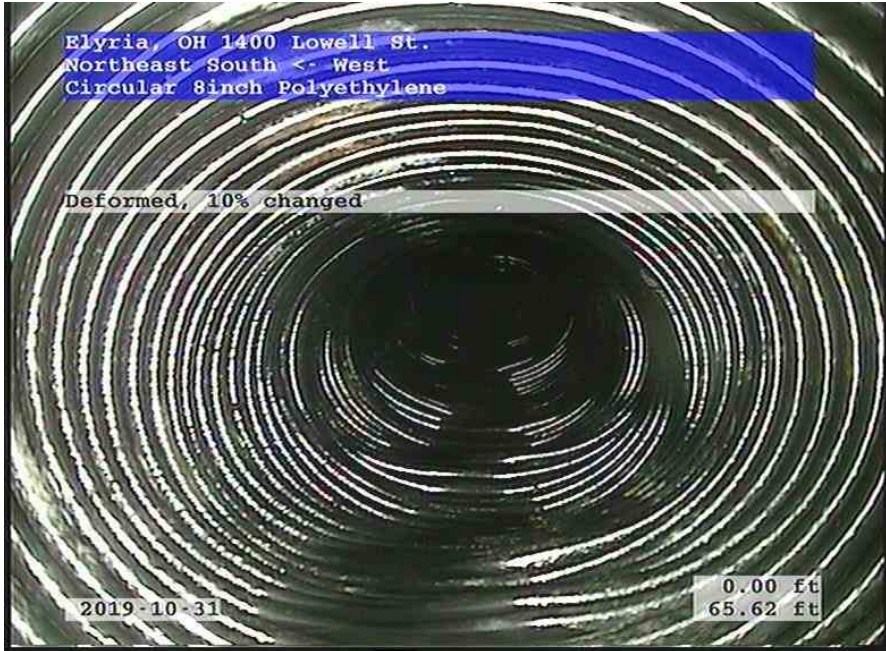
Northeast South-West_aa356f1d-fcf7-4984-8772-1995aa87e02d_20191031_113643_578.jpg, 00:05:25, 65.62ft Deformed, 10% changed
