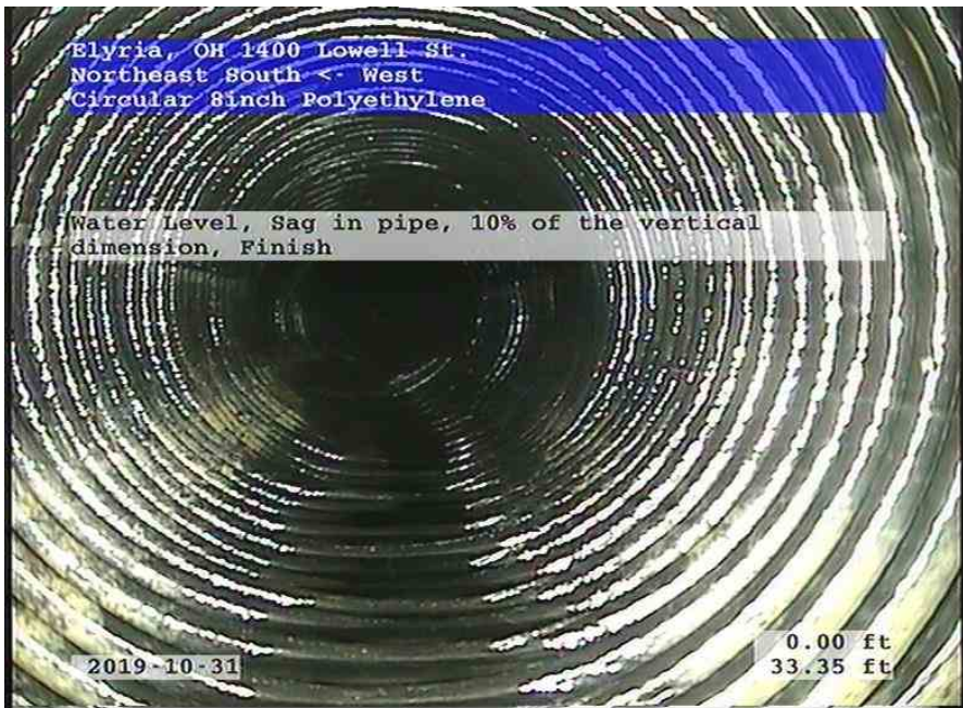
Northeast South-West_2e4c4a35-28a4-4f6f-bd51-1c9a6e7f14ea_20191031_113112_308.jpg, 00:02:10, 33.35ft Water Level, Sag in pipe, 10% of the vertical dimension, Finish
