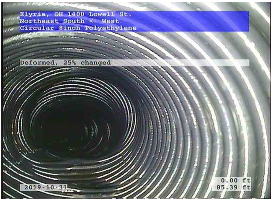
Northeast South-West_2db5c6e7-97ec-4ee7-af13-d6e21f47bca3_20191031_113749_102.jpg, 00:06:19, 85.39ft Deformed, 25% changed
