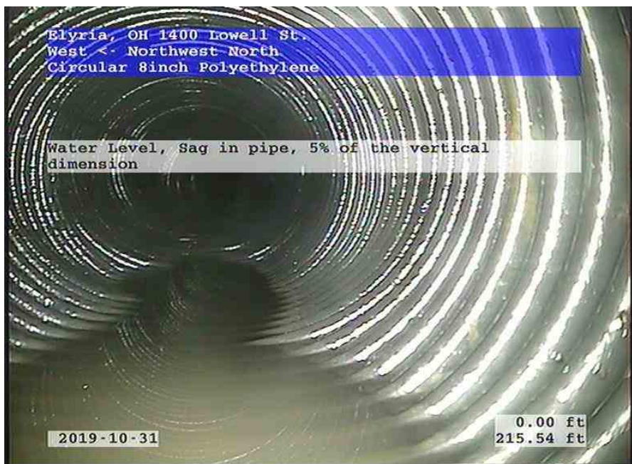
West-Northwest North_c74a3a49-e418-4e00-b0e2-92986ead7913_20191031_165209_892.jpg, 00:06:31, 215.54ft Water Level, Sag in pipe, 5% of the vertical dimension
