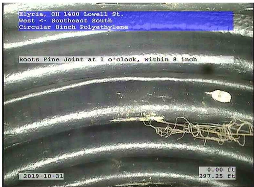
West-Southeast South_f8e9557f-df8f-4bc6-9183-5d22718265db_20191031_141747_650.jpg, 00:13:56, 297.25ft Roots Fine Joint at 1 o'clock, within 8 inch
