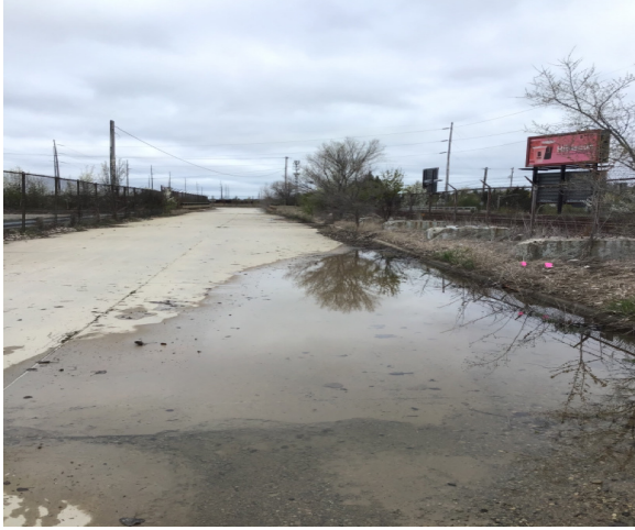
Ponding at P2-MH-13 and P2-MH-12 has decreased since yesterday.
