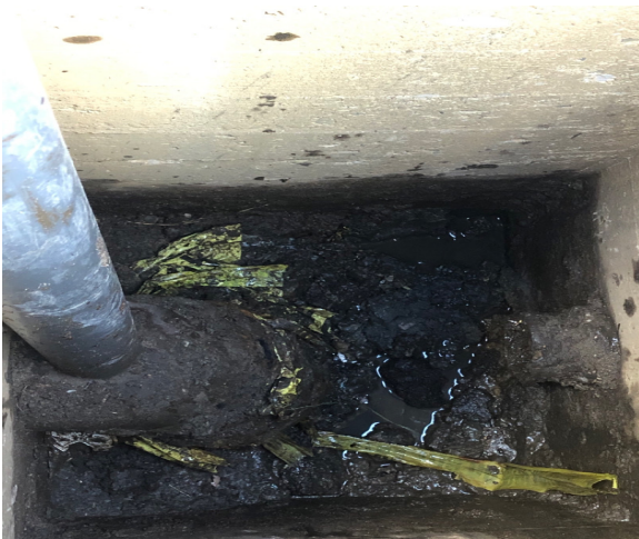
P2-CB-7 cleaned out with 90° pipe exposed
