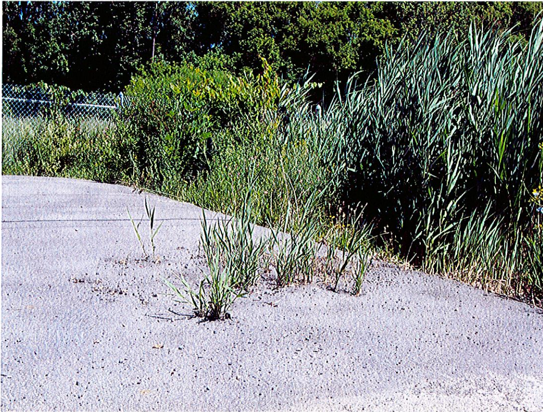
Photograph 15: View of phragmites in pavement access drive.
