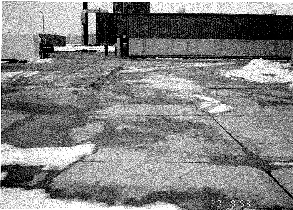
Photograph No. 4 Orientation: East Description: This photograph shows the HWSA, including the central drainage trench.
