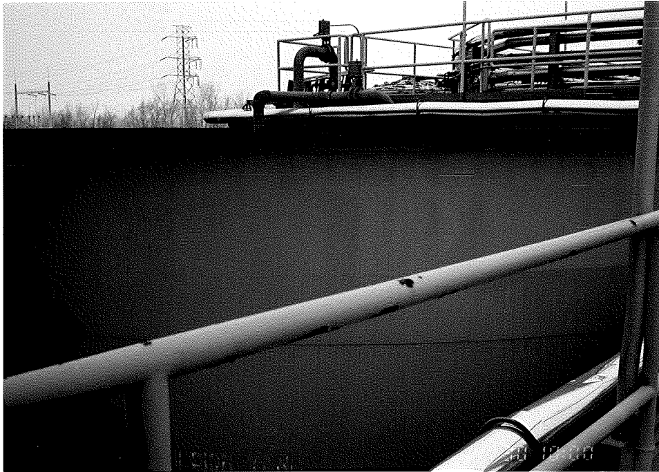
Photograph No. 5 Orientation: North Description: This photograph shows an emulsion AST at the WTP.
