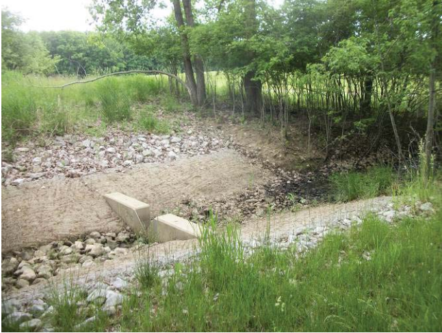
Photo 13: Storm water management weir on the western side of property in wetland B2.
