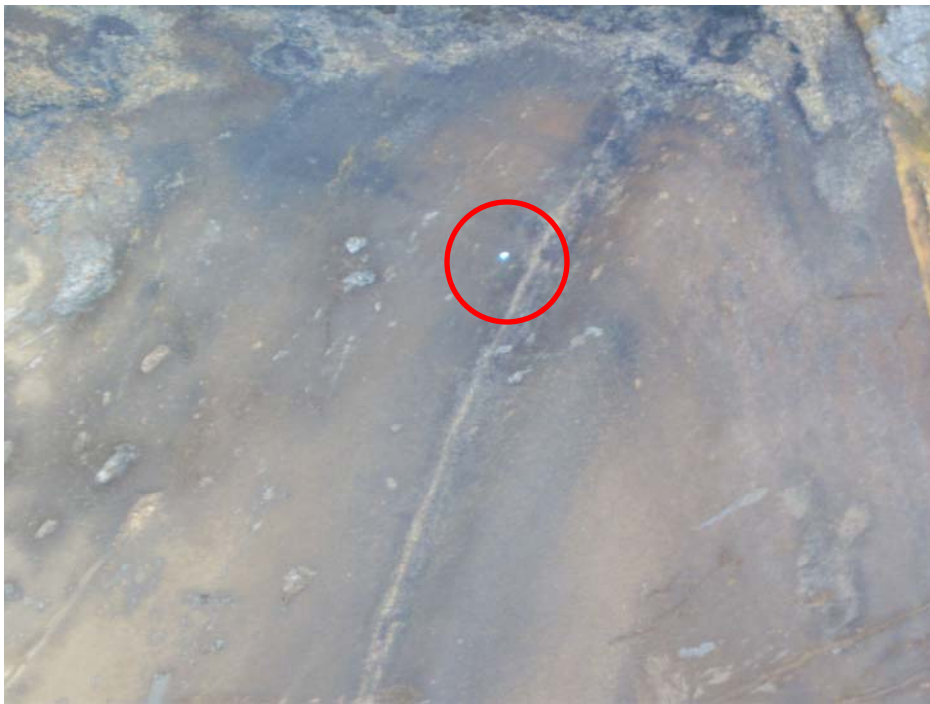
Holiday noted within circle (close-up view)
