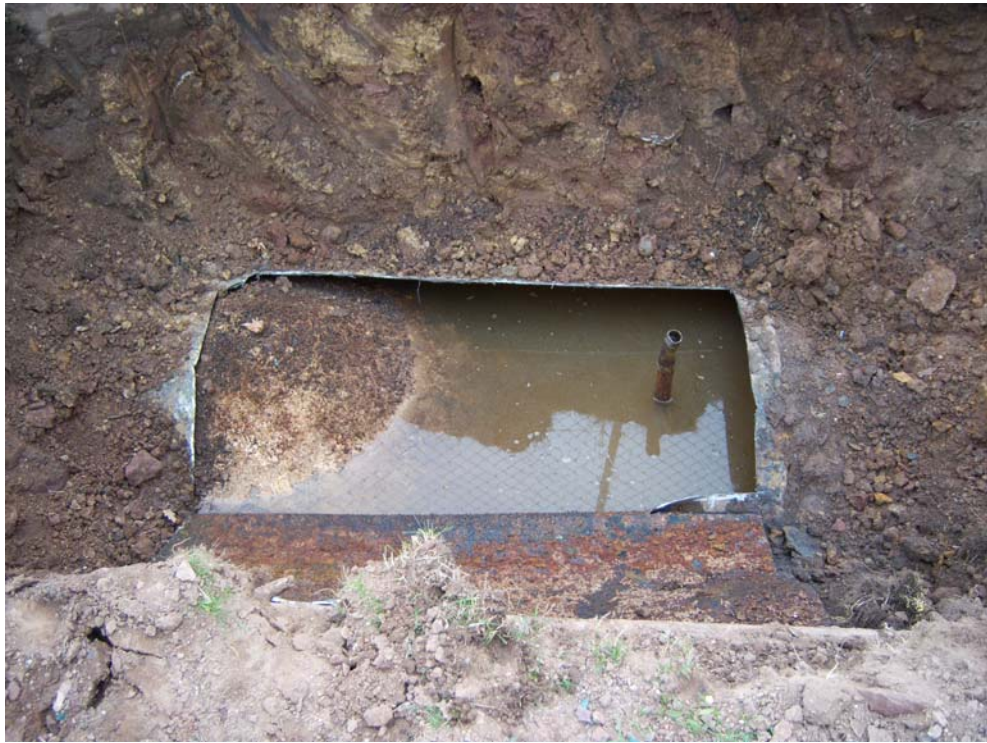
Prior to pumping
