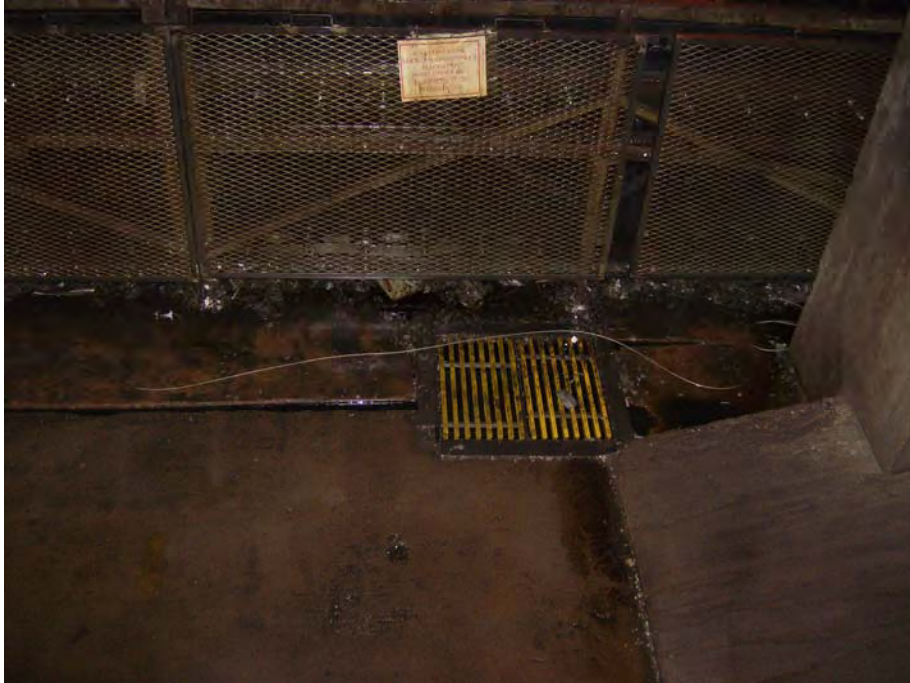
Photo 17: Oily trenches and sump along basement conveyor (typical)
