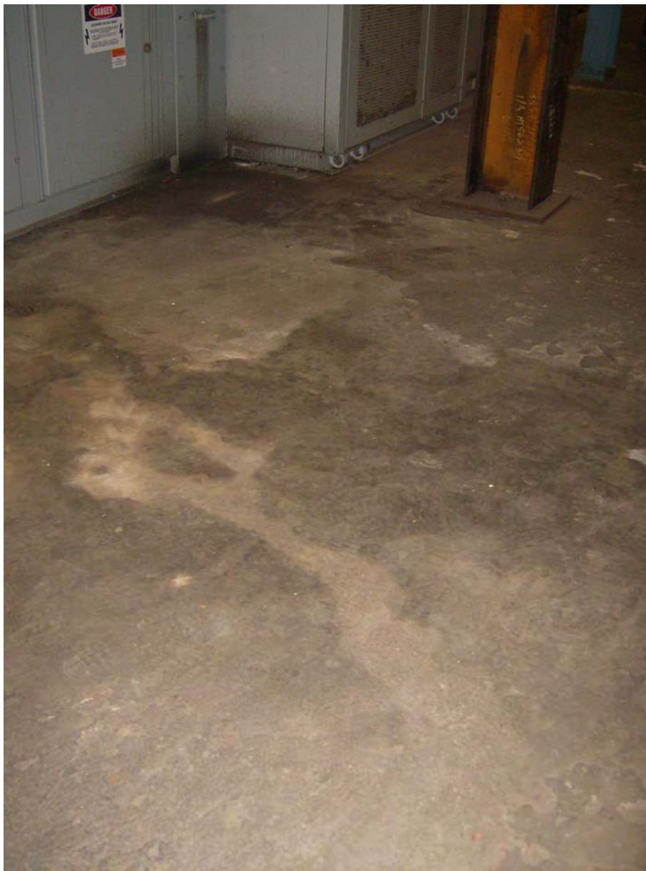
Photo 39: Staining in Substation K in basement
