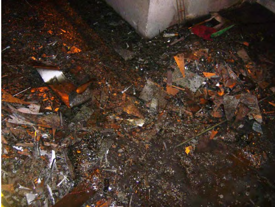
Photo 13: Scrap metal in basement conveyor area
