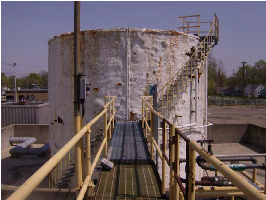
Photo 20: Used oil AST at WWTP
