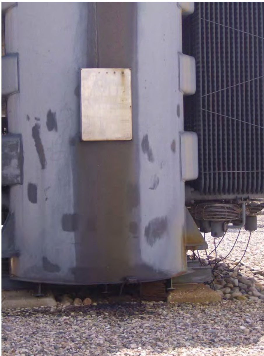
Photo 42: Staining near Consumers transformer
