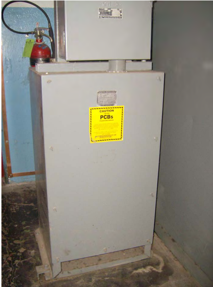
Photo 40: PCB-electrical equipment in Substations B and C
