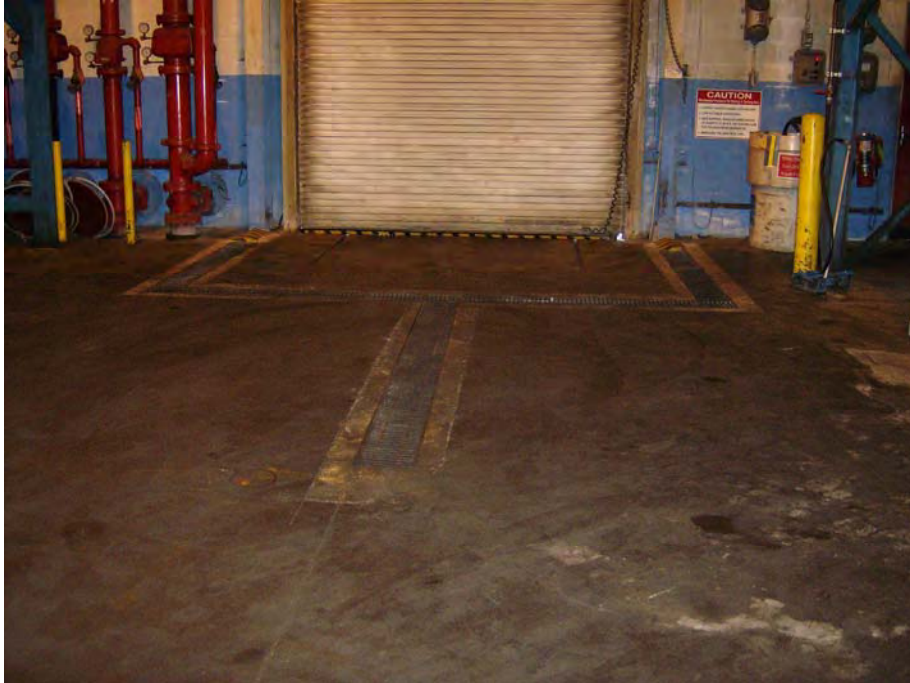
Photo 27: Trench drain in chemical storage area of Oil Stores
