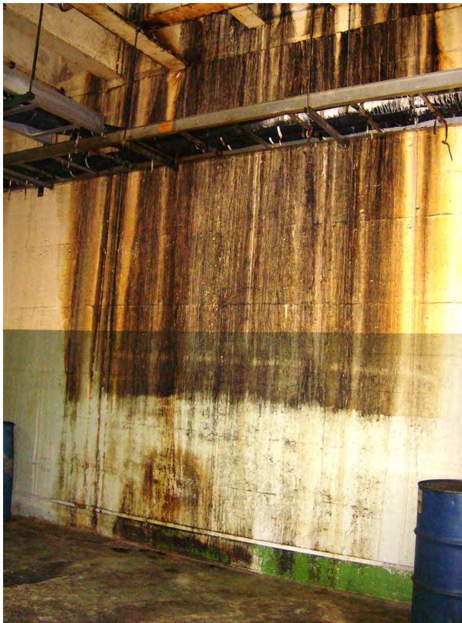
Photo 43: Oil staining on wall of basement
