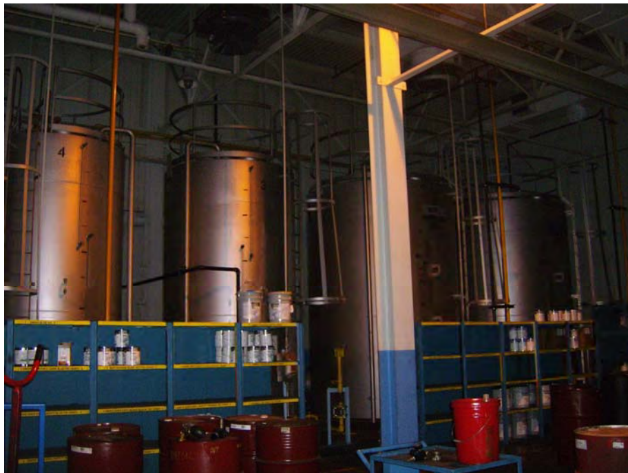
Photo 34: ASTs in Oil Stores
