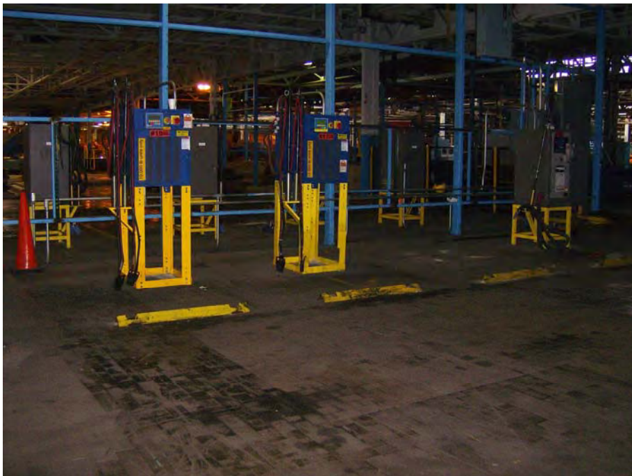
Photo 32: Battery charging area
