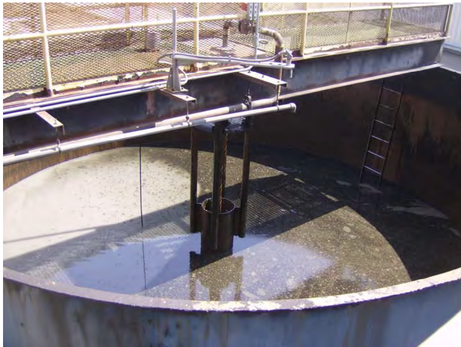
Photo 16: WWTP batch tank
