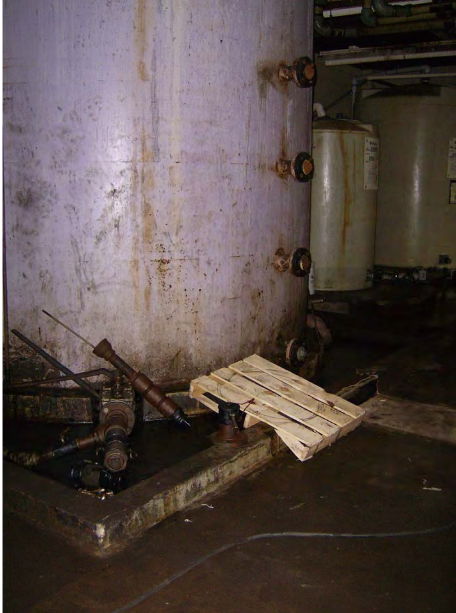
Photo 44: Staining near ASTs in WWTP
