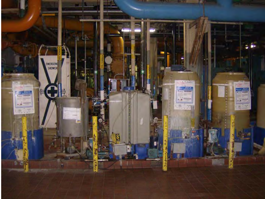
Photo 3: Boiler treatment chemicals in Power House
