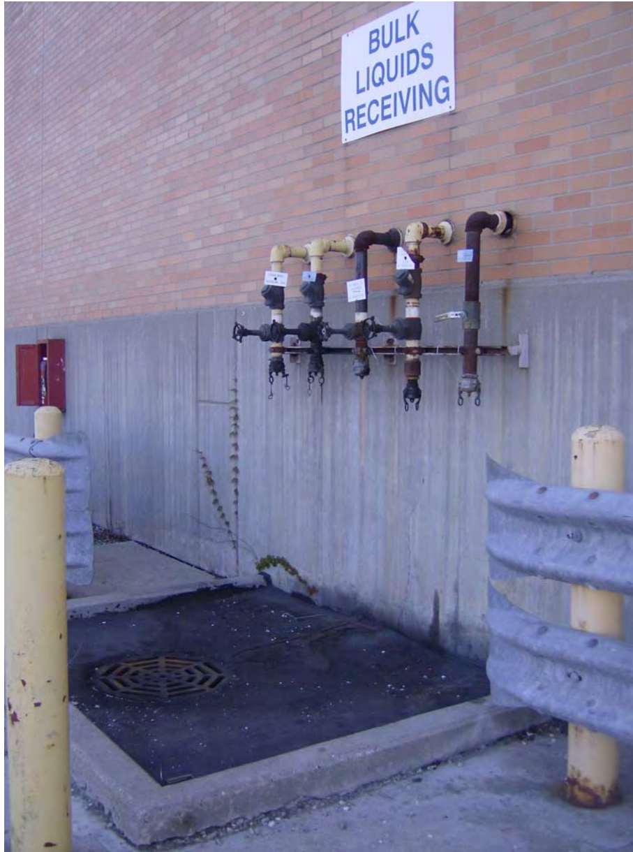
Photo 37: Bulk unload area sump
