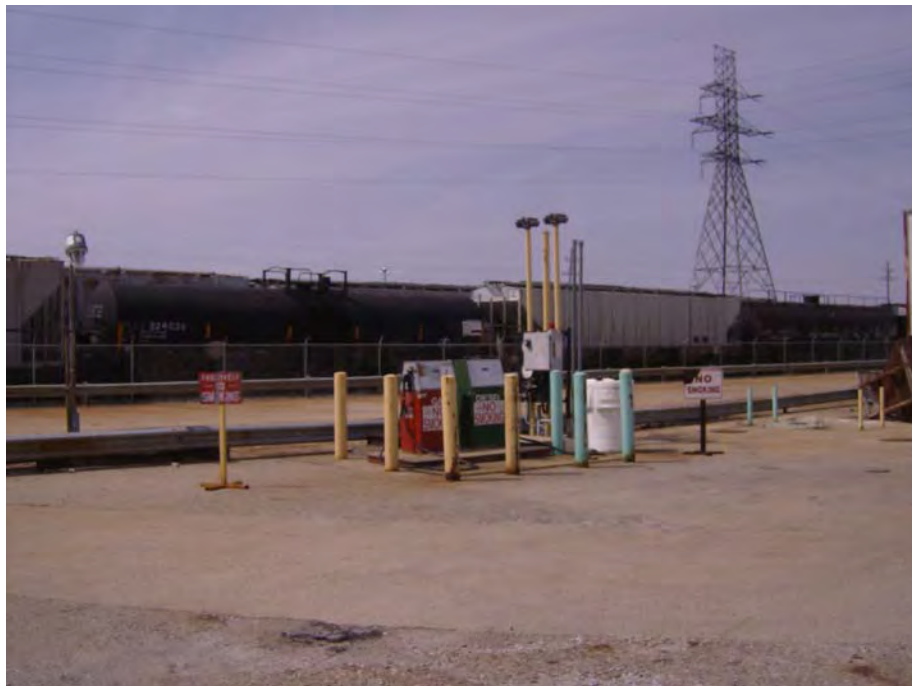
Photo 51: Current UST dispensers
