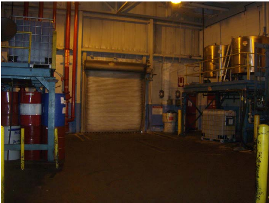
Photo 22: Chemical storage in Oil Stores
