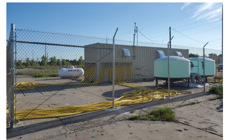
Plant 2 Biosparge Unit and Nutrient Injection Tanks
