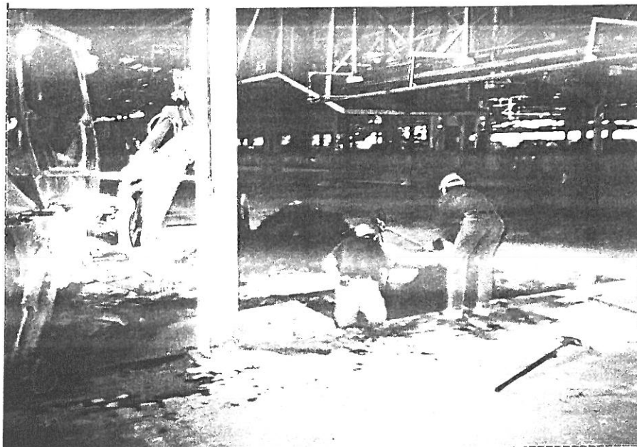
PHOTO 15 - WORKERS ATTEMPTING TO LOCATE KEROSENE PIPE WEST OF THE ESP
