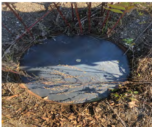
circular catch basin covered with lid
