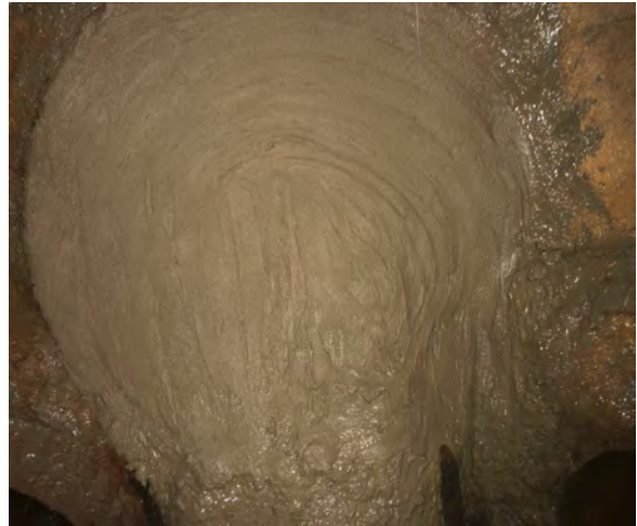
Plugged southwestern pipe Osborn-MH-1 coming from P6-MH-11 that was trickling
