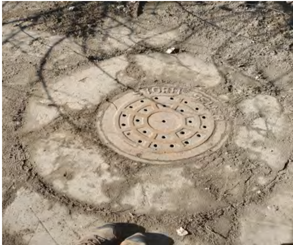
uncovered catch basin lid
