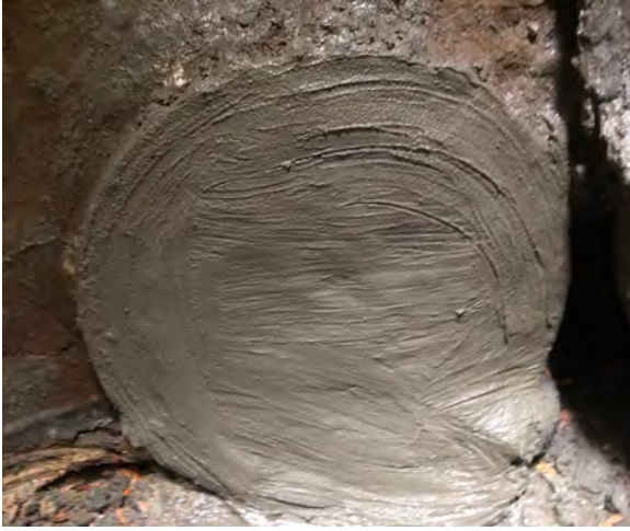
Southern pipe plug Osborn-MH-1
