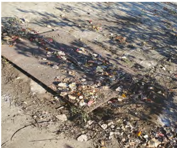
uncovered catch basin lid, steel plate covering because missing lid
