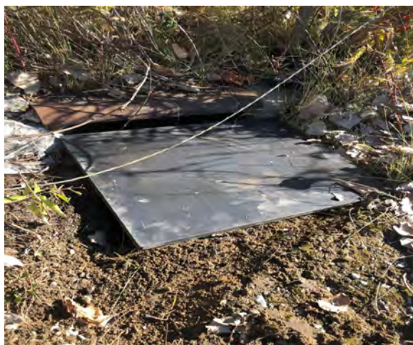
rectangular catch basin covered with lid
