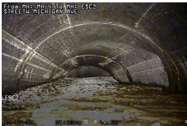
Photograph 18: Inspection of ESC-2 fill from downstream indicated impartial fill and infiltration
