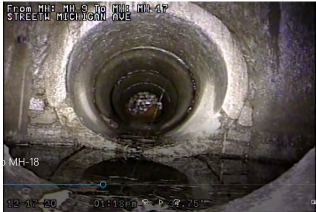
Photograph 16: Blocked pipe called "cut and cap" in 2014 documents located upstream of plant boundary
