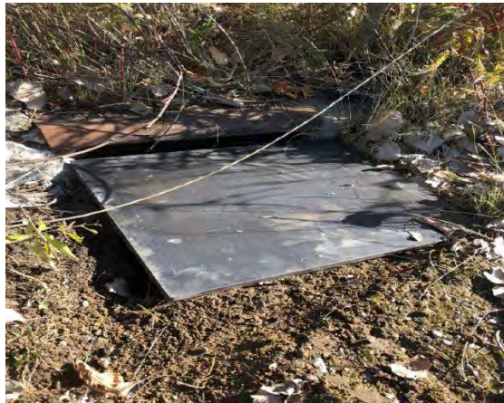
Photograph 4: Lid placed on rectangular catch basin that was missing its lid
