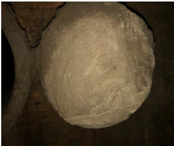
Plugged western HDPE pipe Osborn-MH-1
