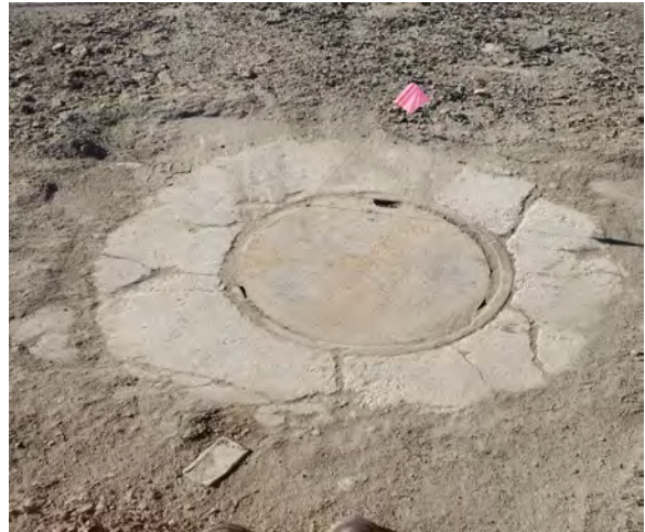
uncovered catch basin lid
