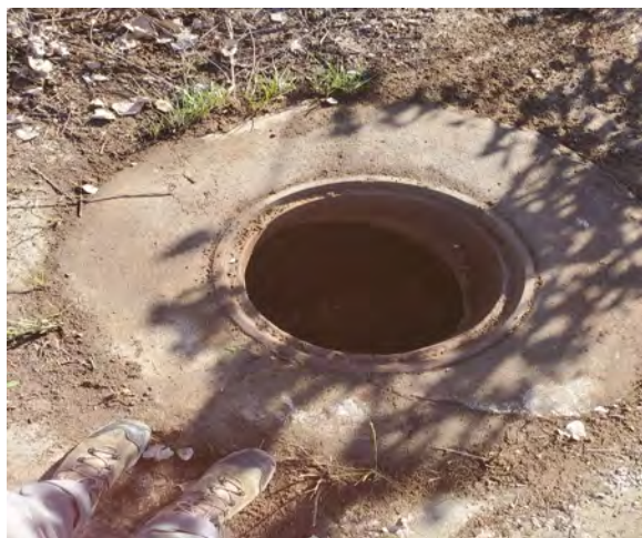
no lid under steel plate, 23.25 diameter
