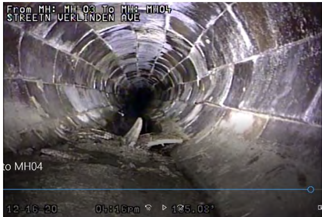
Photograph 14: Fallen piece of pipe blocking CCTV path
