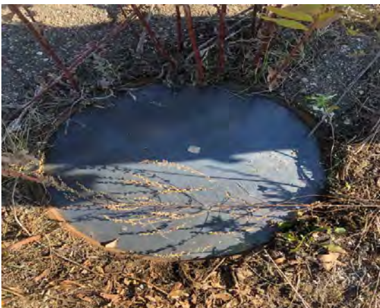
Photograph 5: Lid placed on circular catch basin that was missing its lid
