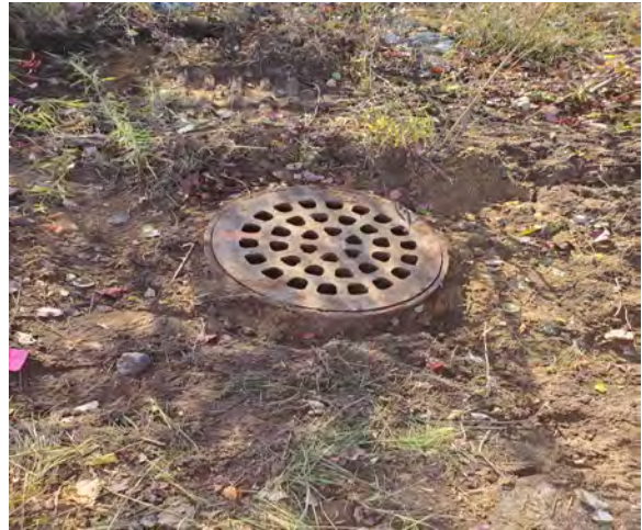
uncovered catch basin lid
