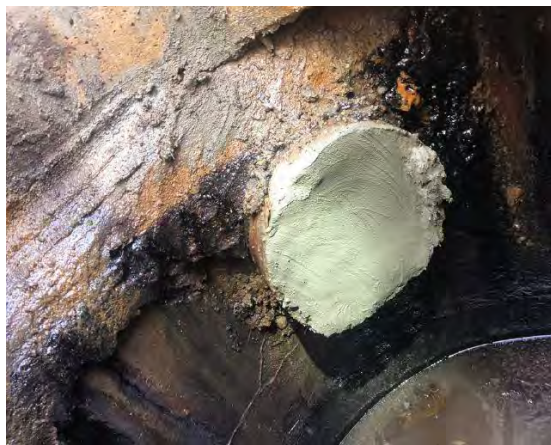
Photograph 6: Typical plugged pipe in Osborn-MH-1
