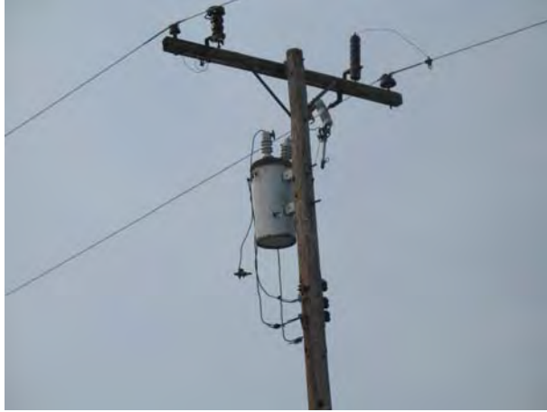
Photograph 10. View of a pole-mounted transformer located in the southeastern portion of the Site.
