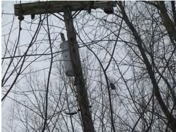
Photograph 11. View of a pole-mounted transformer located in the eastern portion of the Site.
