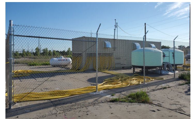
Plant 2 Biosparge Unit and Nutrient Injection Tanks
