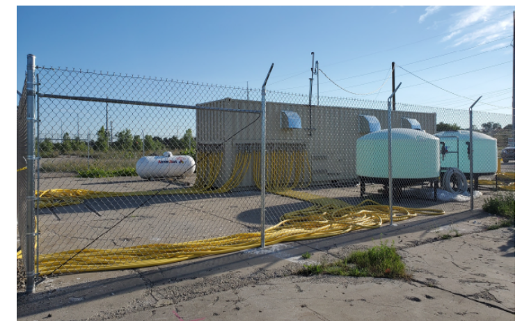
Plant 2 Biosparge Building, Propane Tank, Hoses, and Nutrient Injection Tanks
