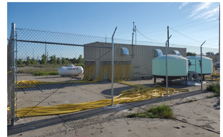
Plant 2 Biosparge Unit and Nutrient Injection Tanks
