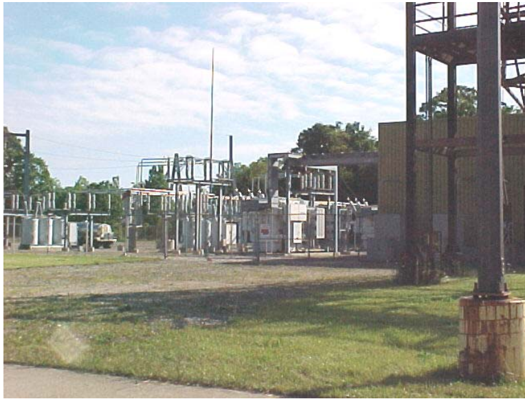
Photograph 13: Electrical substation and building (#560).
