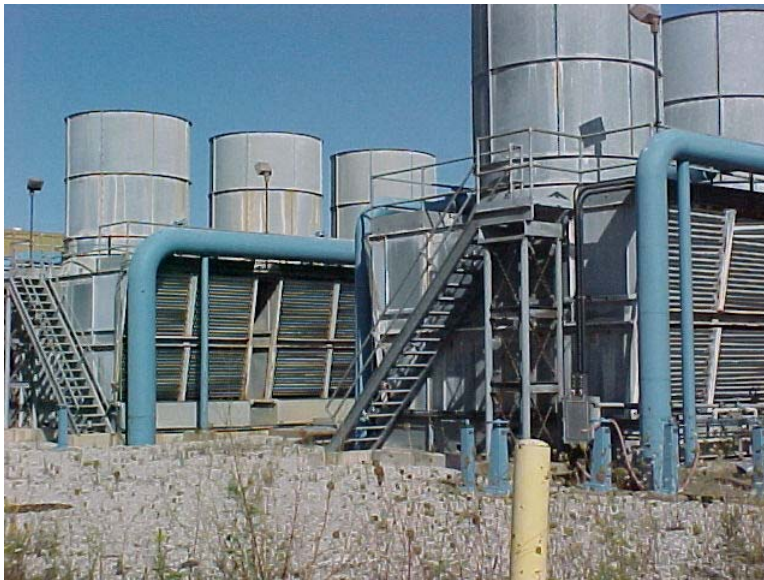
Photograph 16: Compressor cooling towers.
