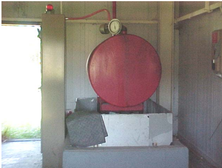
Photograph 20: Diesel storage tank in Building 568.
