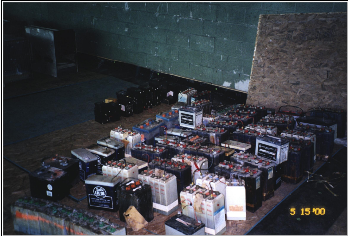
PHOTO #5 COLLECTION OF BATTERIES
