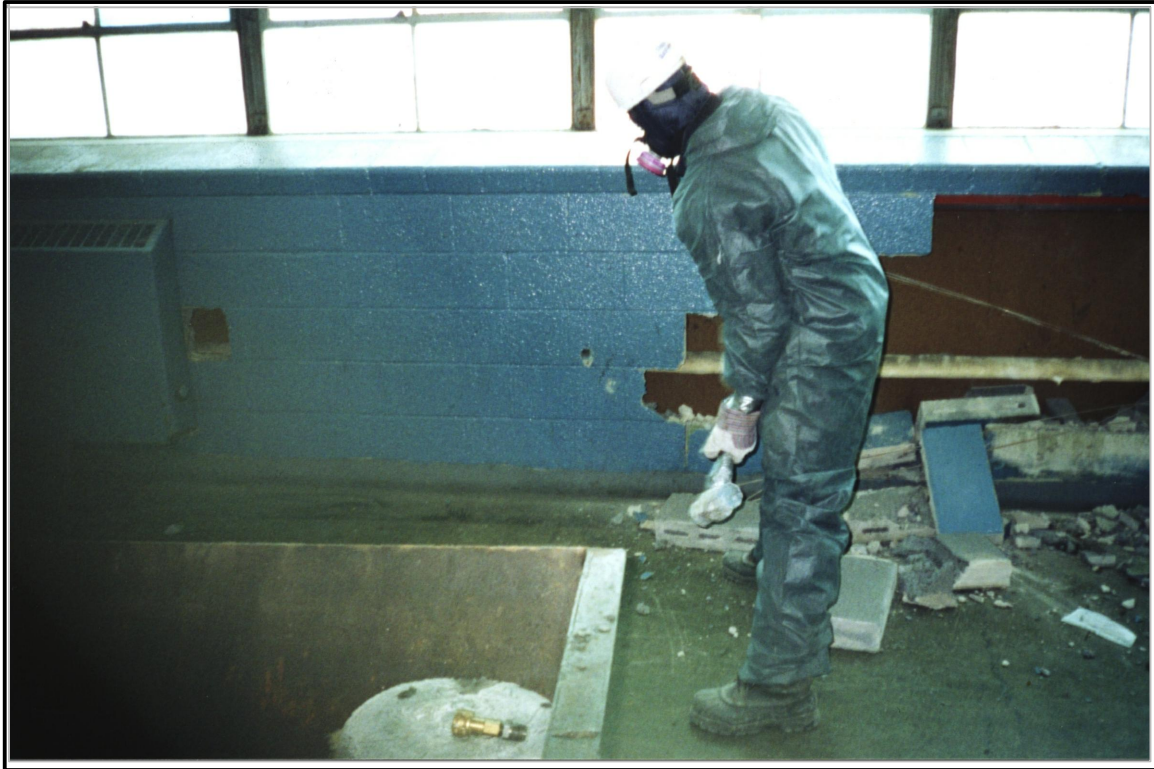
PHOTO #3 EXPOSING ASBESTOS PIPING
