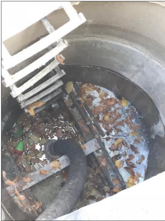
8: The concrete bulkhead sets in P3-MH-1-7. Also pictured is the bypass pump hose that would pump infiltrating water out of the sump
