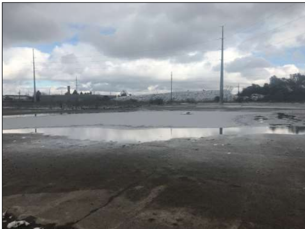
5: Ponding noted near the northeastern fence on November 13, 2018. A capped catch basin can be seen in the middle of the standing water
