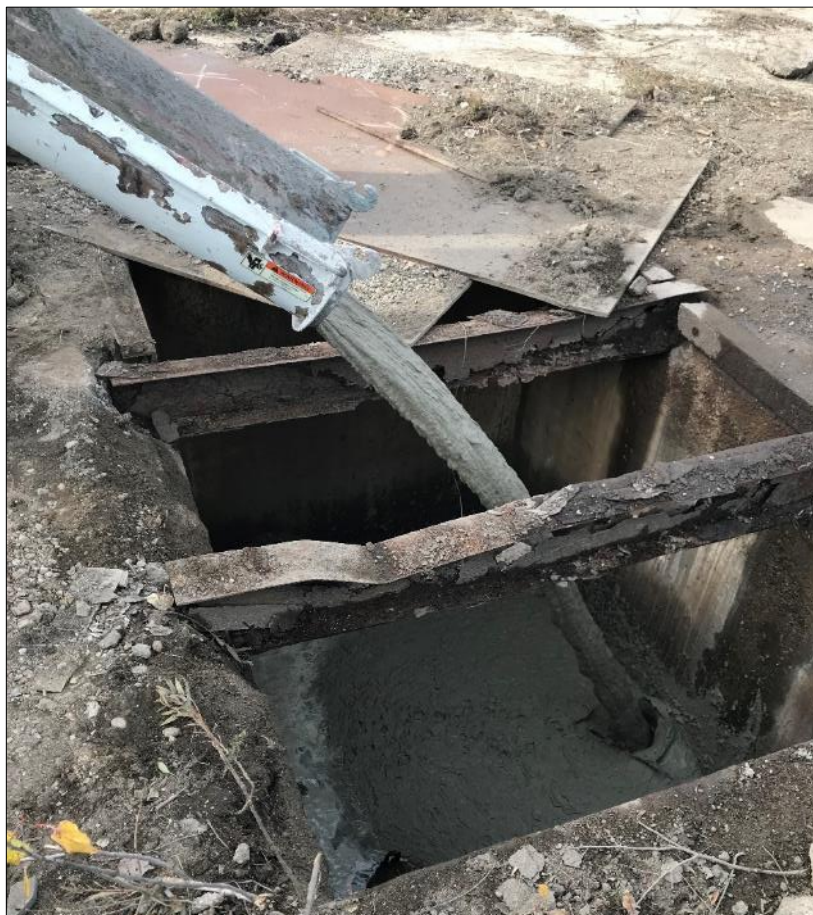
29: The oil-water separator (OWS) was pumped out and filled with CLSM to mitigate runoff into the decommissioned eastern storm main.
