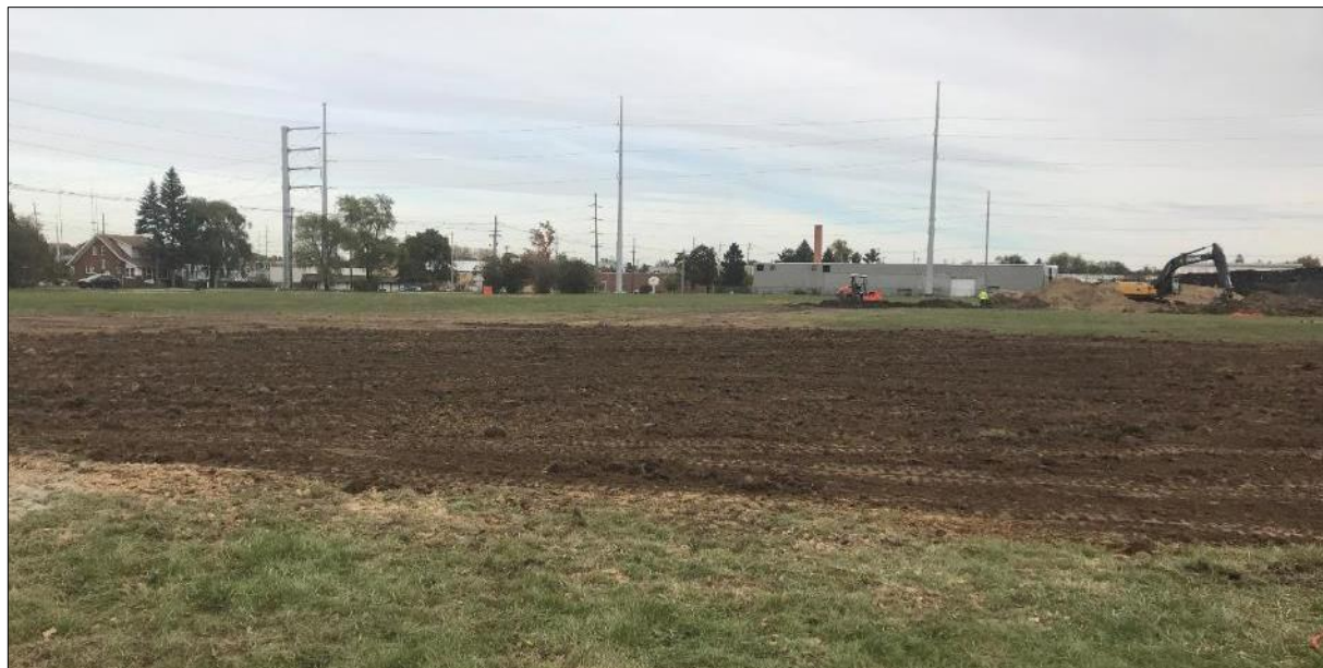
27: Western excavation area after backfilling was complete. The original topsoil was used for restoration.
