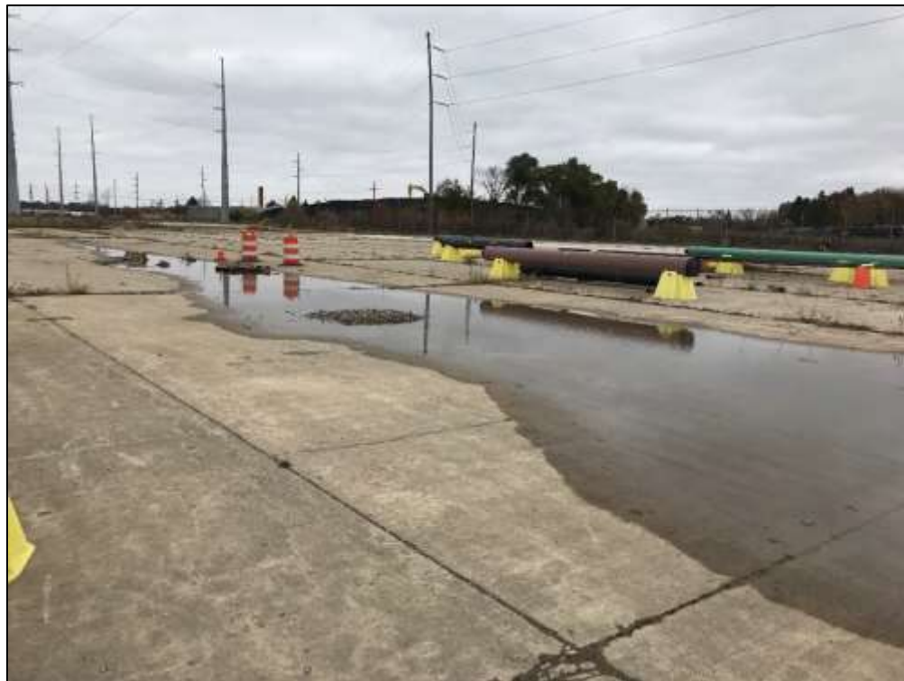
4: Ponding noted near the northeastern fence on November 7, 2018. Relief of the concrete prevents flow off site.
