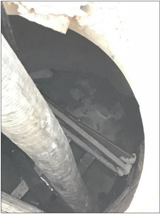
7: The freshly poured bulkhead sets in P3-MH-1-10. Also pictured is the bypass pump hose that would pump infiltrating water out of the sump
