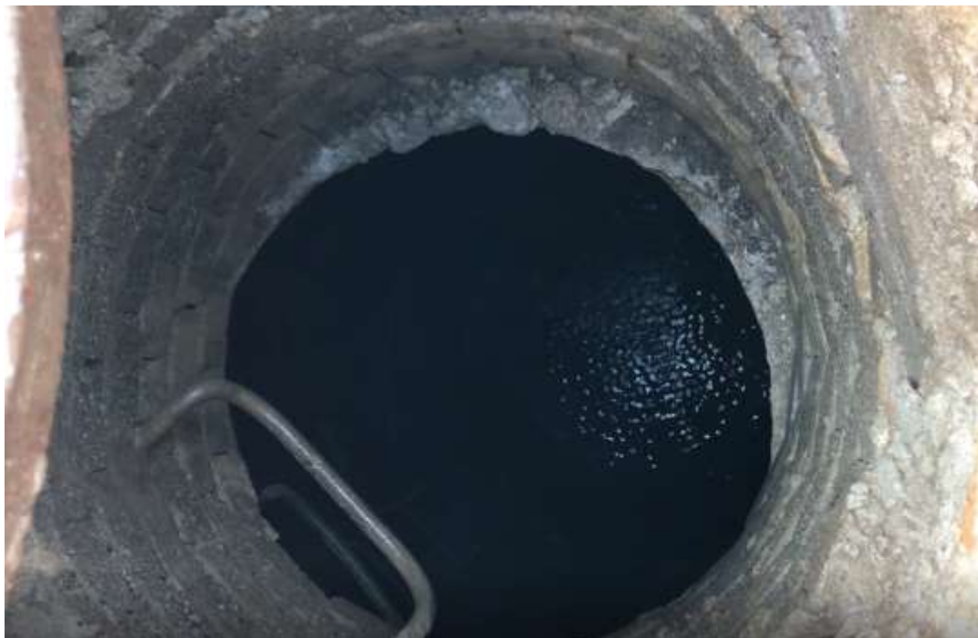
9: Property outfall manhole P3-MH-NE with water accumulation in the sump
