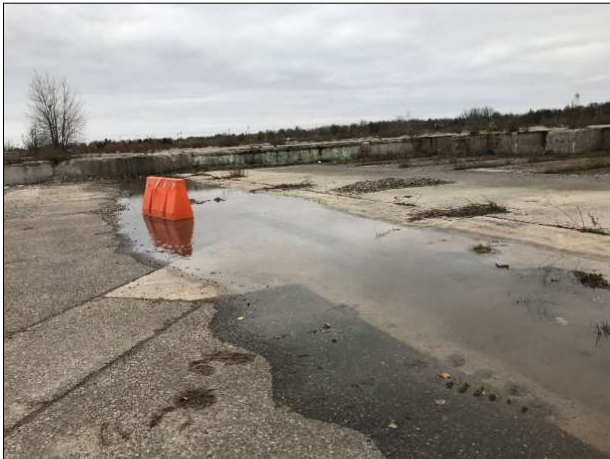
1: Minor ponding present near the plugged floor drain on November 7, 2018
