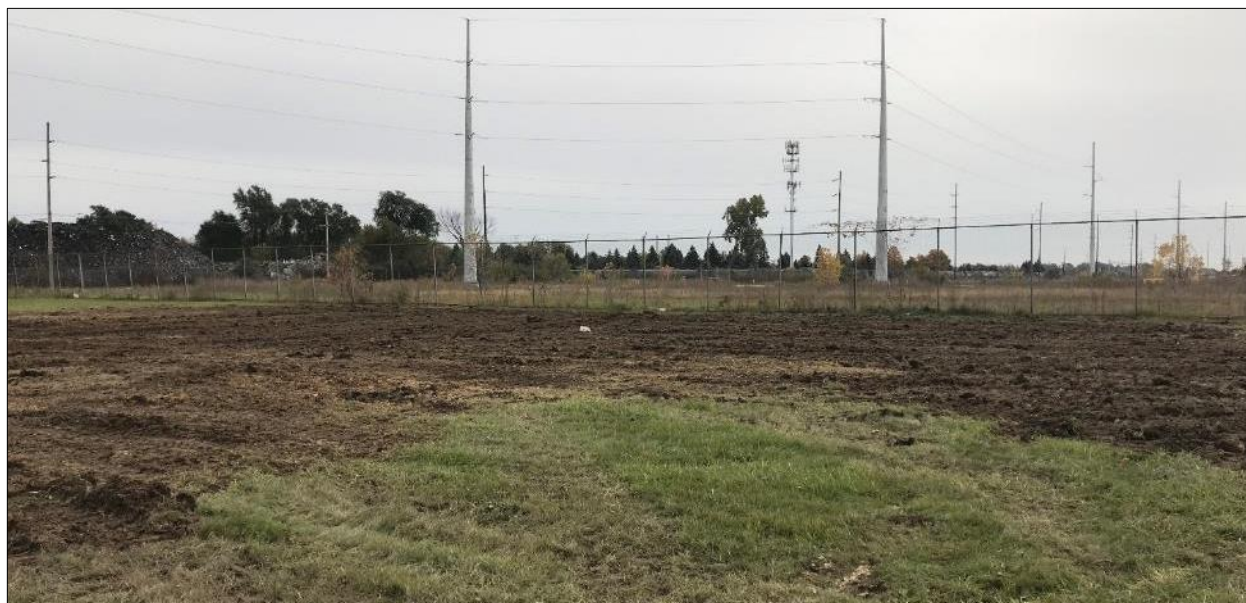
28: Eastern excavation area after backfilling was complete. The original topsoil was used for restoration.
