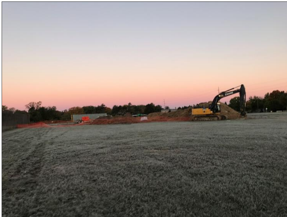
15: Wide view of the western excavation. A snow fence was placed around the excavation to secure it.
