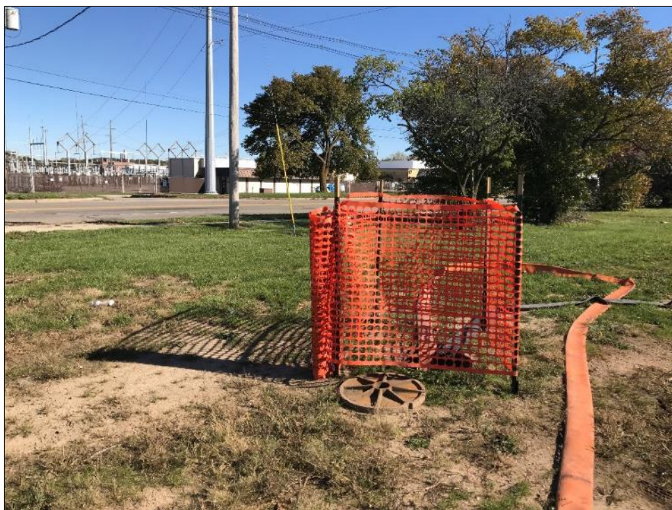
16: Stormwater upgradient of the work areas was bypass-pumped into the property outfall manhole while the pipes were prepared for monolith installation.
