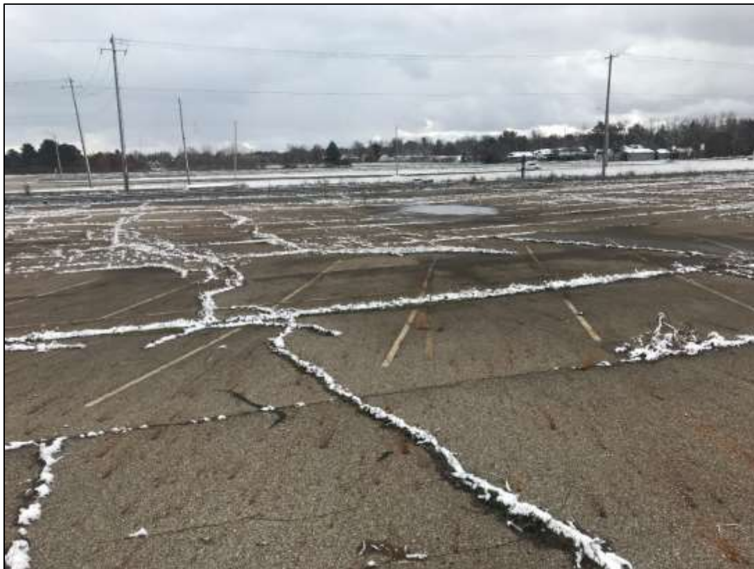
8: Minor ponding noted in southern parking lot area. No runoff noted to Saginaw Street.
