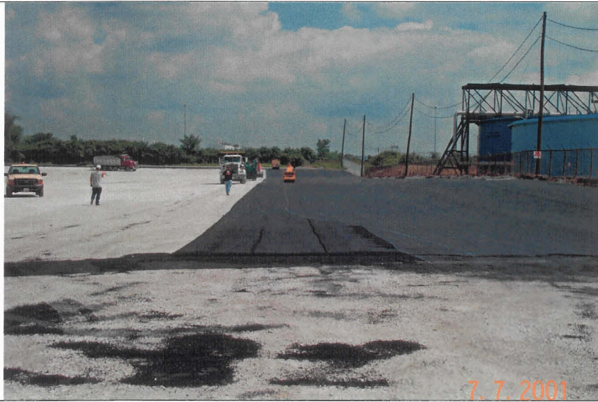
Photograph No. 44 Installing Cover - North Lagoon Placement of initial lift of asphalt pavement on prepared sub base. Looking north along east side.
