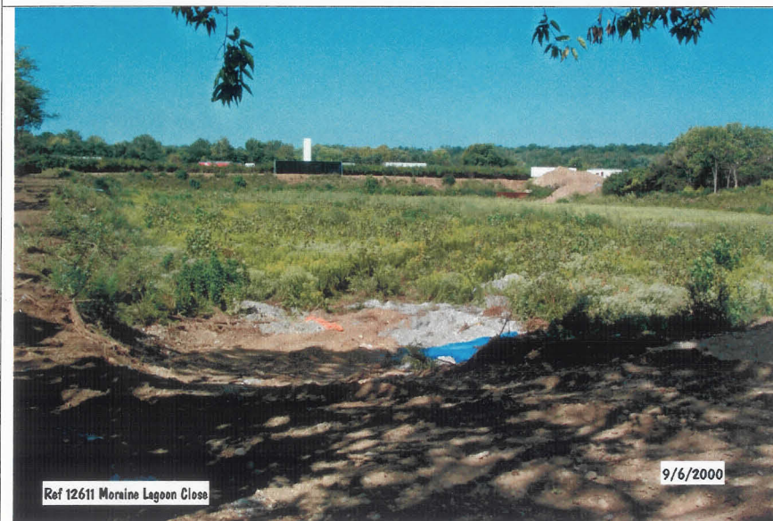
Photograph No. 2 Initial Site Conditions - South Lagoon - Secondary Basin Looking northwest prior to grubbing.
