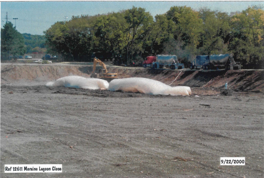
Photograph No. 15 Solidifying Sludge - South Lagoon - Secondary Basin Unloading CKD into visqueen pockets. Looking southeast from west bank.
