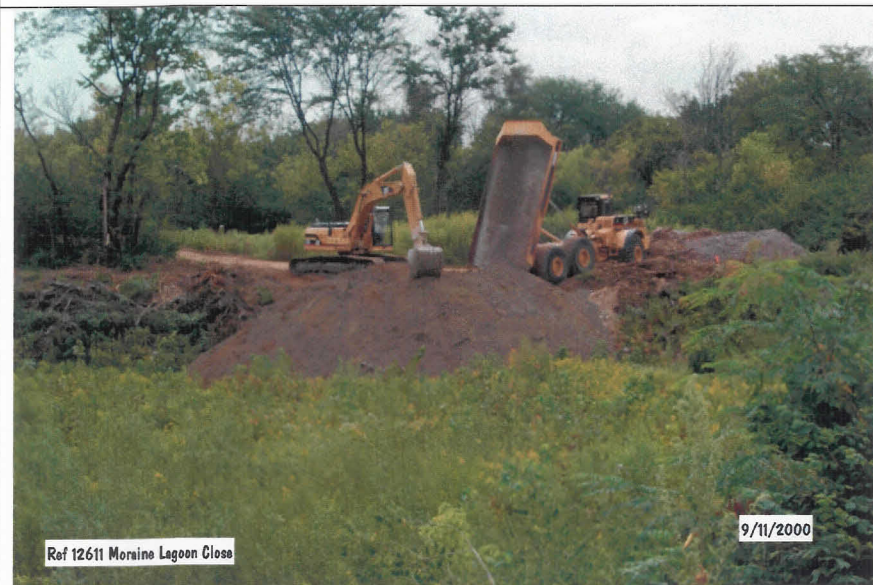
Photograph No. 8 Sludge Transfer - South Lagoon - Secondary Basin.
