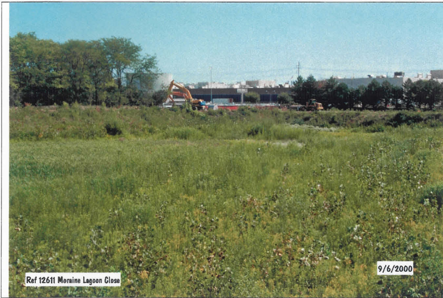
Photograph No. 1 Initial Site Conditions - South Lagoon - Secondary Basin Looking northeast prior to grubbing.
