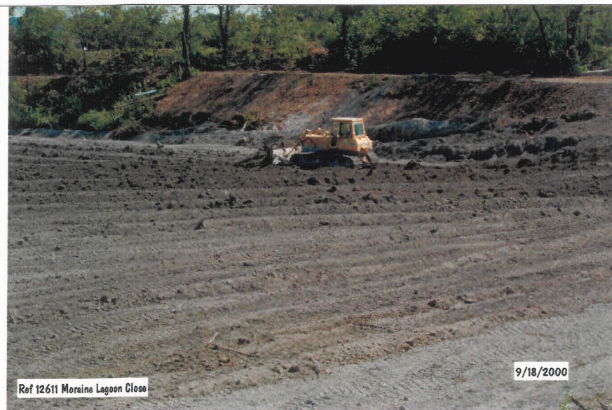
Photograph No. 9 Sludge Transfer - South Lagoon - Secondary Basin
