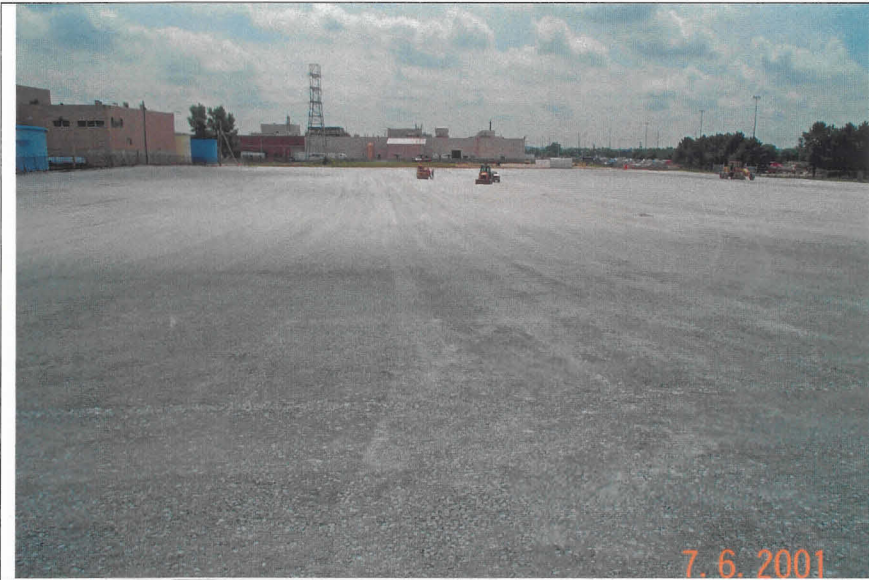
Photograph No. 43 Installing Cover - North Lagoon Prepared sub base prior to installation of asphalt. Looking south from north end.
