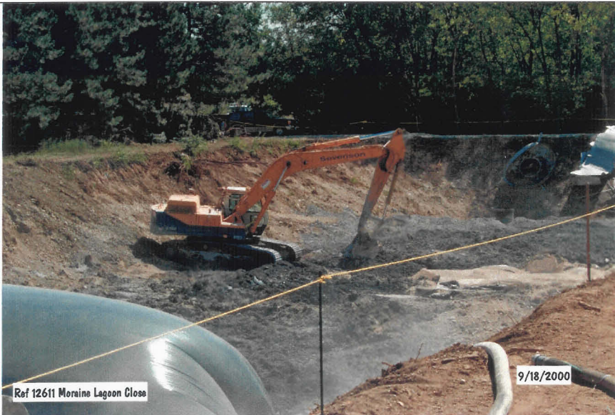
Photograph No. 14 Solidifying Sludge - South Lagoon - Primary Basin Mixing sludge with CKD. Looking southeast from west bank.
