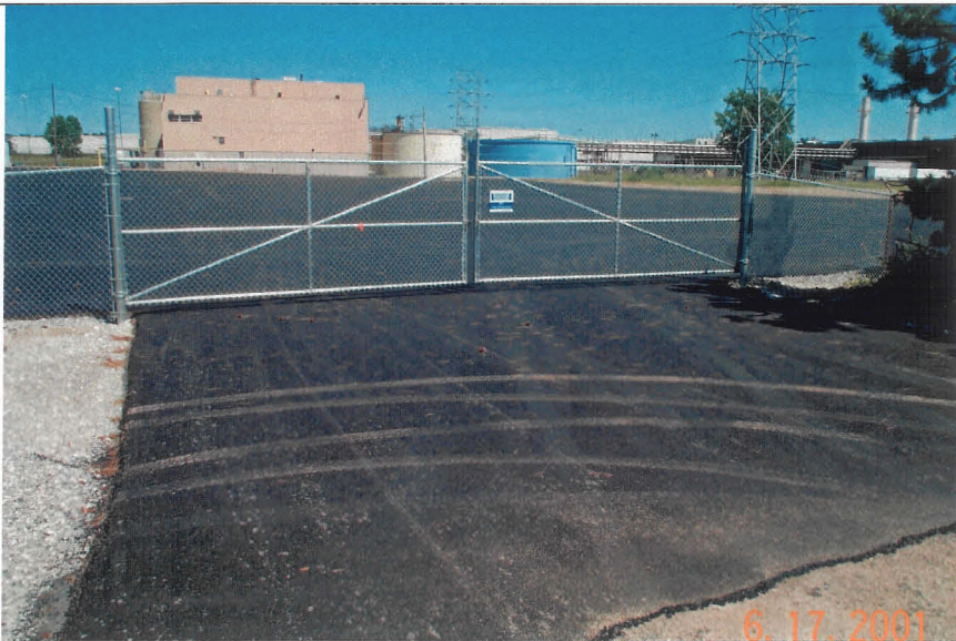
Photograph No. 45 Completed Cover - North Lagoon Completed asphalt cover and new locked gate. Looking eastward at new gate along west side.
