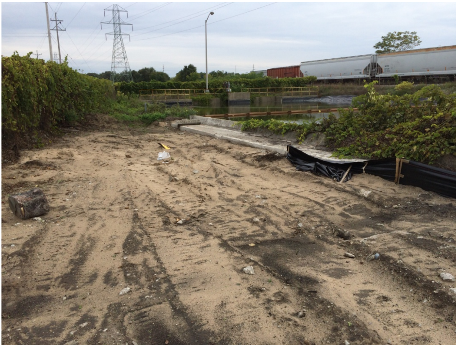
Photo 2 – View of former skimmed oil AST area subsequent to tank and concrete removal
