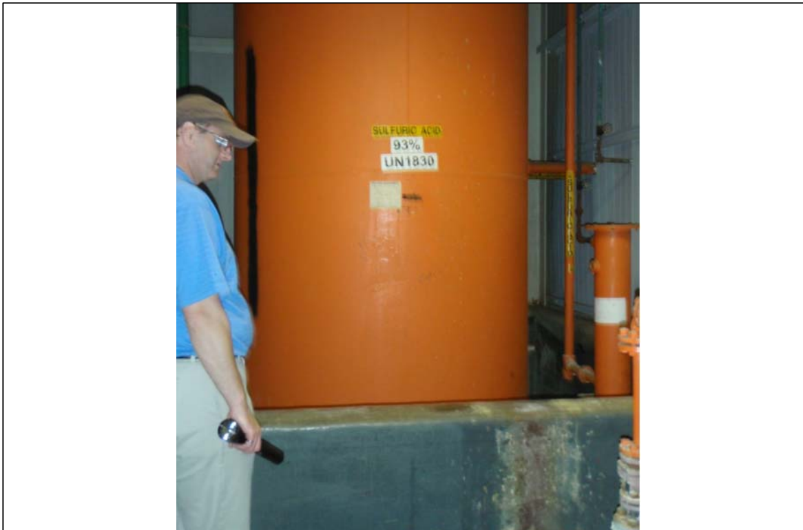
PHOTO 9: Sulfuric acid tank (AST "V")
