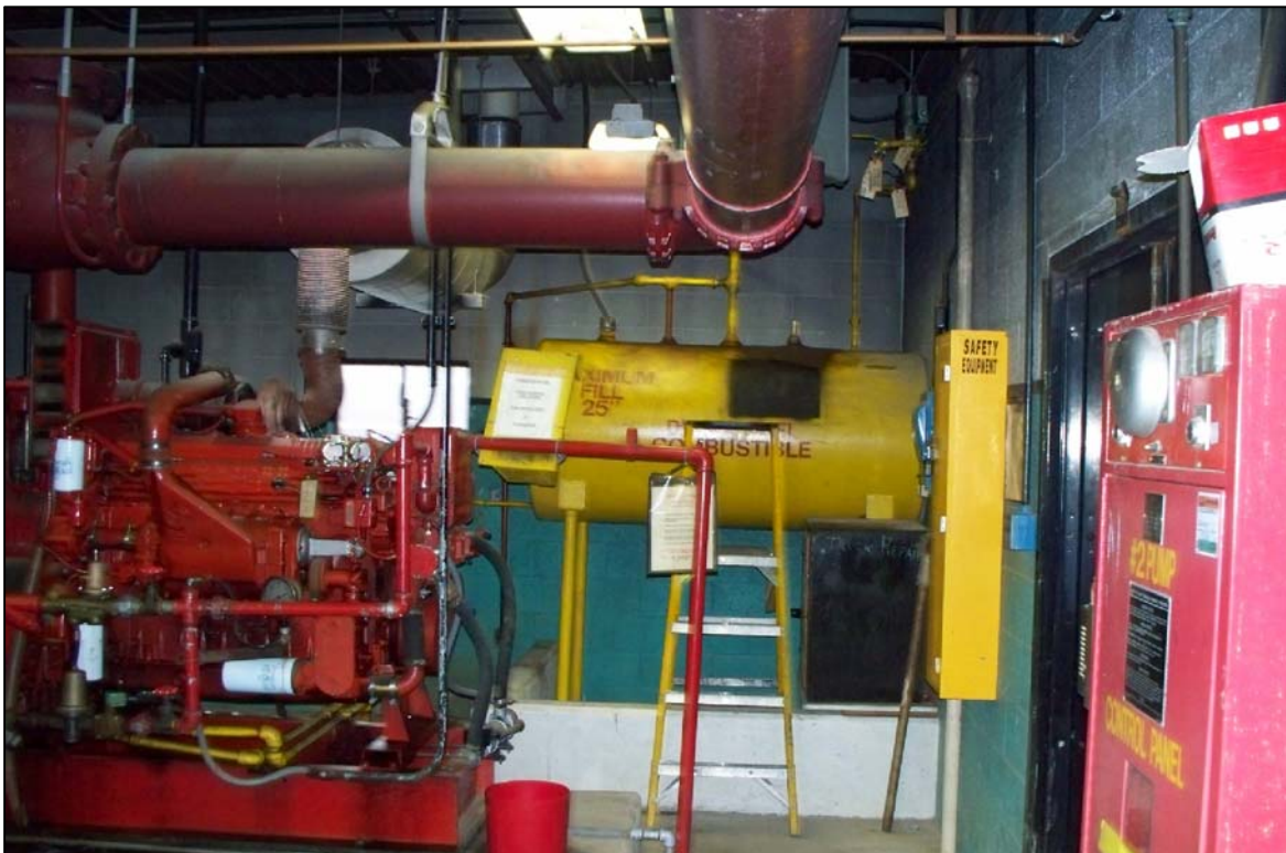
PHOTO 12: One of three diesel ASTs in Pump House No. 2
