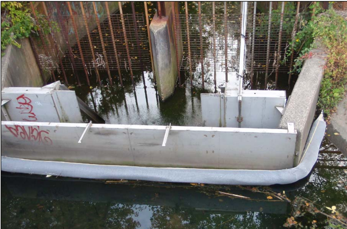
PHOTO 26: Stormwater sluice gate
