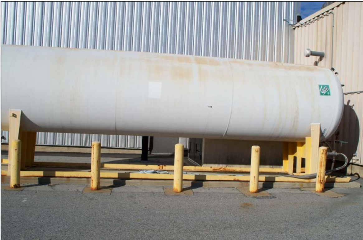
PHOTO 10 : SUVA (Refrigerant) Tank (AST "W")
