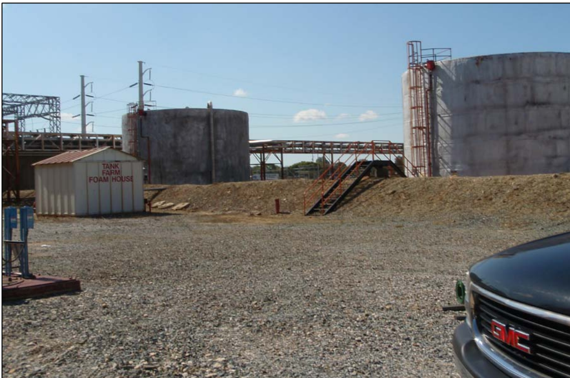
PHOTO 4: ASTs "F" and "G" - Facing west
