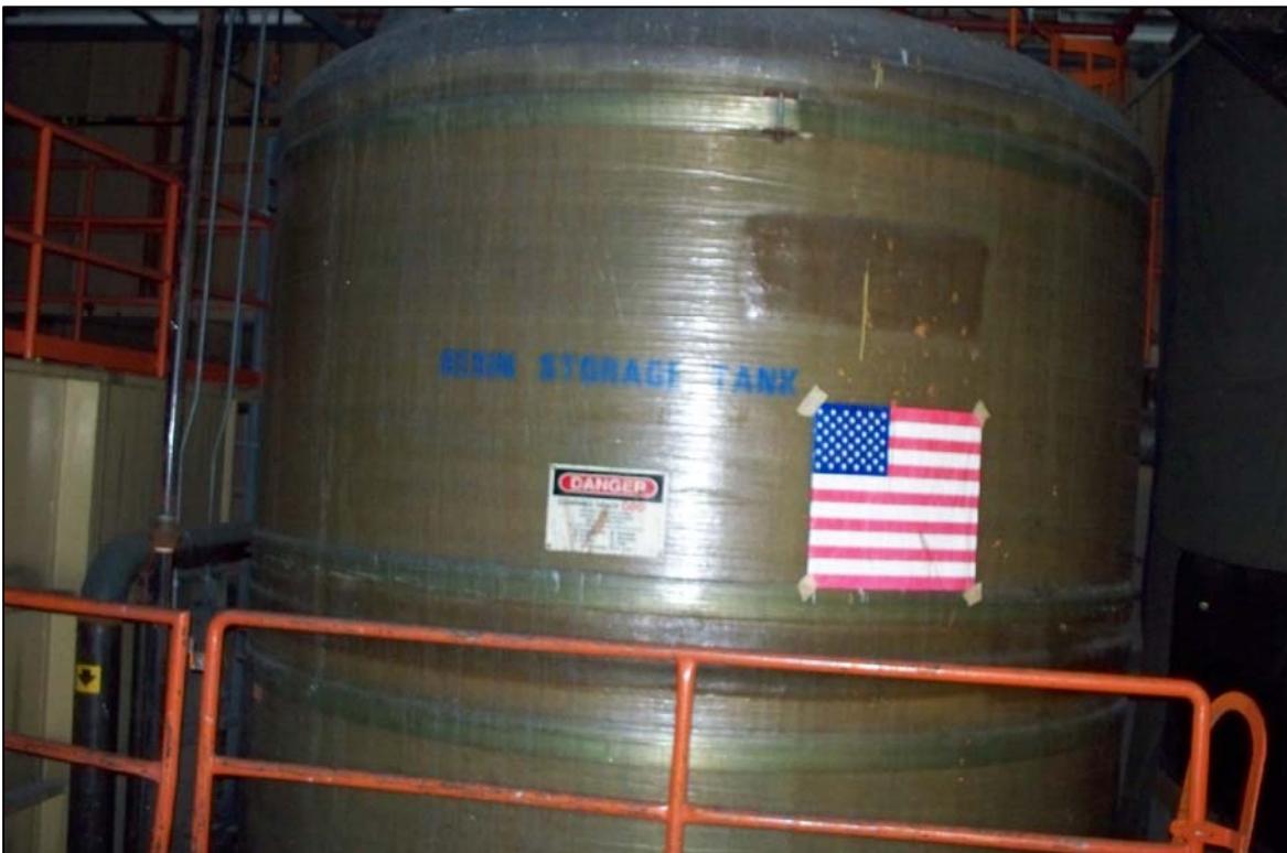
PHOTO 8: ELPO Resin Storage Tanks (AST "U")
