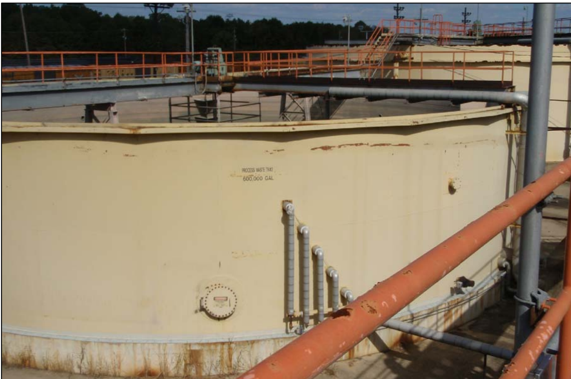
PHOTO 14: WWTP Holding Tank
