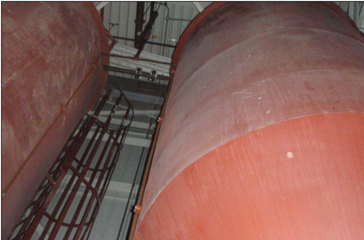
PHOTO 5: Waste Solvent Tanks (ASTs "P" and "Q")
