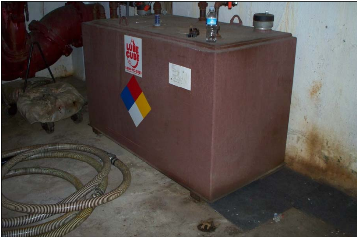
PHOTO 17: Diesel AST in Power House
