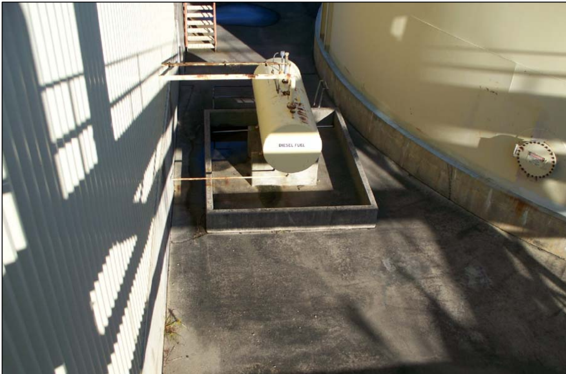
PHOTO 15: WWTP Diesel AST
