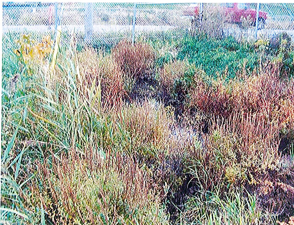
Photograph 13: Blocked catch basin at CB-1.
