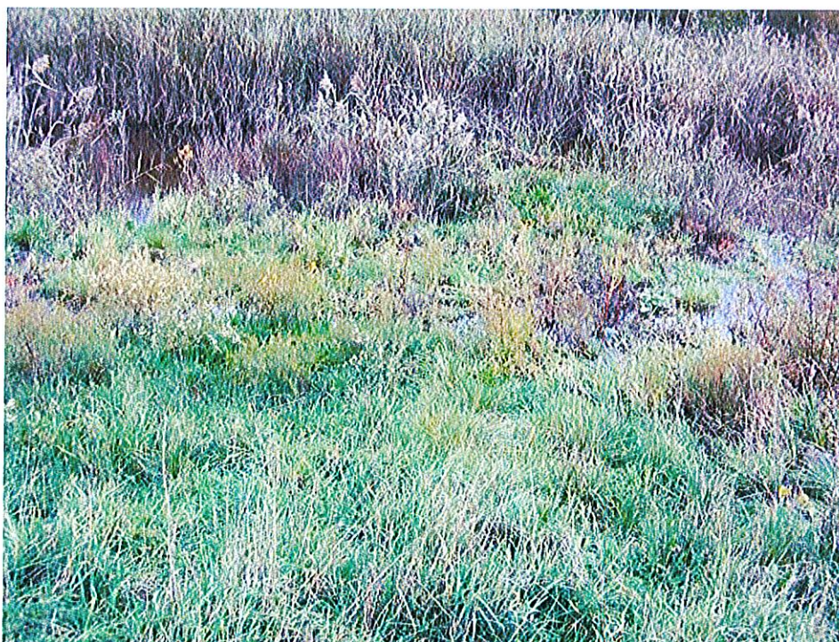
Photograph 14: Scour at CB-1 spillway into Ley Creek.
