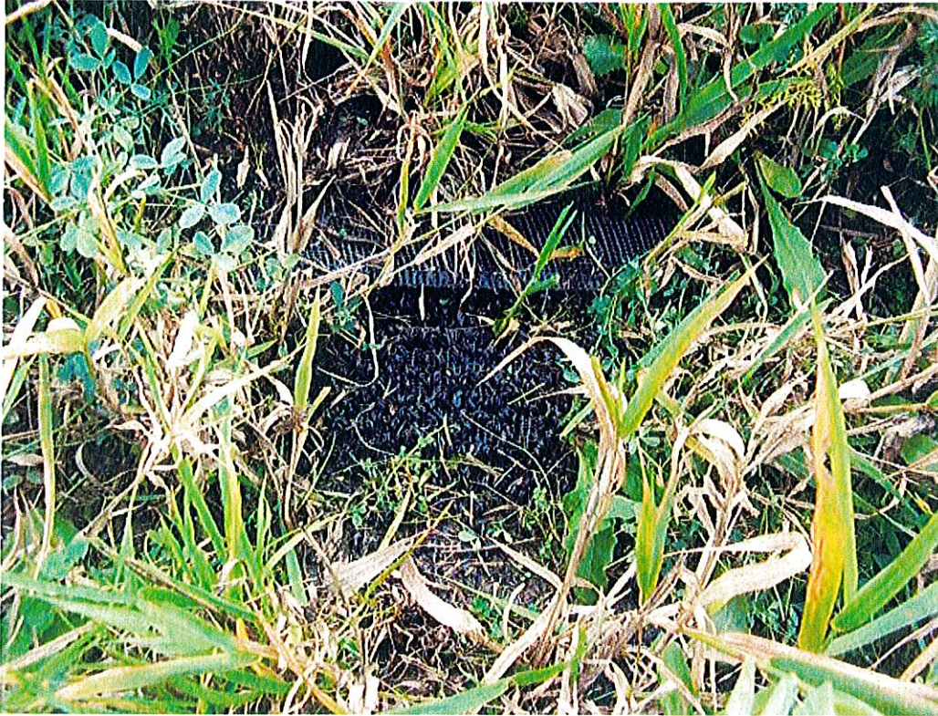
Photograph 1: Exposed erosion fabric in CB-5/Outfall 004 spillway.
