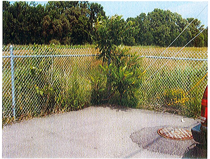
Photograph 10 - Tree growing along fence line at CB-1
