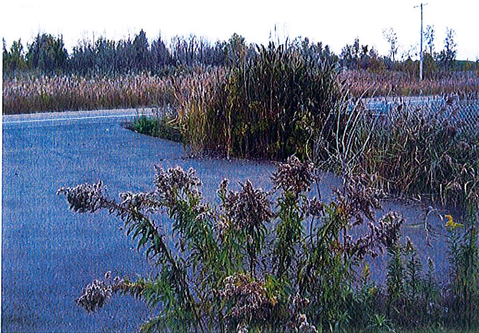
Photograph 11: Vegetation through asphalt.
