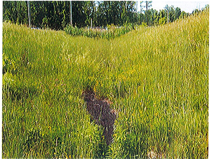
Photograph 6 - CB-3 overflow with exposed erosion control fabric.
