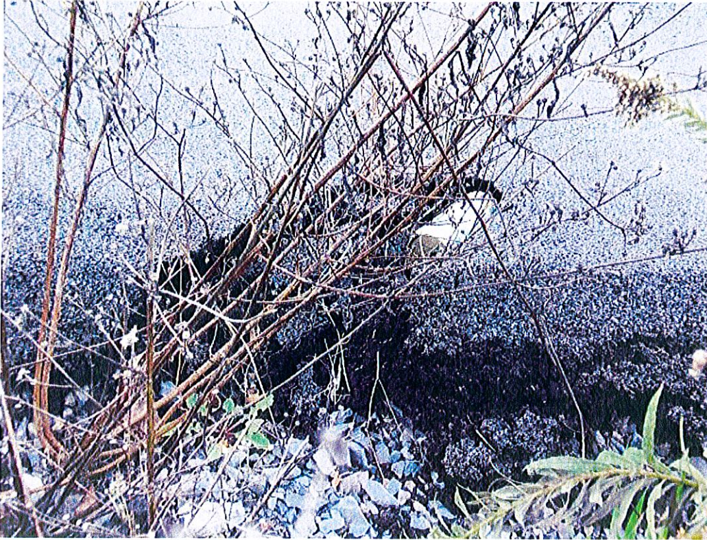
Photograph 9: Pavement depression/erosion with debris.
