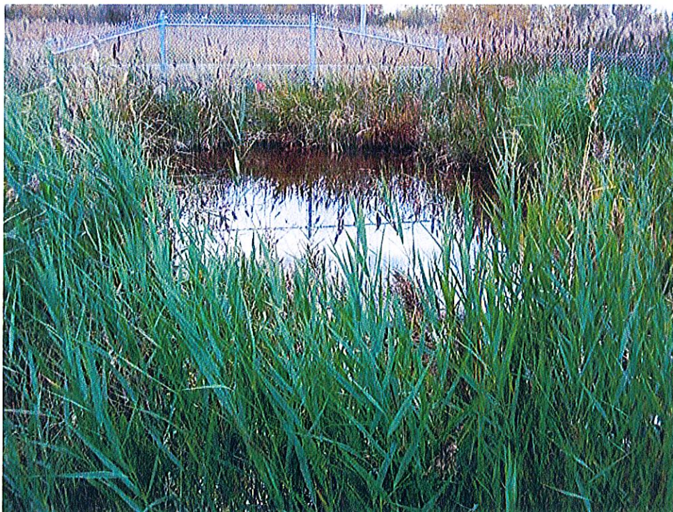
Photograph 12: Blocked catch basin grate at CB-2.
