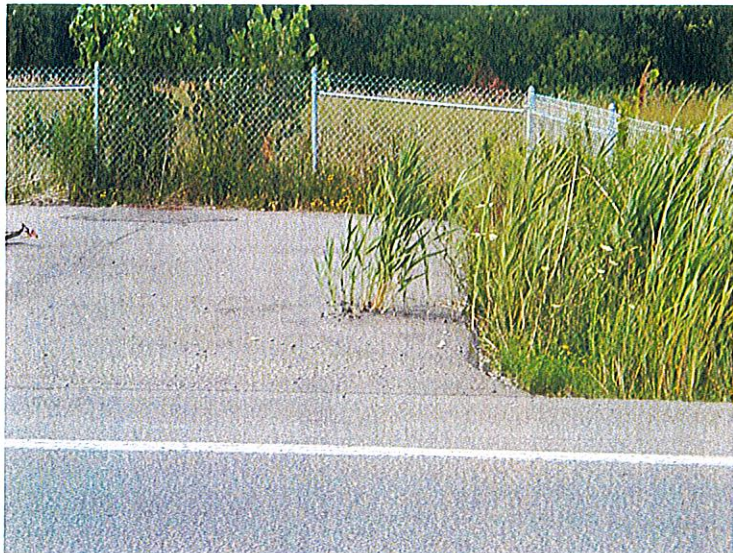
Photograph 11 - Vegetation in pavement and trees along fenceline
