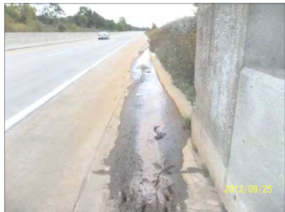
Drainage pattern. Note—no other water in curb and gutter. Photo direction northeast.
