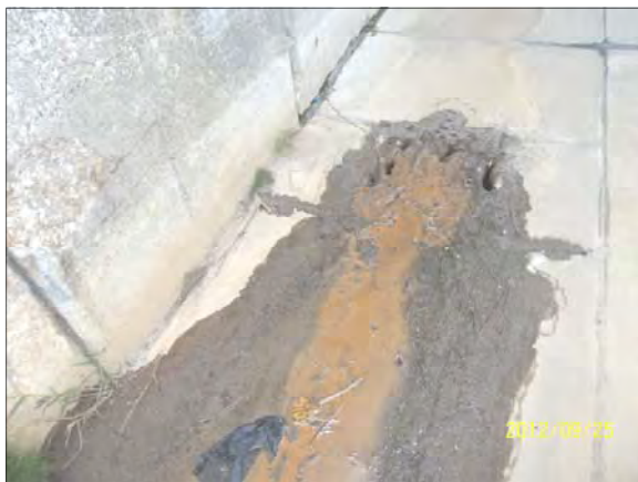
Catch basin on Michigan Ave., under CSX overpass where water is draining.
