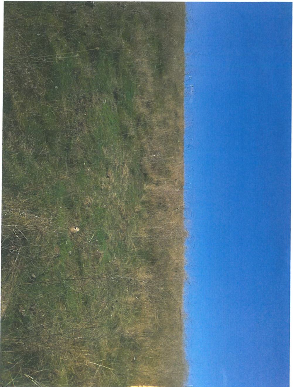
View (to West) of Recently Repaired Washed-Out Area on Eastern Slope of Landfill Near Monitoring Well B-24r
