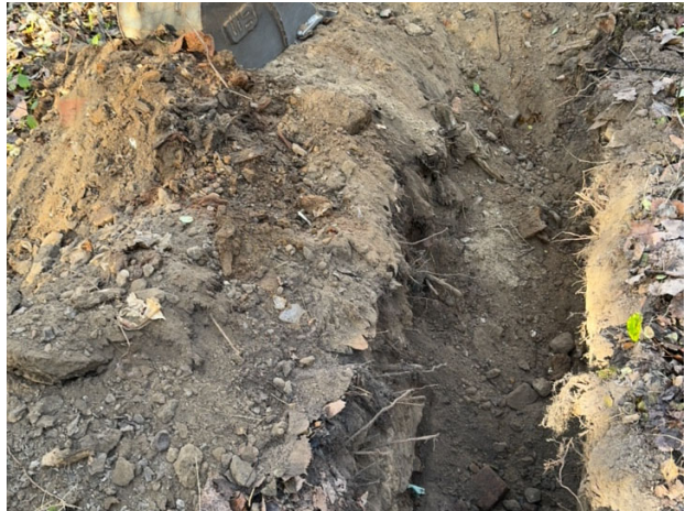
TP-109_0-2_11062024 Debris Present
