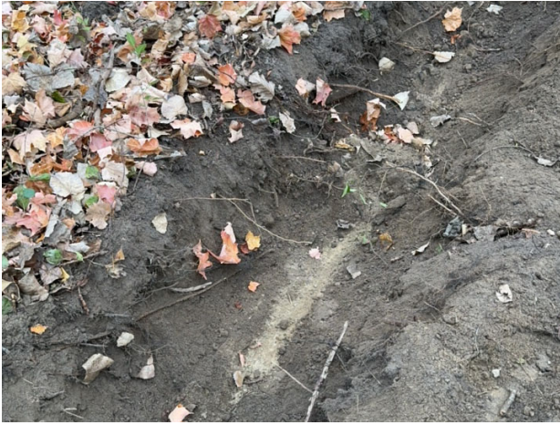
TP-100_0-2_111052024 Debris present
