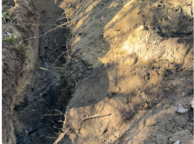
TP-131_0-4_11072024 Debris present
