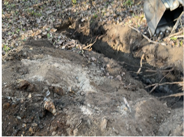
TP-139_0-3_11072024 Debris present
