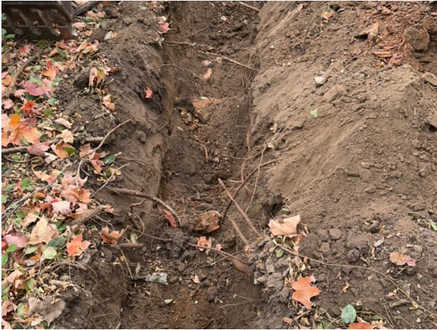
TP-102_0-2_111052024 Debris present
