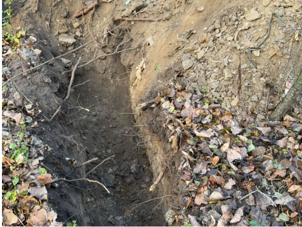
TP-112_0-3_11062024 Debris present
