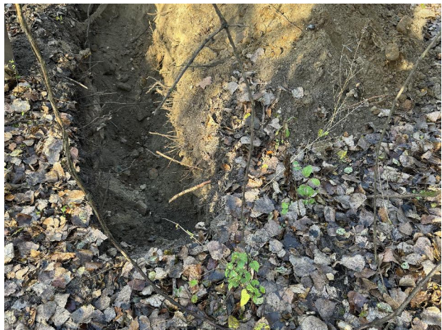
TP-111_0-3_11062024 Debris present
