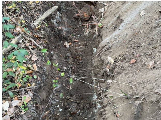
TP-105_0-2_111052024 Debris present
