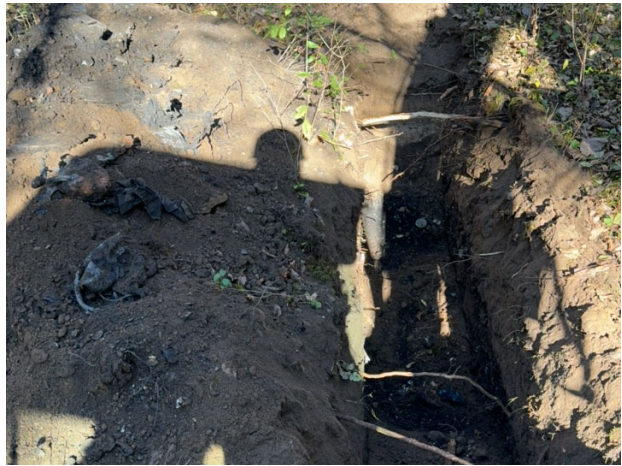
TP-133_0-4_11072024 Debris present
