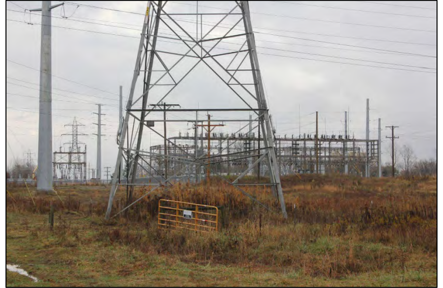
Photo 30: Close up of power substation, looking southeast.
