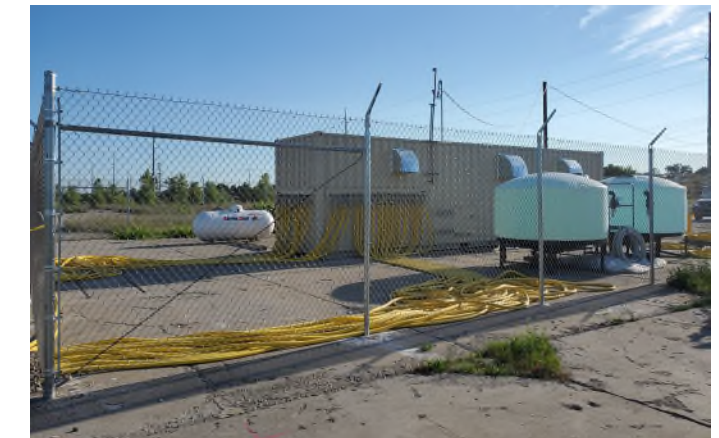
Plant 2 Biosparge Unit and Nutrient Injection Tanks
