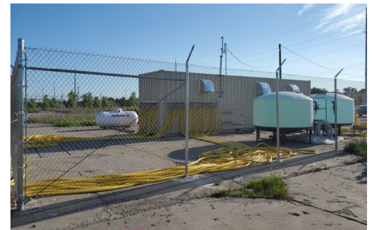
Plant 2 Biosparge Unit and Nutrient Injection Tanks
