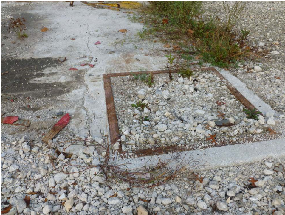
Photograph 19. (AOI-02) Concrete pad at former industrial waste pump house. Note staining on concrete and sump feature. Photo taken from northeast edge of feature, facing west. Red colored objects appear to be metal fragments of a former hydrant.
