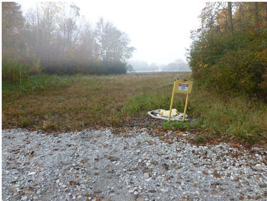
Photograph 8. (AOI-01) Photo taken at northeastern area of Site, facing south. Gravel is present in former AST area.
