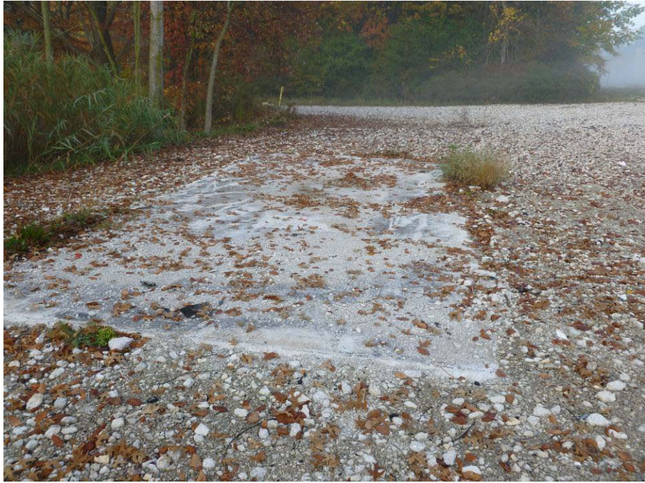
Photograph 15. (AOI-01) Pump pad concrete pad, located southeast of AST area. Photo taken facing west.
