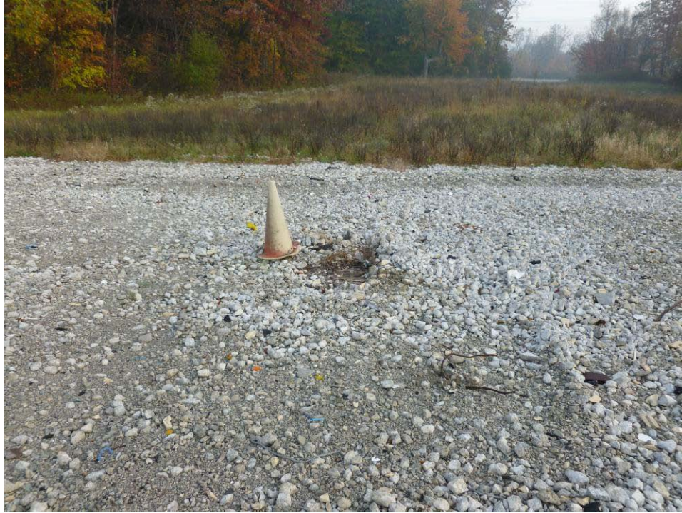
Photograph 33. Storm drain located at edge of former exterior concrete parking area, north side of former facility footprint.
