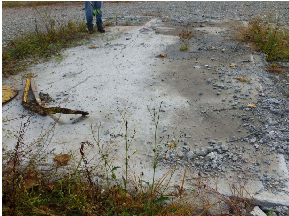
Photograph 18. (AOI-02) Concrete pad at former industrial waste pump house. Note staining on concrete. Photo taken from southwest edge of feature, facing east.
