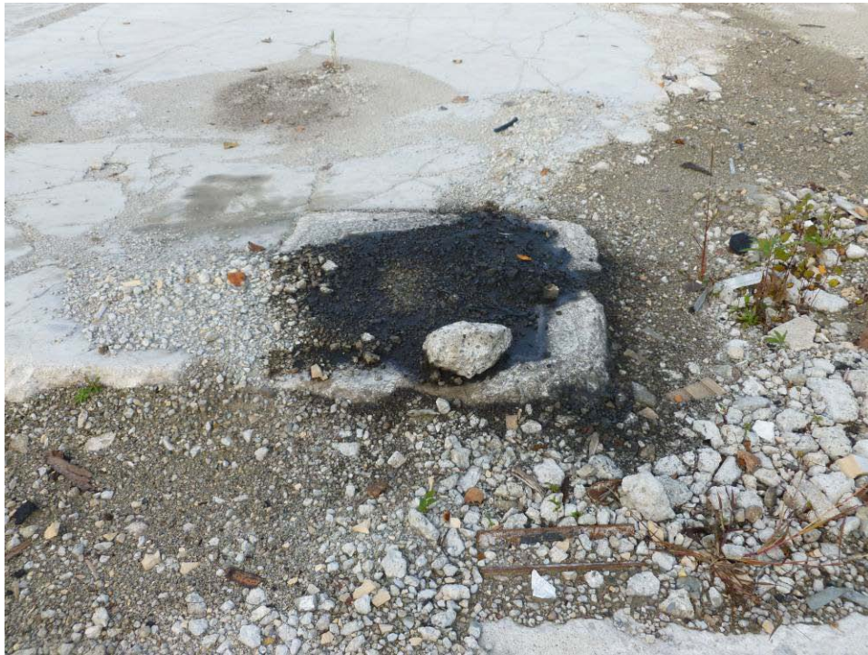
Photograph 27. (AOI-04) Dark, oily staining observed on concrete in eastern portion of former facility. Location believed to be outside of southeast corner of Test Cell "D" Wing. Material may be associated with building demolition or post-demolition activities.
