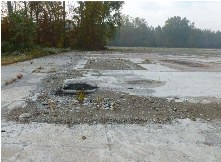
Photograph 28. (AOI-04) Note dark, oil staining on concrete in eastern portion of former facility. Photo taken facing south. Location believed to be outside of southeast corner of Test Cell "D" Wing.
