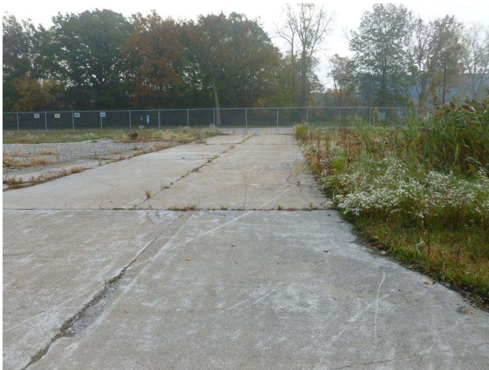
Photograph 25. (AOI-06) Access to east area of facility, leading to area of baghouse, cold test trailer and closed UST. Photo taken facing east.
