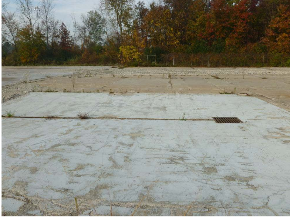
Photograph 35. (AOI-07) Area of former shipping dock and drum storage shed. Photo taken facing west.
