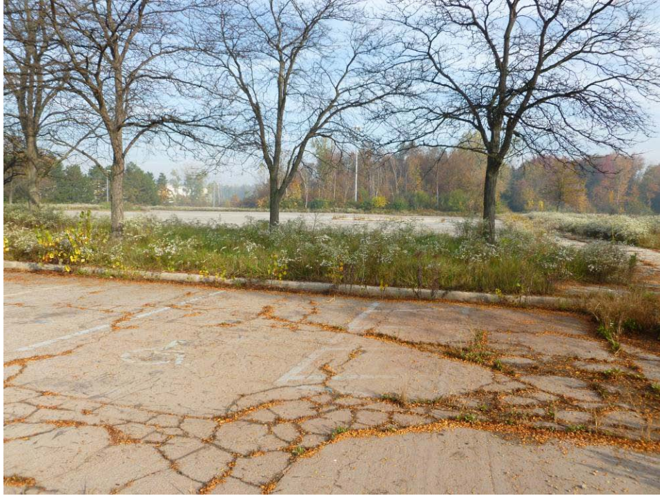
Photograph 37. Photo taken from parking lot located on west side of Site, facing east across former facility footprint.
