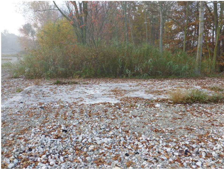
Photograph 16. (AOI-01) Pump pad concrete pad, located southeast of AST area. Photo taken facing east.
