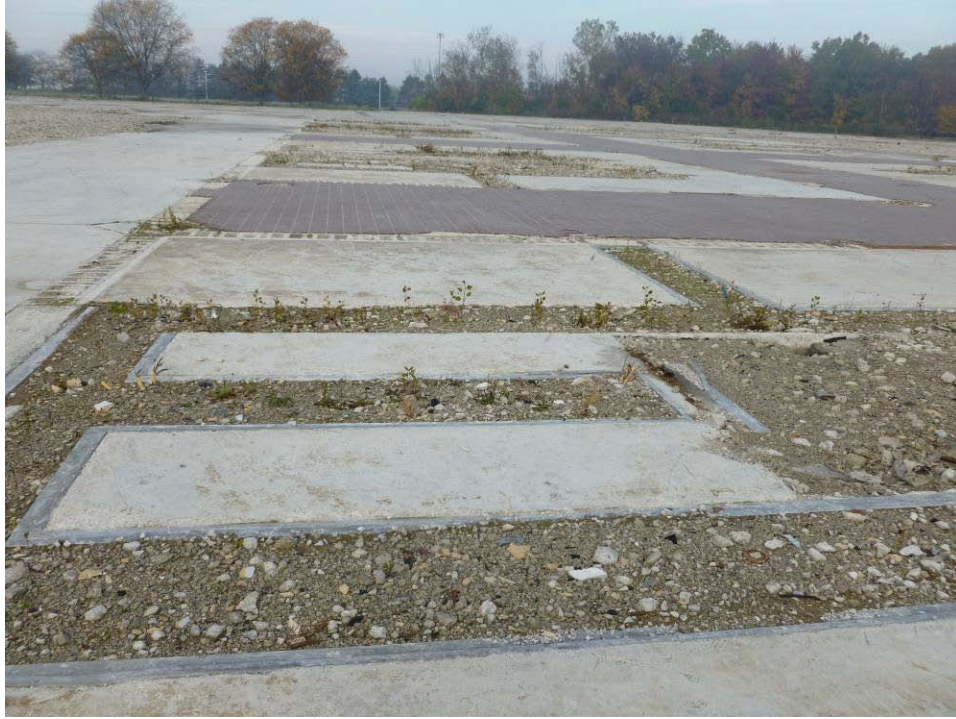
Photograph 29. Concrete tile features in footprint of former facility. Areas believed to be former dynamometer testing areas and tiled aisles, Test Cell "E" Wing. Photo taken near eastern area of former facility, facing west.
