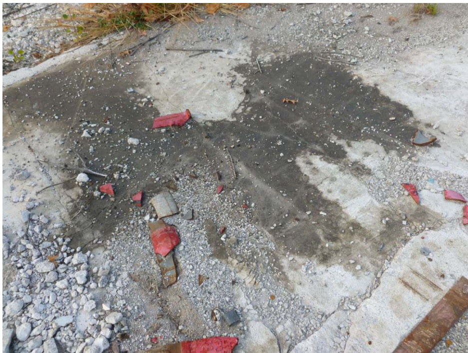
Photograph 20 (AOI-02) Close-up of staining on concrete pad at former industrial waste pump house.
