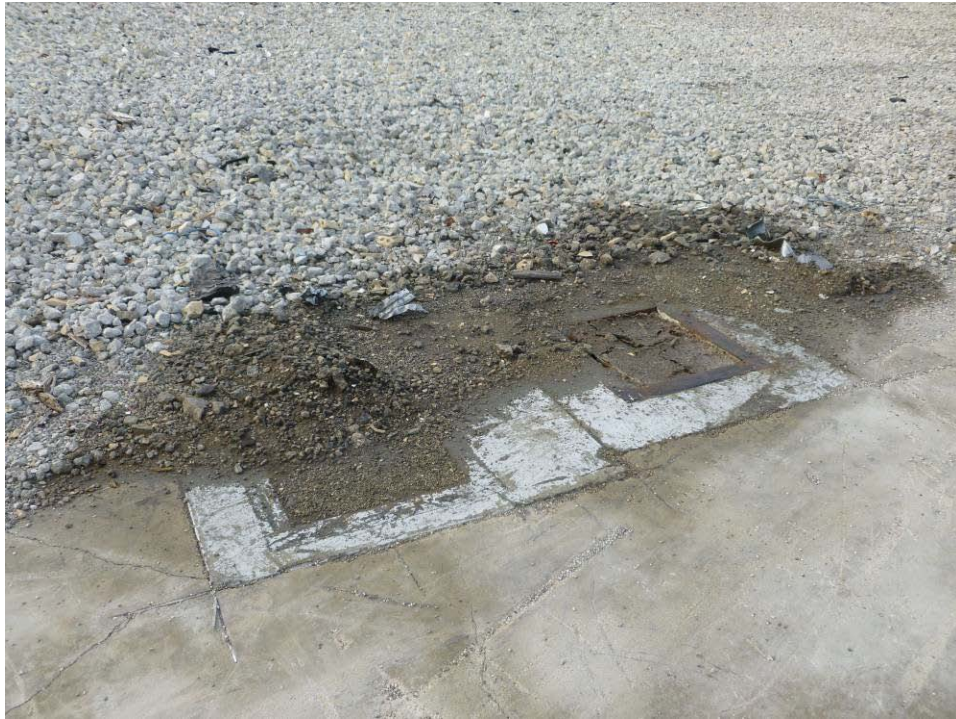
Photograph 31. (AOI-05) Staining observed on concrete and gravel in footprint of former facility. Location believed to be northeast area of Test Cell "E" Wing.
