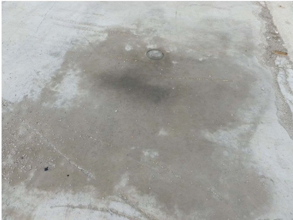
Photograph 30. Light staining observed on concrete in footprint of former facility.
