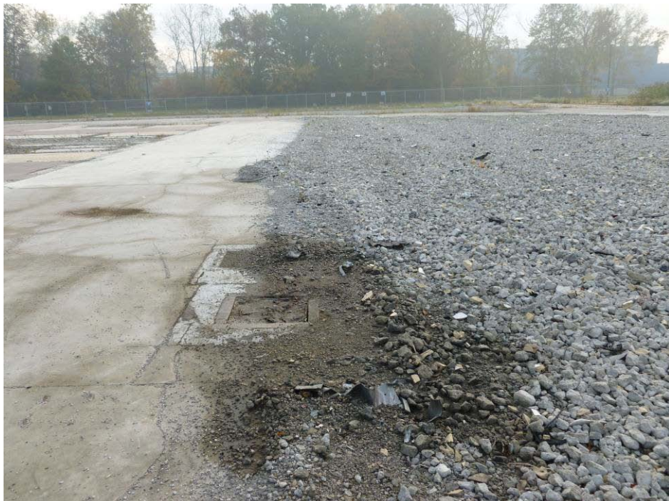
Photograph 32. (AOI-05) Staining observed on concrete and gravel in east central portion of former facility footprint. Location believed to be northeast area of Test Cell "E" Wing. Photo taken facing east.
