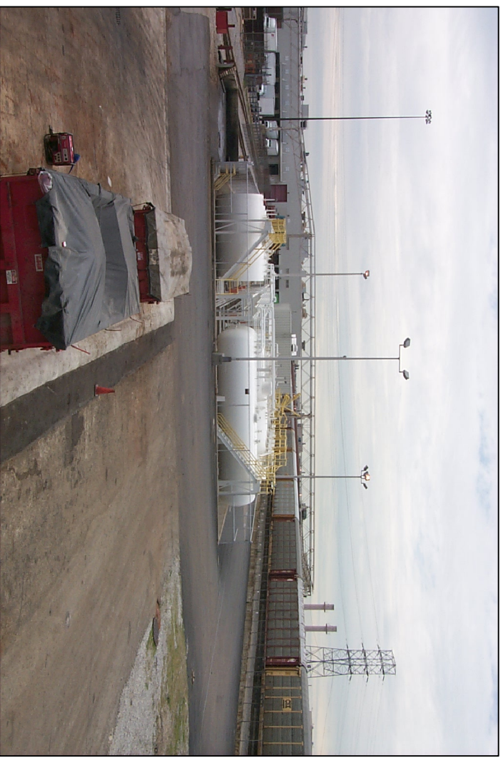
VIEW FACING SOUTH, WITH CHIP PAD IN THE FOREGROUND AND MORAINE ENGINE TANK FARM IN THE BACKGROUND.
