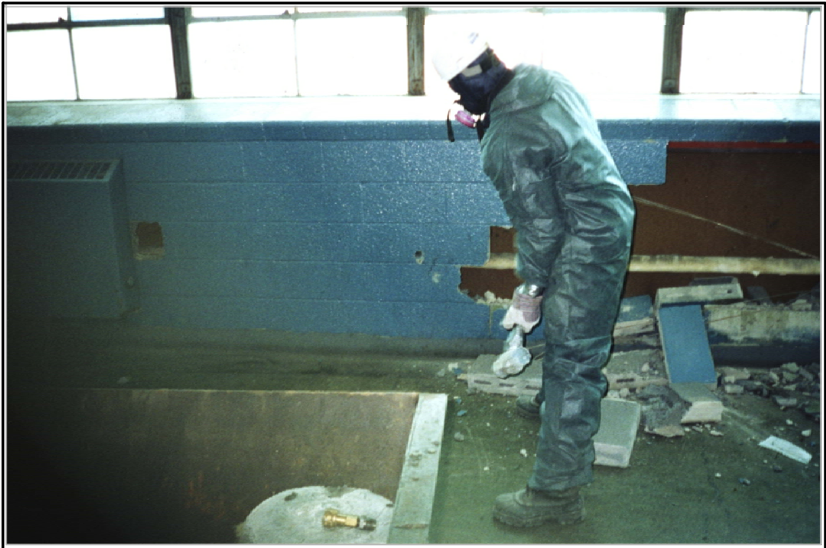
PHOTO #3 EXPOSING ASBESTOS PIPING
