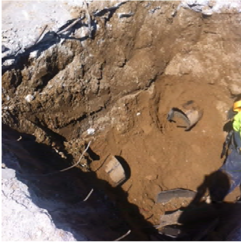
Photo 5: View of cut/separation of pipe at bulkhead location #3.
