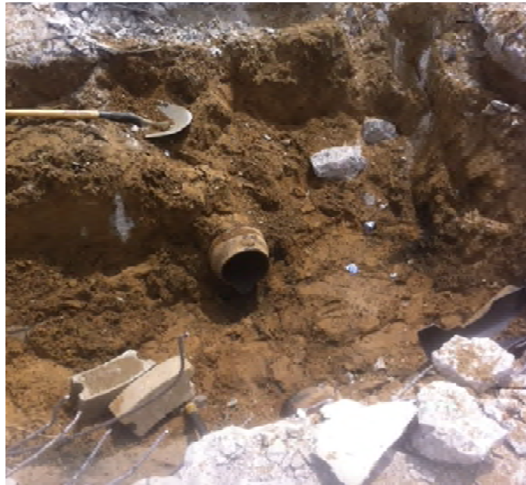
Photo 4: View of cut/separation of pipe at bulkhead location #2.
