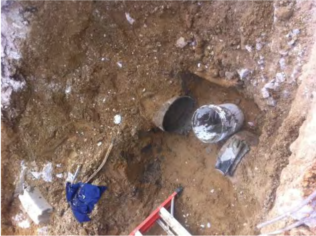
Photo 1: View of cut/separation of pipe at bulkhead location #1.
