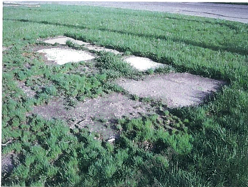
Photo 7: Concrete patches along northern portion of Site
