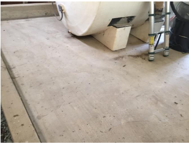
Photo #3: Concrete pad of secondary containment system
