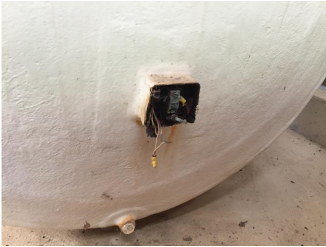
Photo #7: Termination of electrical feed
