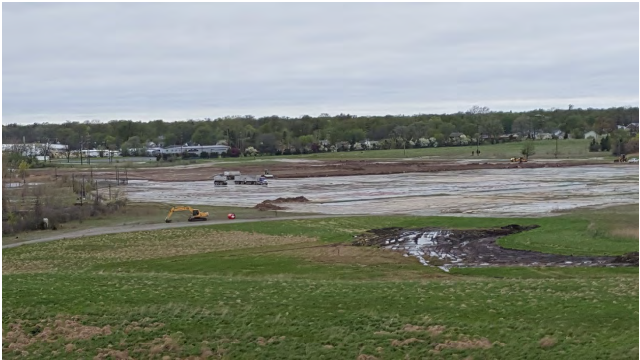
Photo 3 – May 2, 2017 – Concrete Floor Slab and Compensating Cut Area from Greenpoint Landfill – Clay Placement
