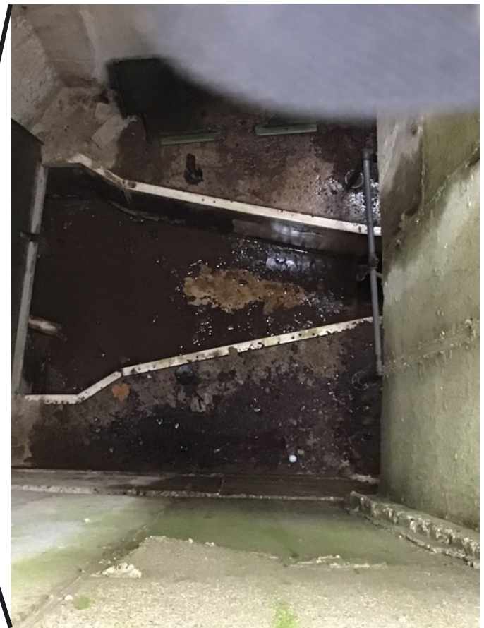
Trickle flow observed in sanitary sewer outfall
