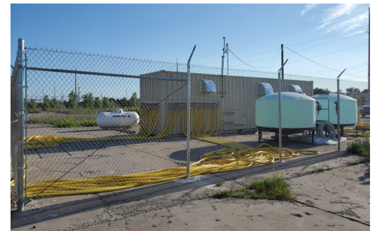
Plant 2 Biosparge Unit and Nutrient Injection Tanks
