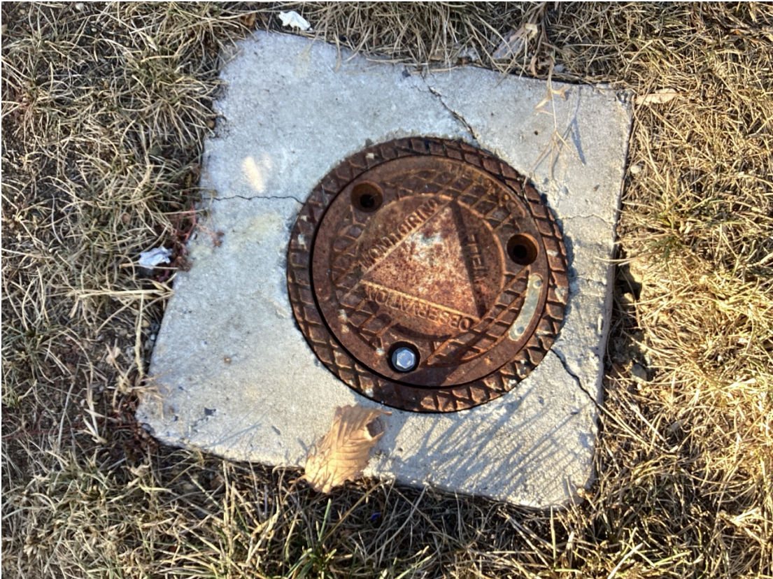
Photo 1: Outside of well
