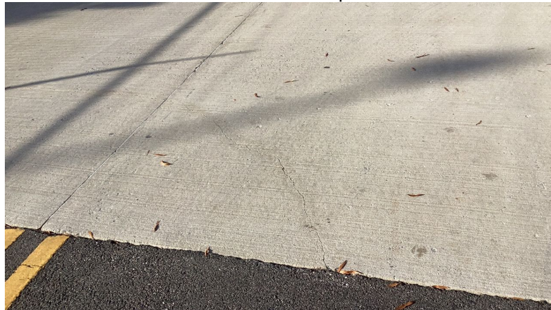
Photo 1 - Small crack as road turns into concrete cap.
