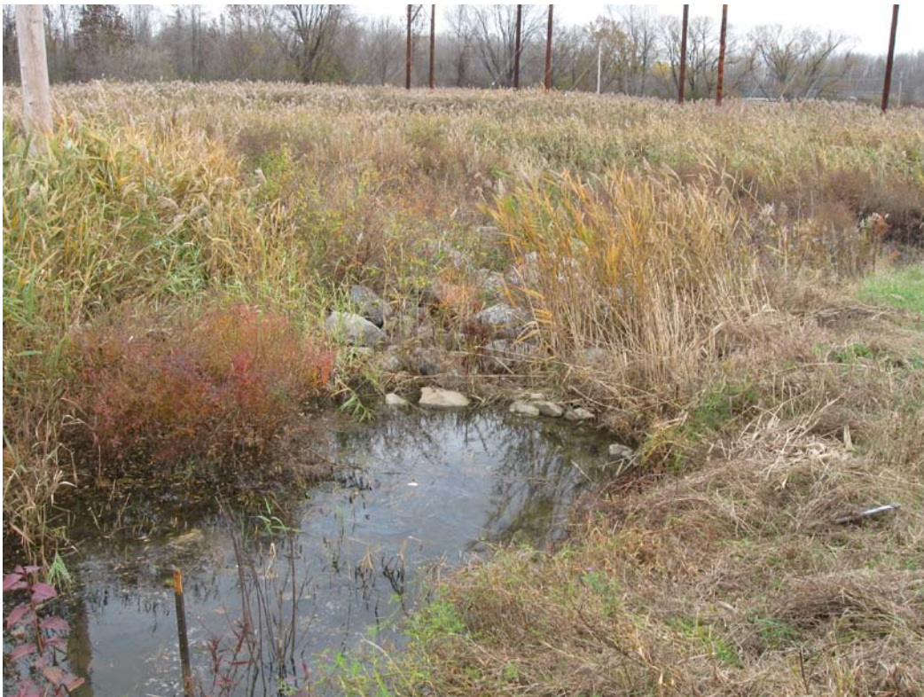
Photograph 4: View of CB-04. Plugged.
