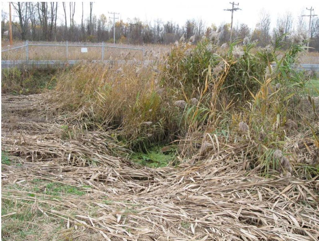
Photograph 8: View of CB-03. Not overflowing, but plugged.
