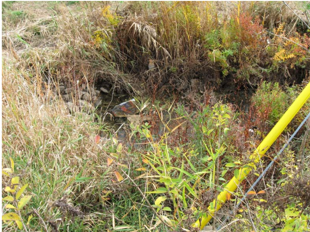
Photograph 14: View of CB-01. Plugged.
