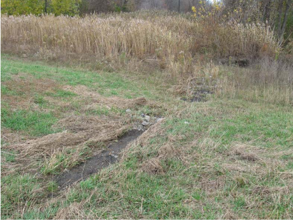
Photograph 9: View of scoured section of CB-03 overflow channel.
