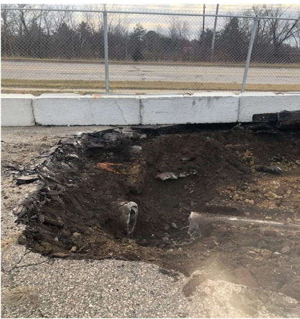
Example of disconnected line. Sewer line excavated, disconnected and temporary plugged prior to sealing
