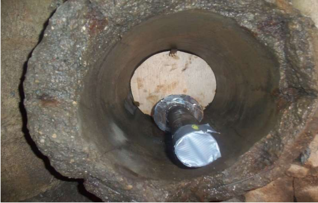
Example of plug on 24" line with flow through pipe still in place
