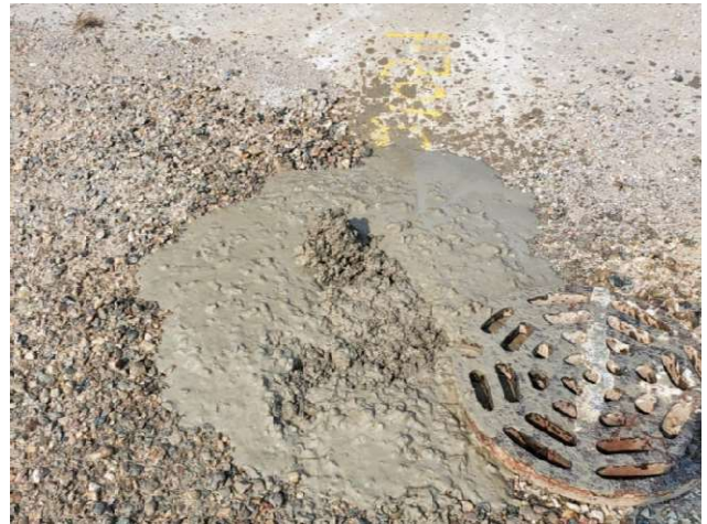
Filled manhole (on left) to grade, prior to finishing. Former cover on right.
