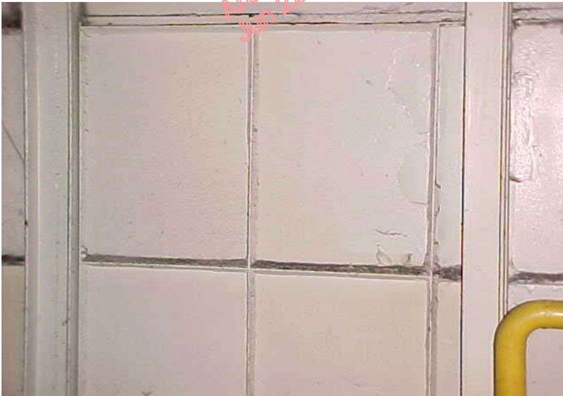
ACM Paint on Windows Located in Main Plant and Oil Storage
