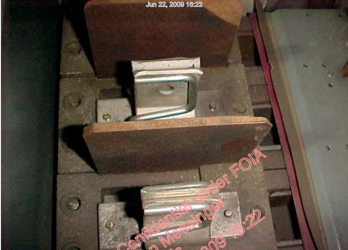
Panels with Asbestos Paper, Transite Backing and Asbestos Block
