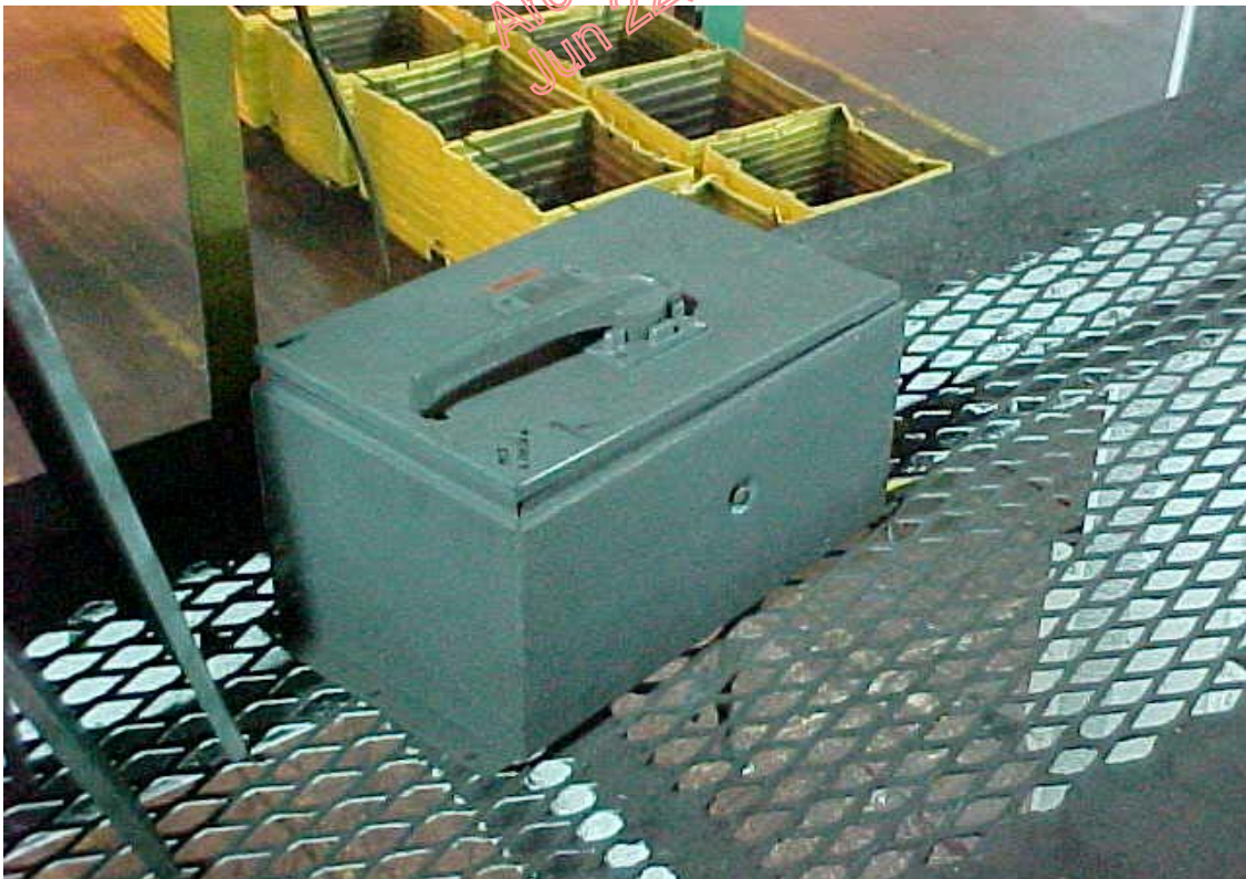
As Shown Above, No Insulation on Handle = Asbestos Inside Unit
