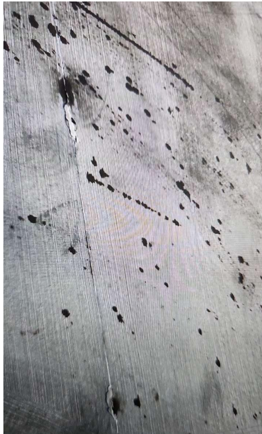
Photo 8 Cap concrete showing filled small wear areas that have been filled
