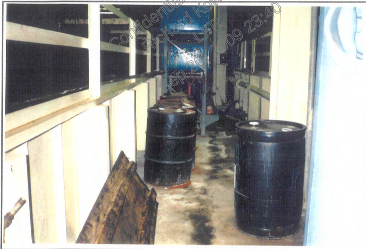
PHOTOGRAPH 4: STAINED CONCRETE FLOOR IN BUILDING 45
