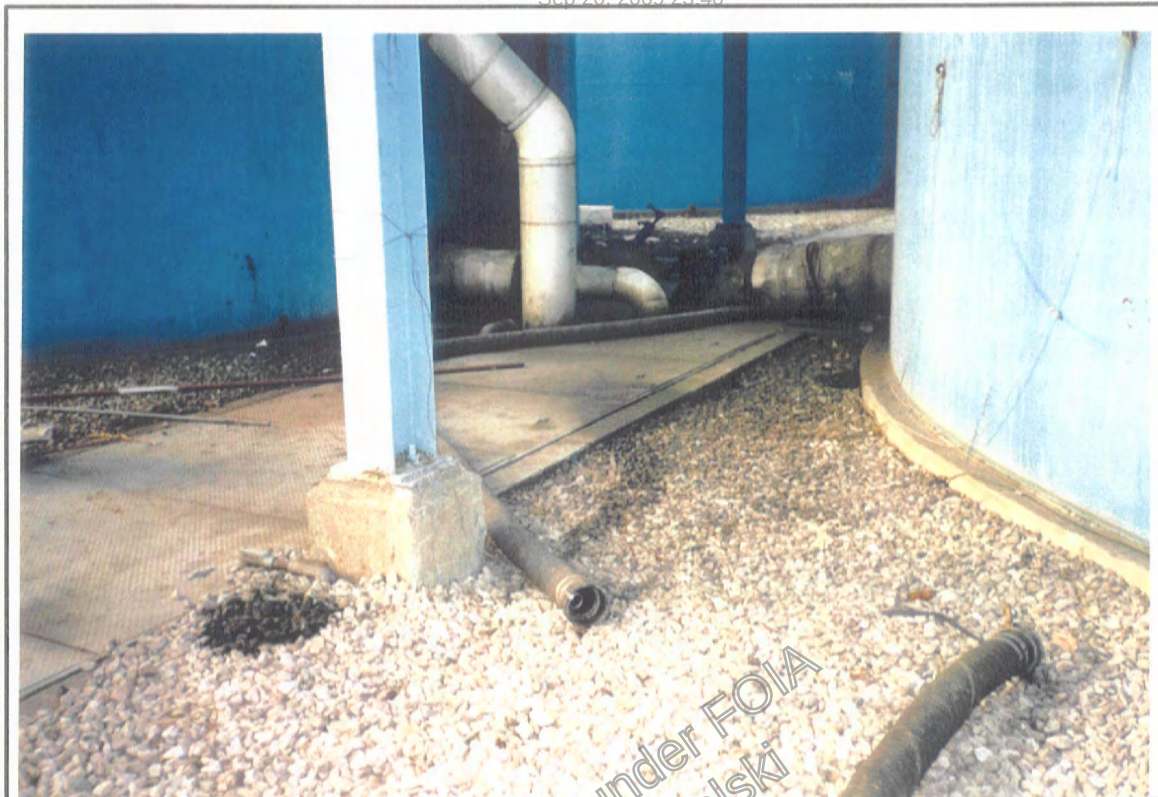
PHOTOGRAPH 7: STAINED GRAVEL BETWEEN OILY WASTE TANK NO. 3 AND FLOTATION RECYCLE TANK
