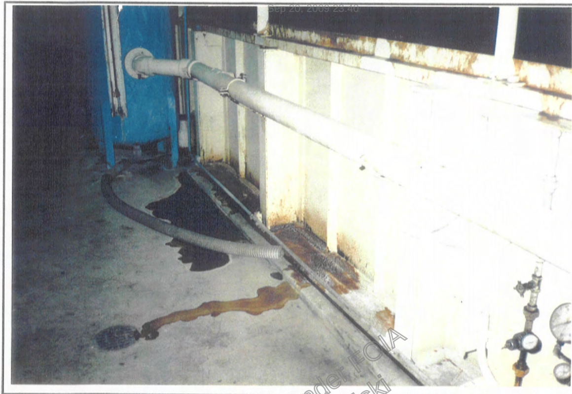
PHOTOGRAPH 5: LEAKAGE TO FLOOR DRAIN IN BUILDING 45 ADJACENT TO FLOCCULATION UNIT
