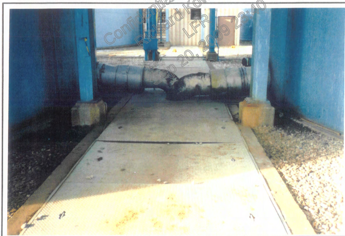
PHOTOGRAPH 10: STAINED GRAVEL BETWEEN OILY WASTE TANK NO. 1 AND OILY WASTE TANK NO. 2
