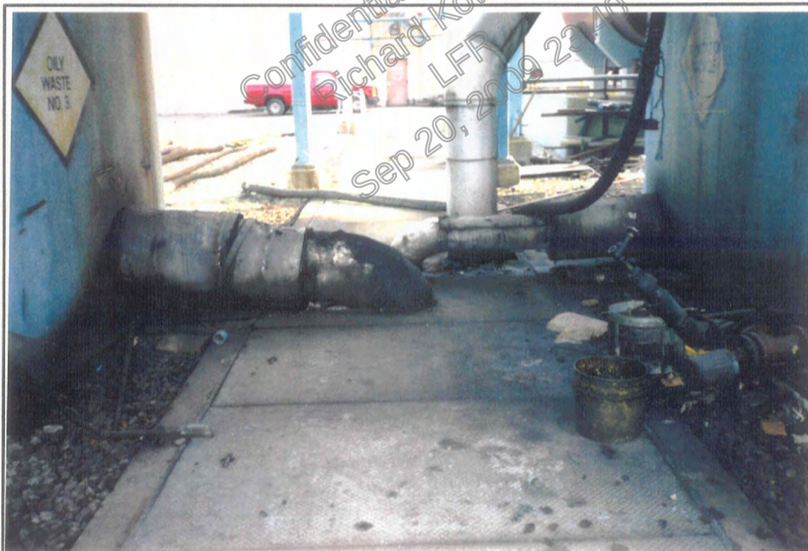
PHOTOGRAPH 8: STAINED GRAVEL BETWEEN OILY WASTE TANK NO. 3 AND FLOTATION RECYCLE TANK
