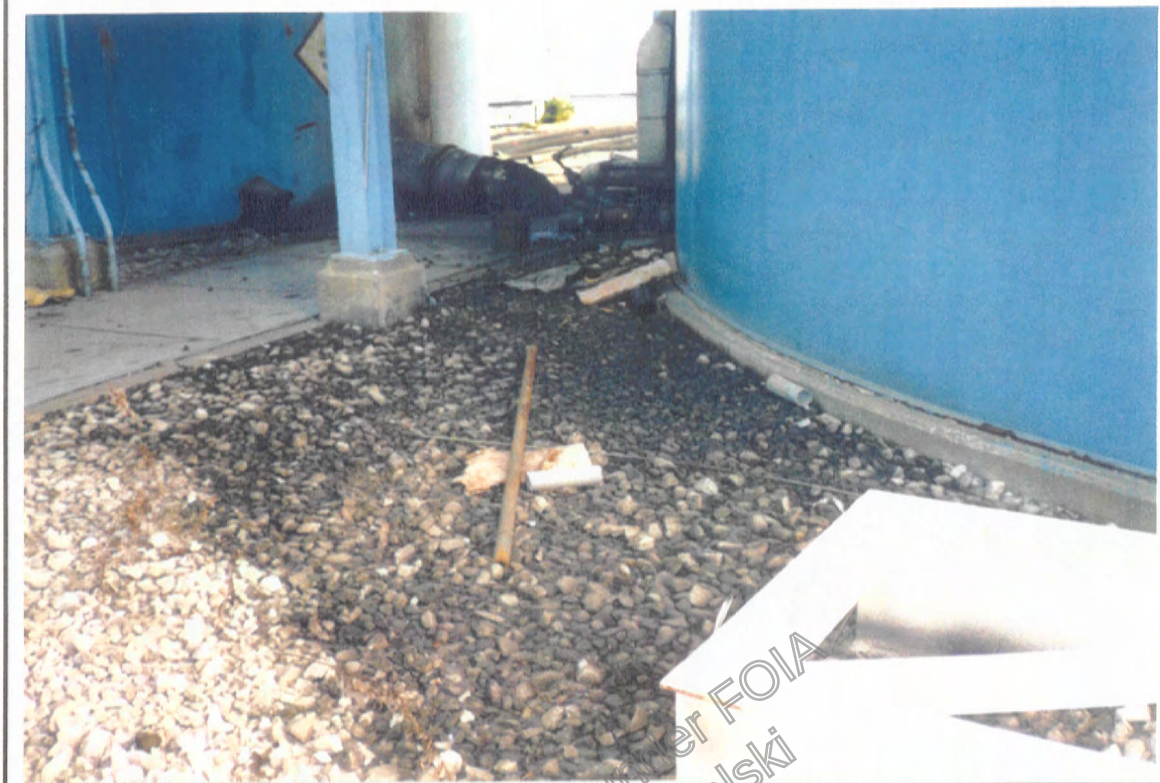
PHOTOGRAPH 9: STAINED GRAVEL BETWEEN OILY WASTE TANK NO. 1 AND OILY WASTE TANK NO. 2
