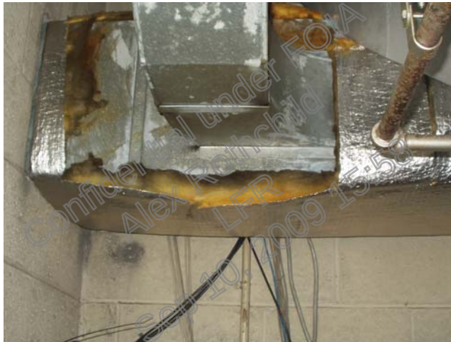
Photograph 19. View of exposed and damaged suspect asbestos containing insulation in air conditioning room on the second floor.
