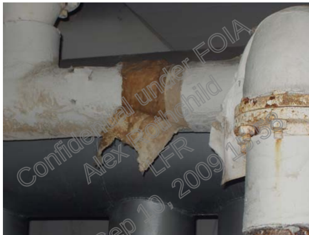
Photograph 11. View of exposed and damaged suspect asbestos containing piping insulation in the boiler room of the basement.
