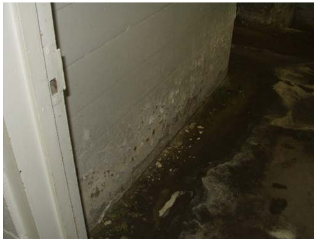
Photograph 12. View of peeling paint in the hallway to the boiler room in the basement.
