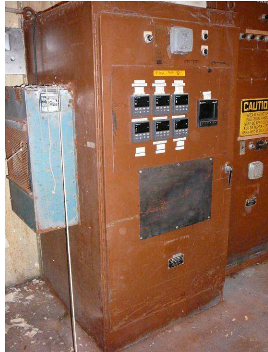
Photo 86. AJAX #1 – Electric Controls (P-074).
