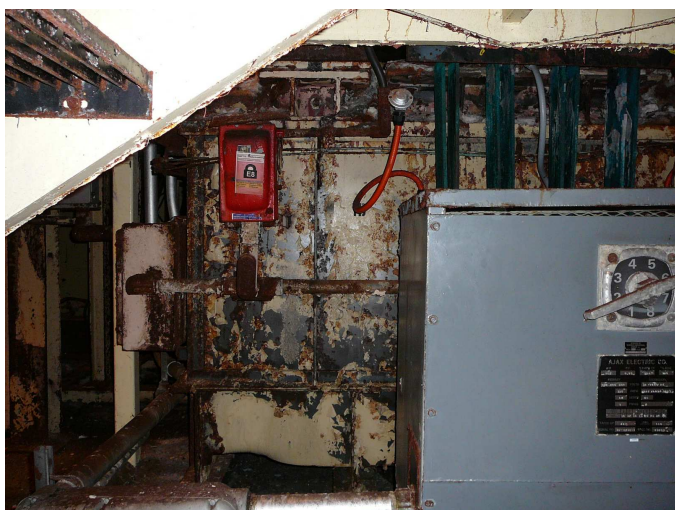
Photo 72. AJAX #1 – Furnace (W-071).
