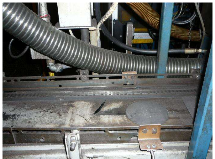
Photo 54. Bonder #1 – conveyor tray (W-052).
