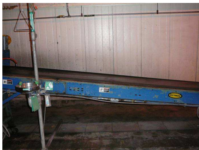
Photo 36. Slurry Area – Conveyor Belt (W-034).
