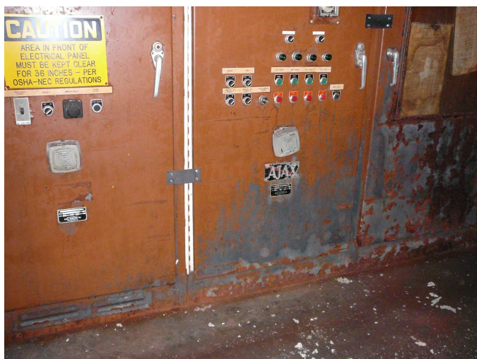
Photo 78. AJAX #2 – Furnace Control (W-077).
