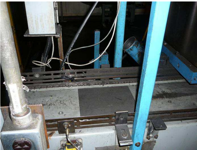
Photo 50. Bonder #5 – conveyor tray (W-048).
