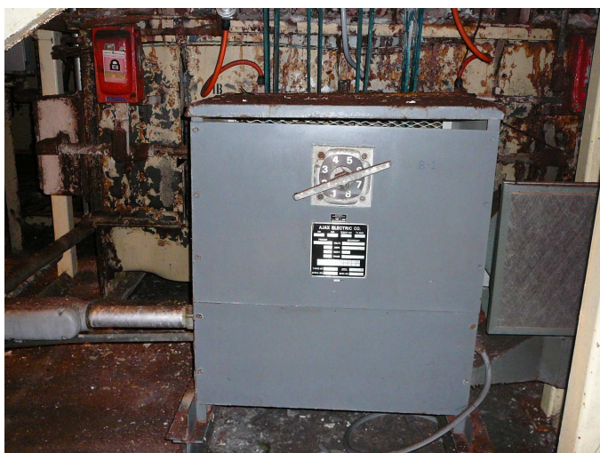
Photo 73. AJAX #1 – Speed Control (W-072)
