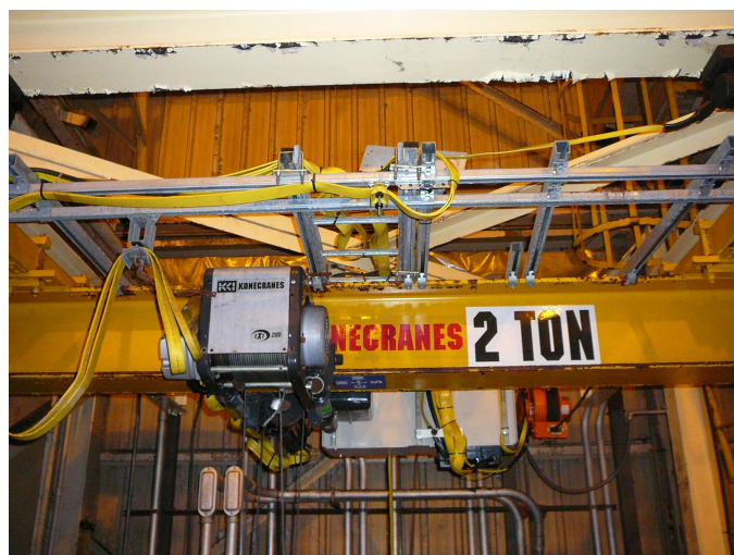
Photo 75. AJAX #1 – Bridge Crane (W-074 / P-075).
