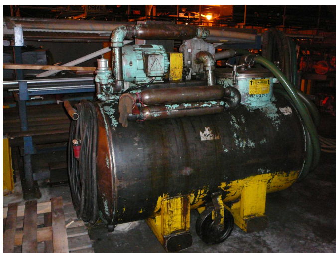
Photo 80. Delco Vacuum Pump (P-027).
