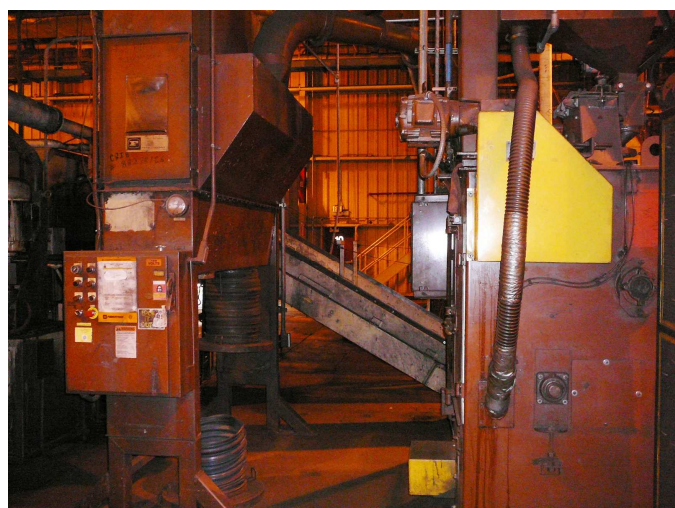
Photo 83. Shot Peen Filtration System (P-068).
