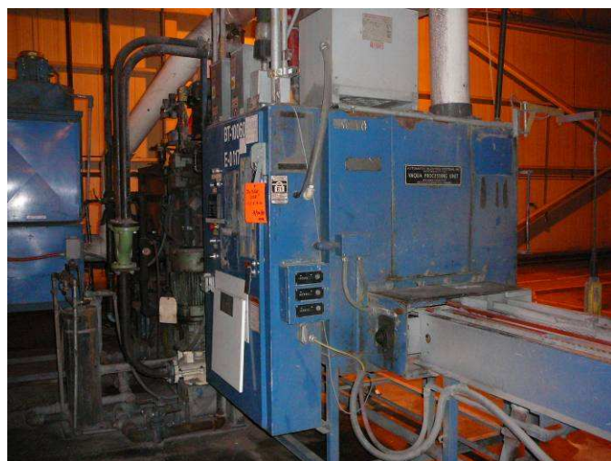
Photo 35. Slurry Area - Vaqua Processing Unit (W-033).
