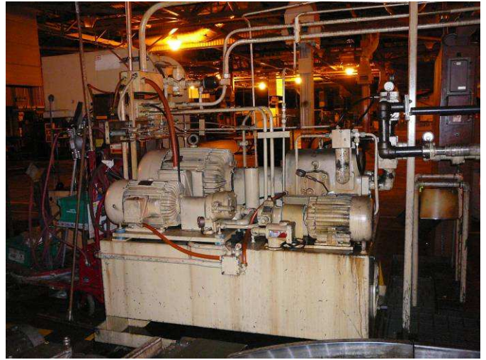
Photo 40. Broach #2 – oil reservoir motors (W-038).
