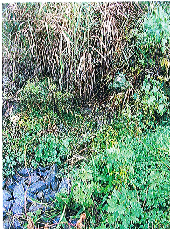
Photograph 18: View of erosion near outlet of CB-1 at Ley Creek bank.
