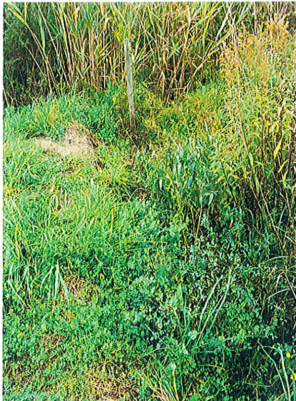
Photograph 6: View of erosion channel near CB-3 along fenceline.
