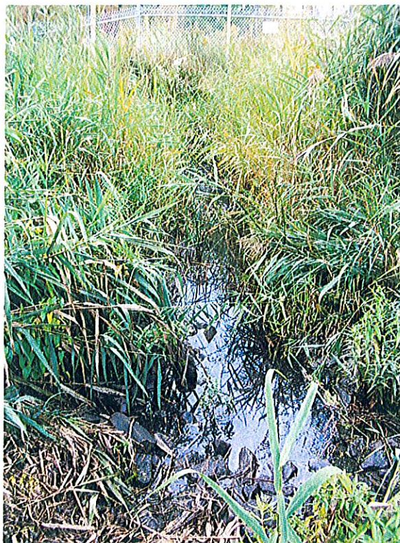
Photograph 8: View looking at CB-3 (clogged grate).
