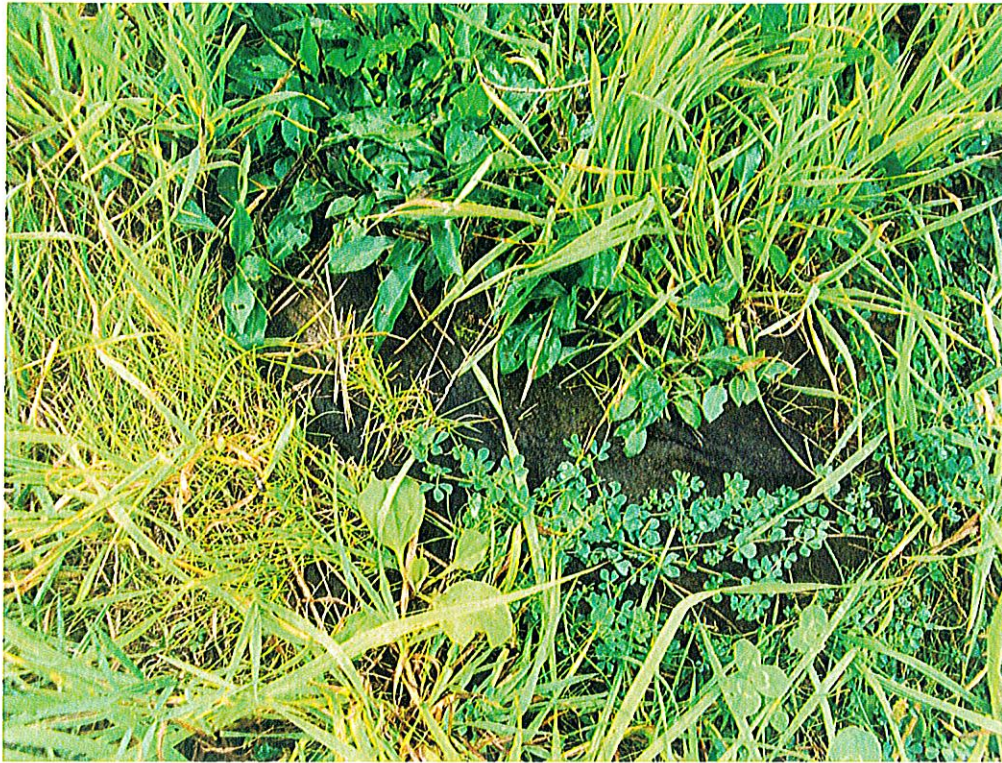
Photograph 9: Non-woven geotextile exposed due to erosion within CB-3 overflow spillway.
