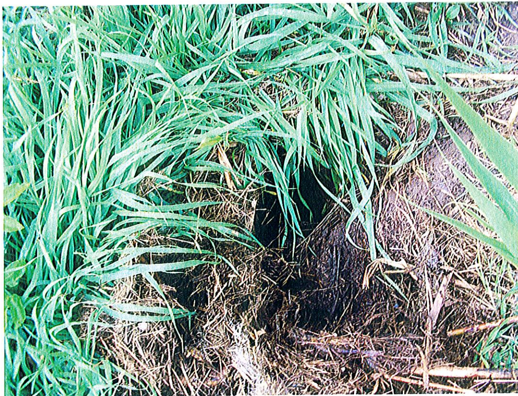
Photograph 20: View of burrowing animal hole at crest of CB-21 overflow spillway slope.
