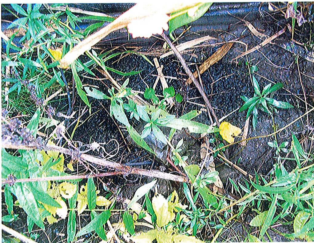
Photograph 17: View of exposed non-woven geotextile fabric along creek bank near CB-1 outlet.
