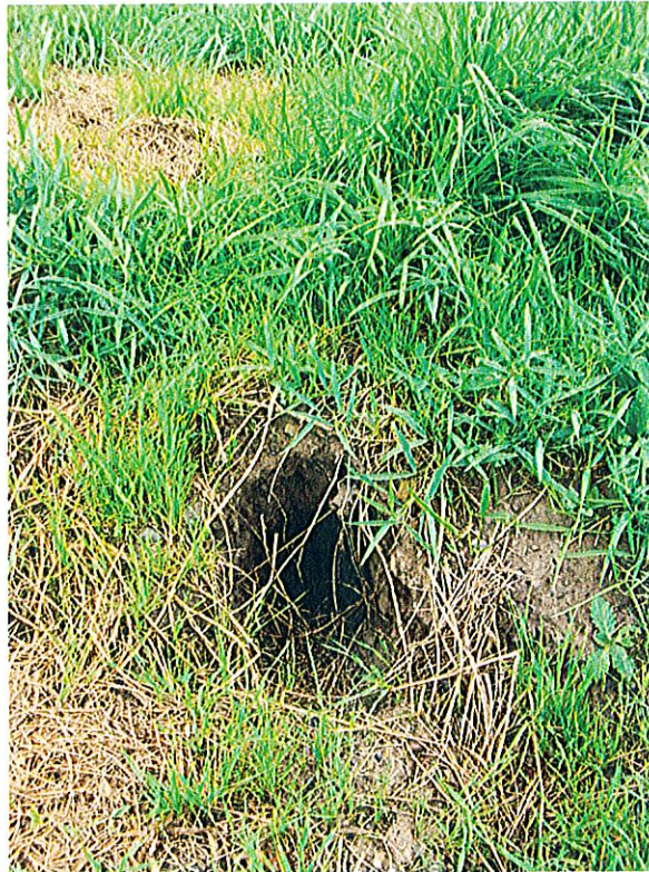
Photograph 12: View of burrowing animal hole at crest of CB-2 overflow spillway slope.
