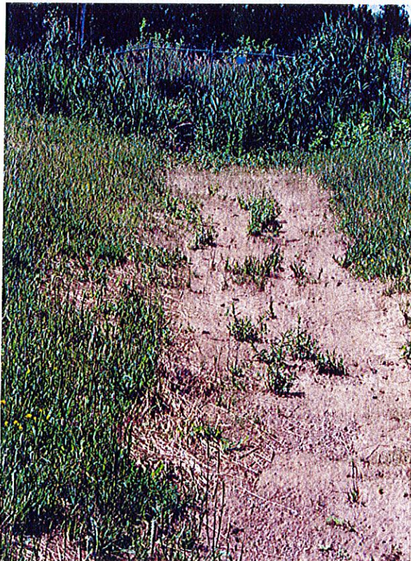
Photograph 6: Newly placed topsoil in CB-3 overflow spillway without vegetation establishment.
