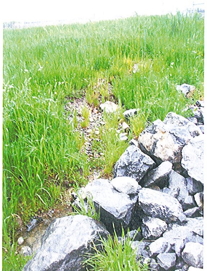
Photograph 32 - View of erosion in CB-4/003 overflow spillway.
