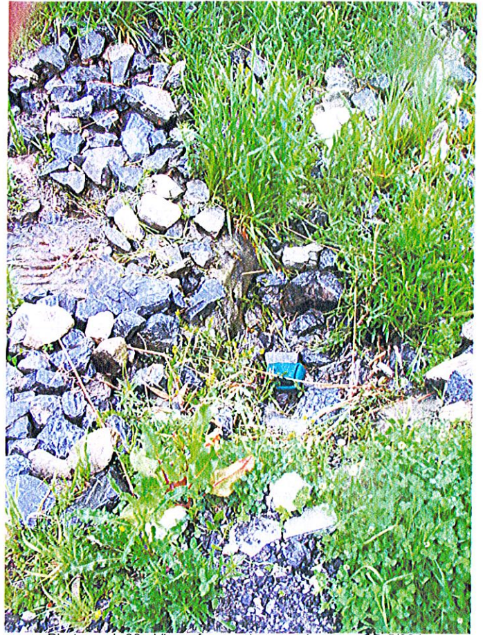
Photograph 30 - View of excessive scouring near CB-5/004.
