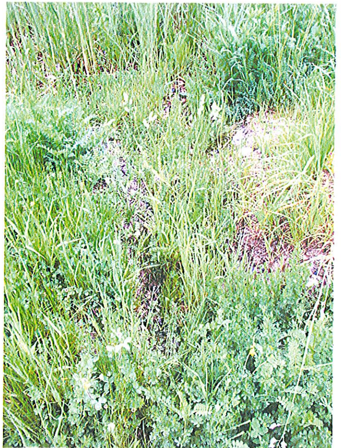
Photograph 20 - View of erosion channel near CB-3.
