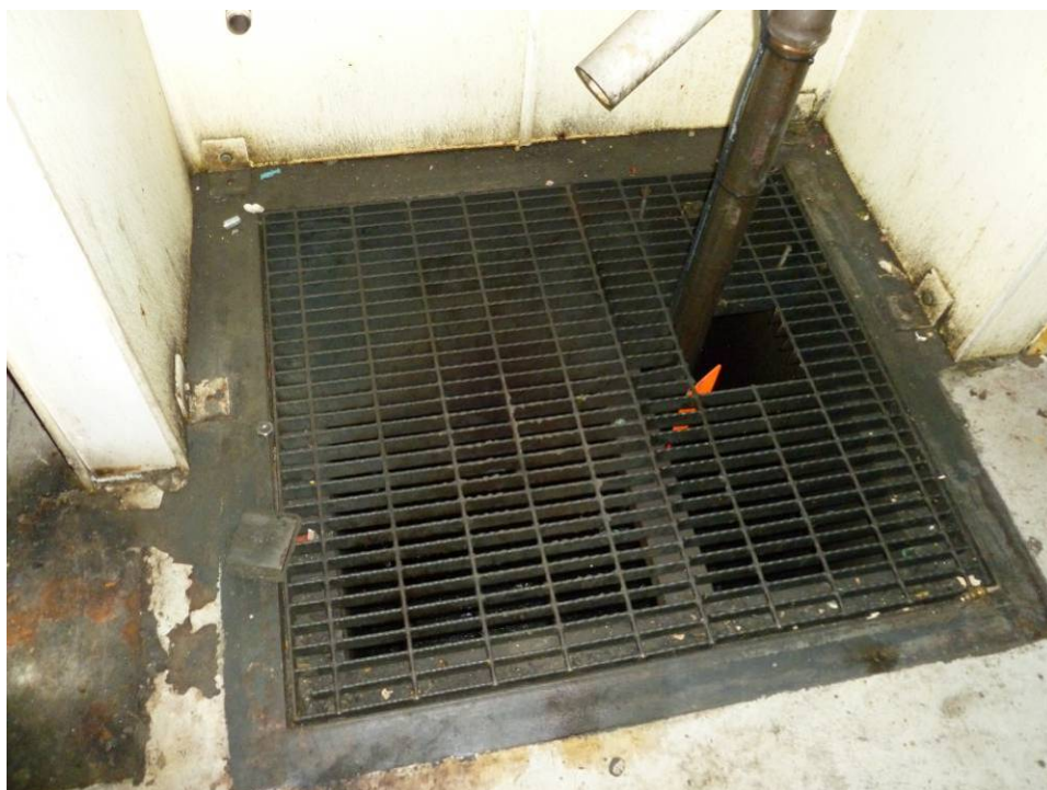
Photograph 68. (AOI-42) Dump Station near Column G2. Oily sludge observed in pit.
