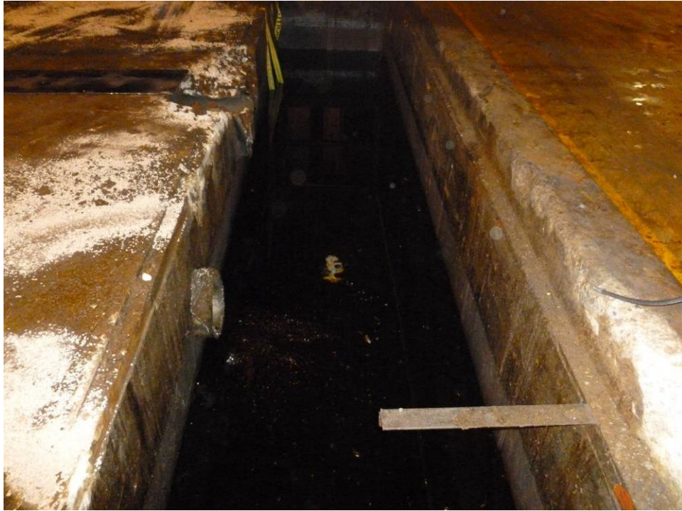
Photograph 79. (AOI-12) Oil-filled pit near Column G4.
