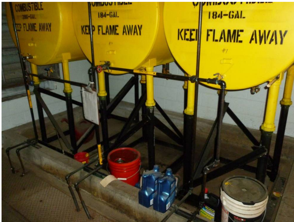
Photograph 38. (AOI-31) Fire Pump House. Three aboveground diesel fuel storage tanks located along interior northeast wall.
