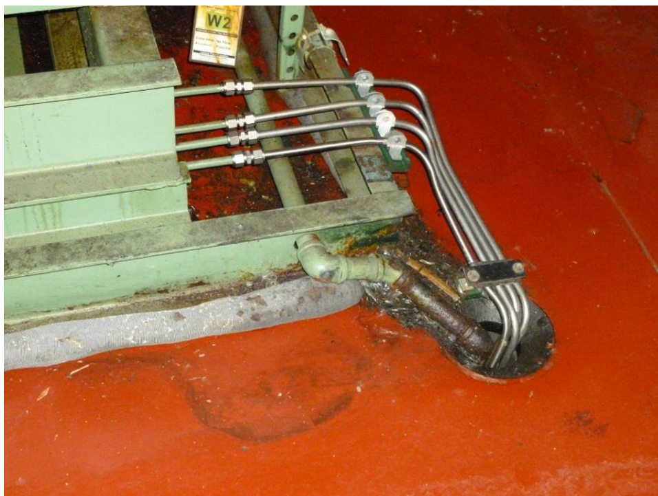
Photograph 113. (AOI-35) Equipment in Air Compressor Building. Lines extending from equipment located in northeast area of building to drain. Note dark staining and oily residue.
