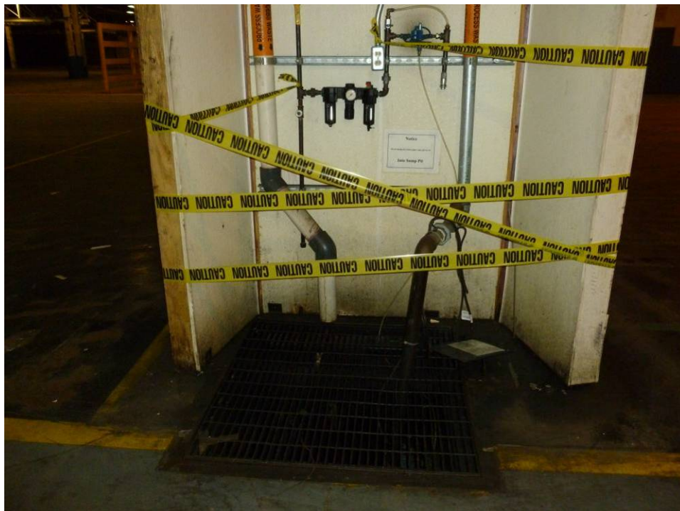
Photograph 67. (AOI-16) Dump Station near Column M/1A. Appears to be routed to process waste. Oily sludge observed in pit.
