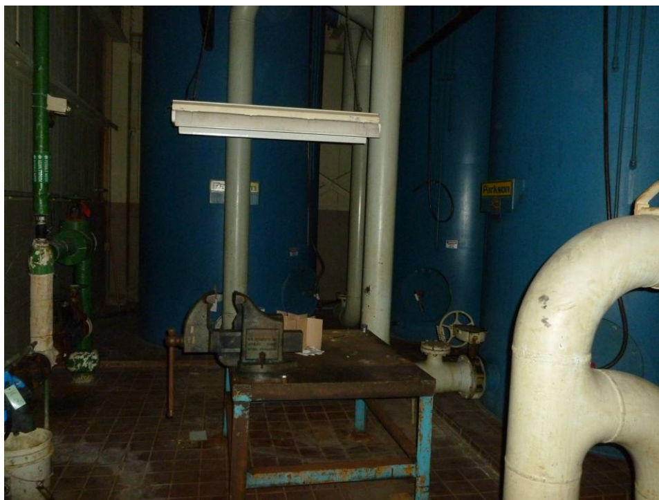
Photograph 121. (AOI-36) Parkson Lamella System. Bulk process tanks located east of the Oil Storage Building, west of the Less Than 90-Day Hazardous Waste Storage Area (AOI-34).
