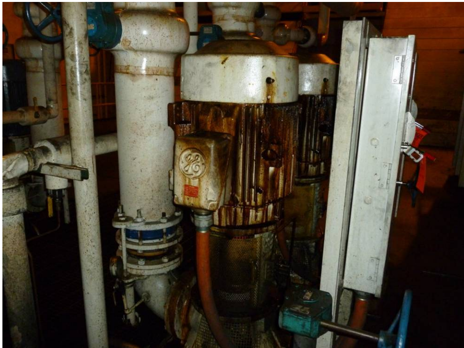
Photograph 14. (AOI-06) West Gallery. Oily residue on crank shaft machining equipment.
