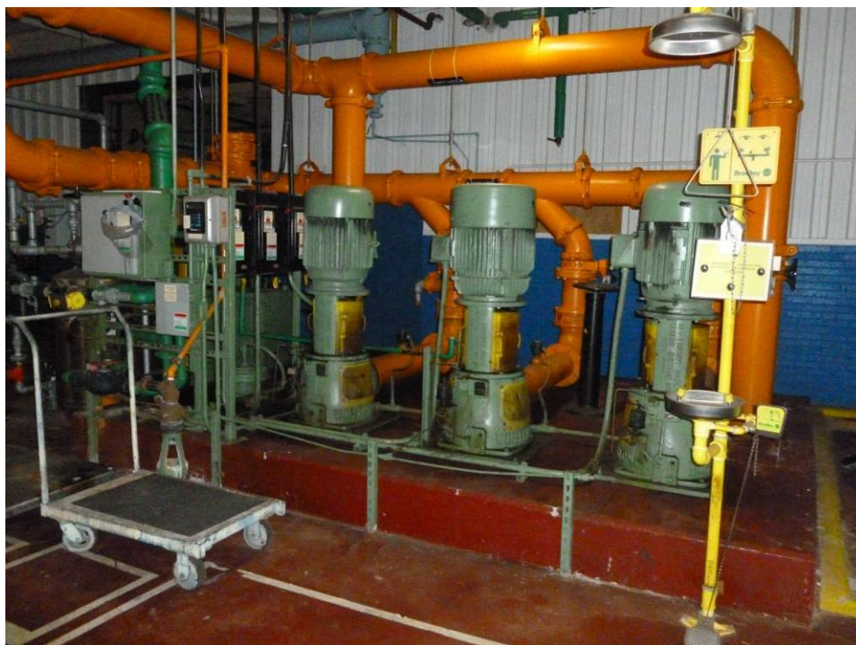
Photograph 111. (AOI-35) Equipment in Air Compressor Building. Photo taken facing south wall of building. Note dark staining and oily residue on elevated concrete platform.
