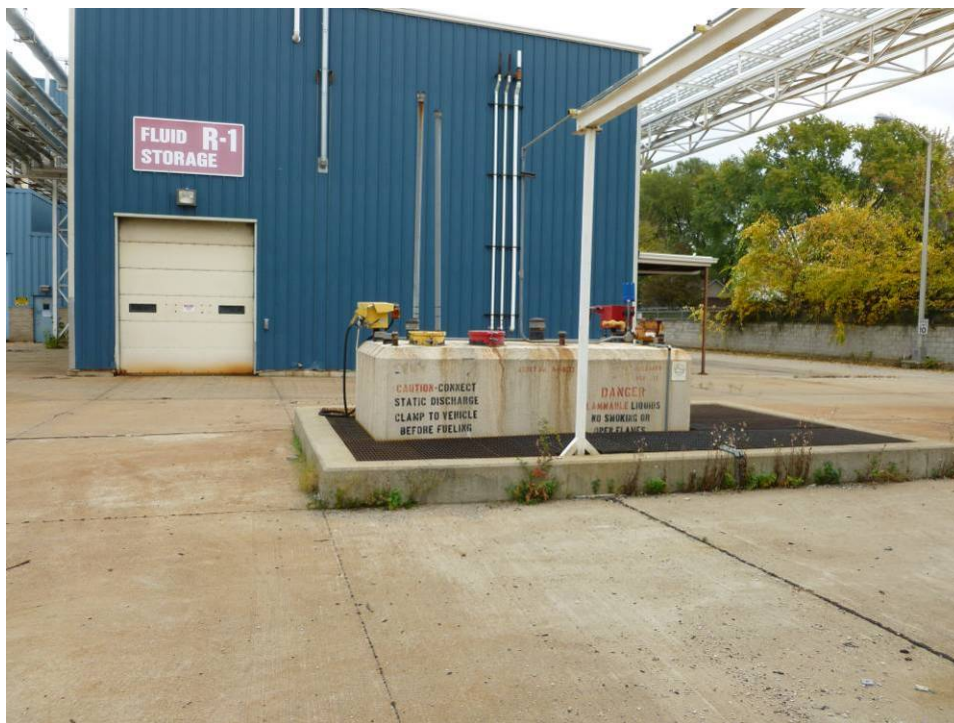
Photograph 107. (AOI-37) Two Aboveground Storage Tanks. Photo taken facing east. Tank at north end is labeled, "Diesel 200 Gallons." Tank at south end is labeled, "Unleaded 800 Gallons." Note Fluid Storage Building aka Oil Storage Building (AOI-36) in the background.
