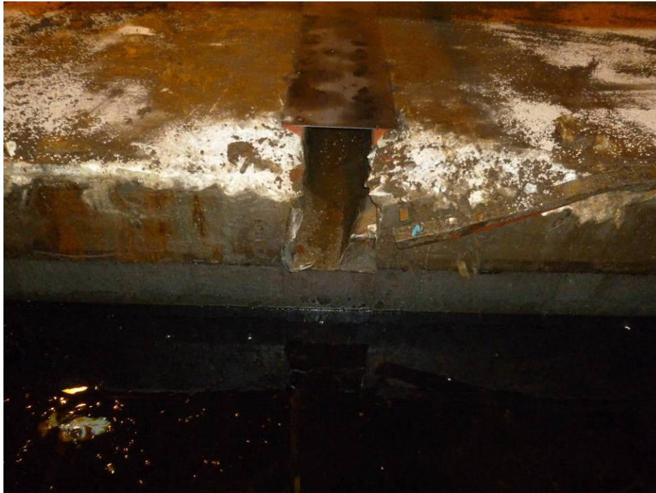
Photograph 81. (AOI-12) Oil-filled pit near Column G4.
