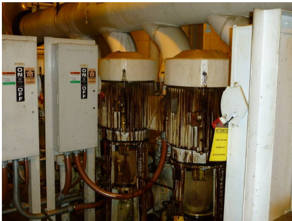
Photograph 5. (AOI-02) South Gallery, east side. Oily residue on block grinding equipment. Oily residue also observed on floor surrounding equipment.
