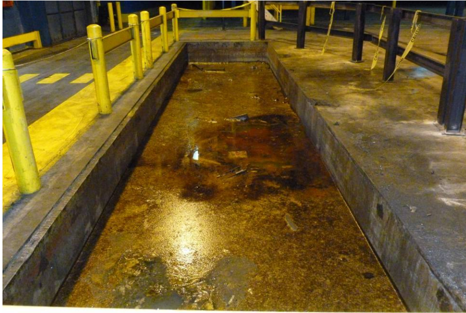
Photograph 29. (AOI-14) Equipment Pit near Columns A3/A2. Note oily coolant/water remaining in pit. Photo taken facing south.
