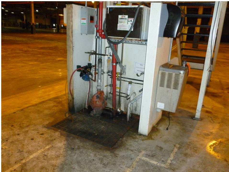
Photograph 84. (AOI-11) Dump Station near Columns J5/K5.
