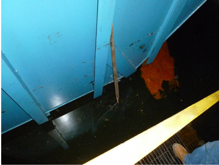
Photograph 1. (AOI-02) South Gallery, west side, sub-basement. Note level of water accumulated in basement, approximately 12" to 18" deep with possible oil and coolant content.
