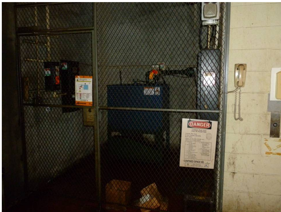
Photograph 19. (AOI-33) Control room for WWTP elevator.
