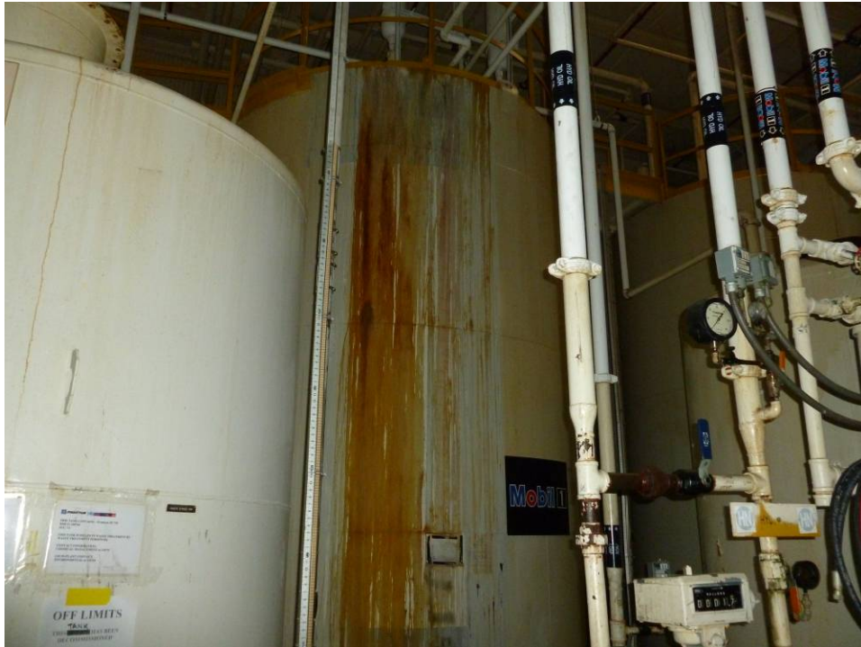
Photograph 120. (AOI-36) Oil Storage Building. Note staining on bulk engine oil storage tank. Unknown whether rust or oily staining at time of site reconnaissance.
