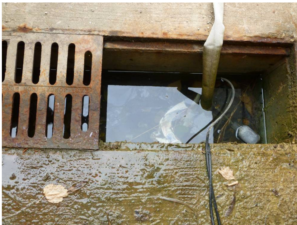
Photograph 46. (AOI-25) Purple dock. Blind trench exterior to dock area. Minor sheen observed.
