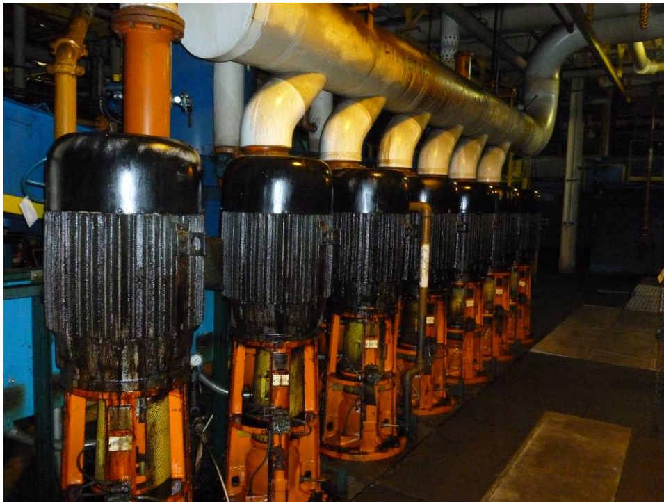
Photograph 2. (AOI-02) South Gallery, west side. Oily residue on honing/chip processing equipment. Oily residue also observed on floor surrounding equipment.
