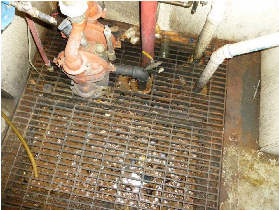
Photograph 83. (AOI-11) Dump Station near Columns J5/K5. Note, the pit is filled with oily / coolant sludge.
