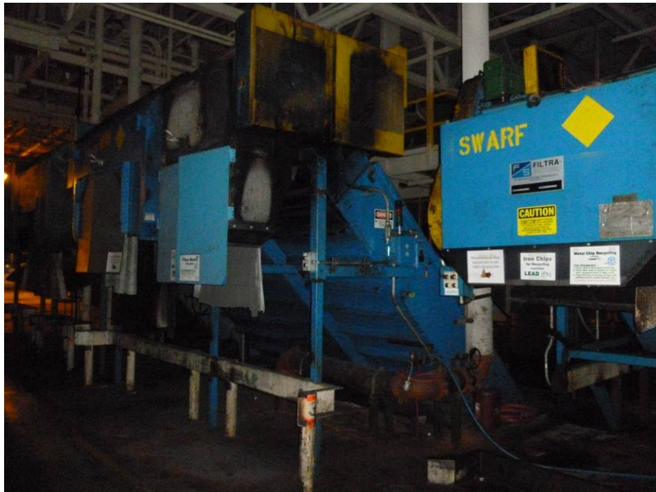
Photograph 91. (AOI-04) Swarf management associated with East Gallery (AOI-04). Located on main level of Plant. Note signage: "Iron Chips for Recycling Contain Lead."
