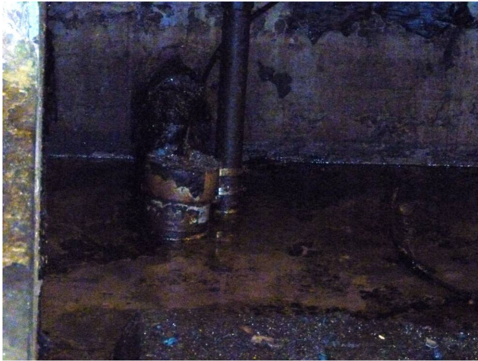
Photograph 77. (AOI-12) Oil-filled trench/flume located approximately 25 feet from equipment pit, extending approximately 100 feet north of the pit. Float observed in northwest corner of pit.
