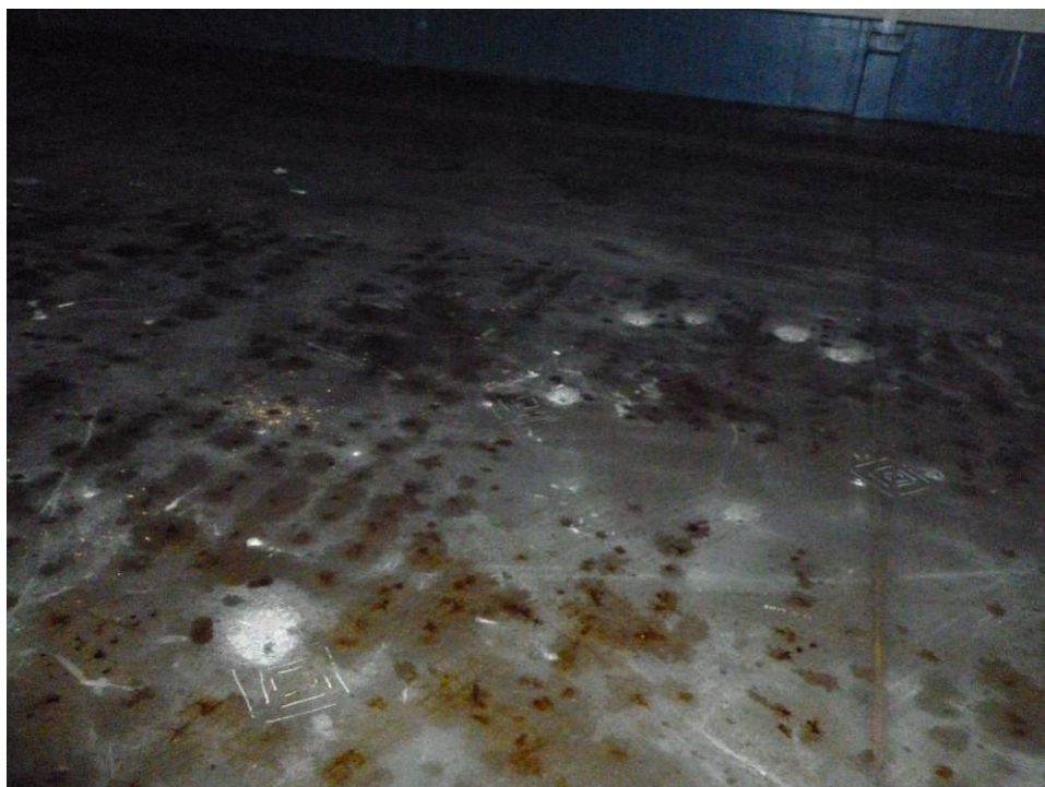
Photograph 43. Northwest area of Plant, area between Columns WB and WJ, facing north wall. Dark brown spots appear to be oily condensate dripping from overhead lines.
