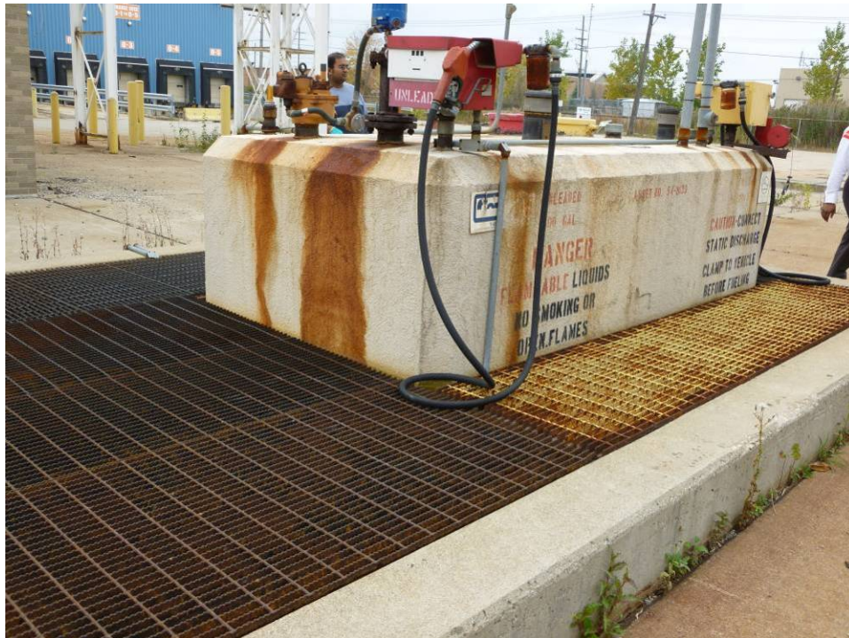
Photograph 109. (AOI-37) Two Aboveground Storage Tanks. No liquids were observed in the containment around the tanks. Photo taken facing northeast.
