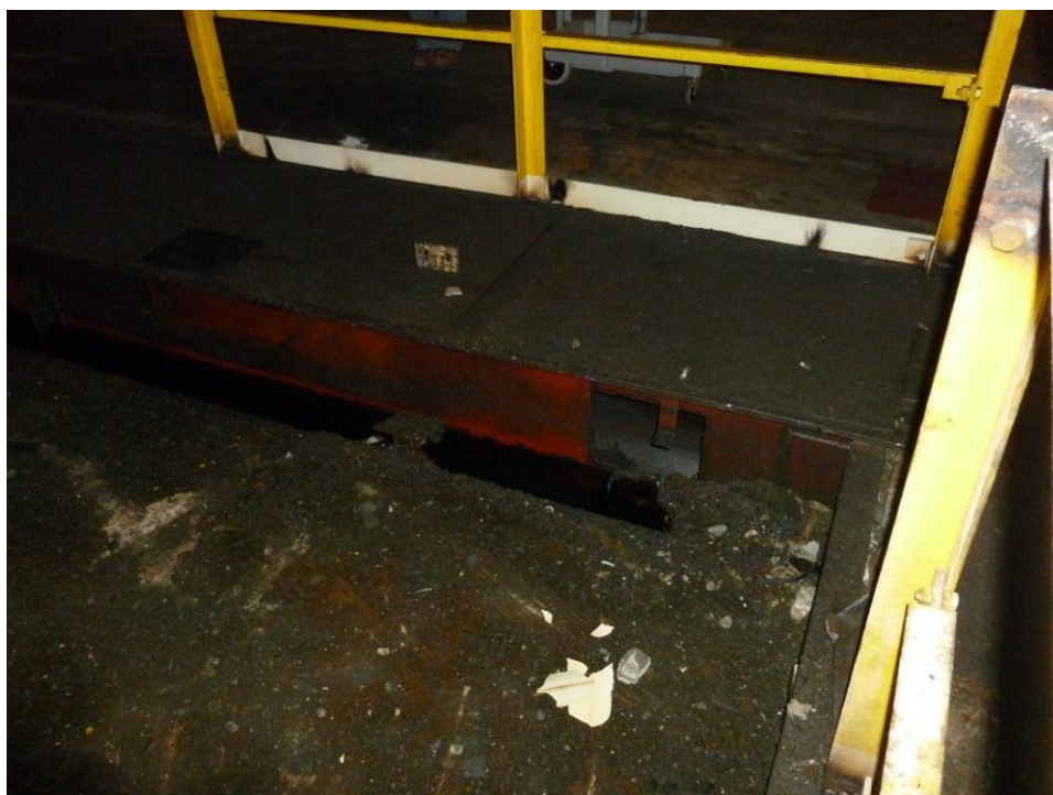
Photograph 70. (AOI-15) Equipment Pit near Columns D2/E2. Dark staining, some debris observed in pit.
