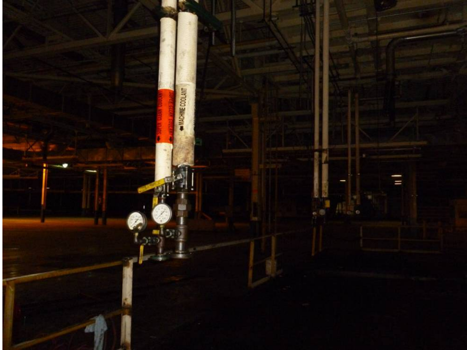
Photograph 71. (AOI-15) Equipment Pit near Columns D2/E2. Coolant lines observed in pit area.
