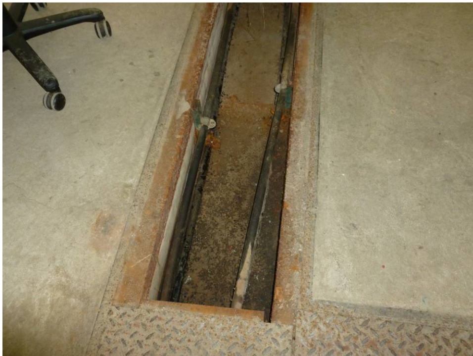
Photograph 42. (AOI-31) Fire Pump House. Trench for electrical conduit. Note dark staining.
