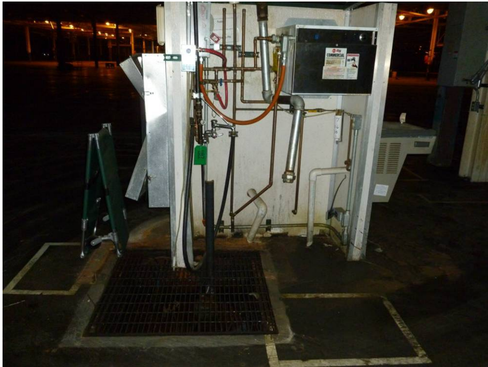
Photograph 55. (AOI-18) Dump Station near Columns 4A/J. Note, this Dump Station appeared to be approximately 1 foot deep and was partially filled with water.
