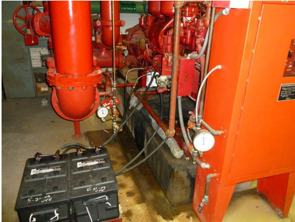
Photograph 41. (AOI-31) Fire Pump House. Fire pump engine #3. Note oily staining.
