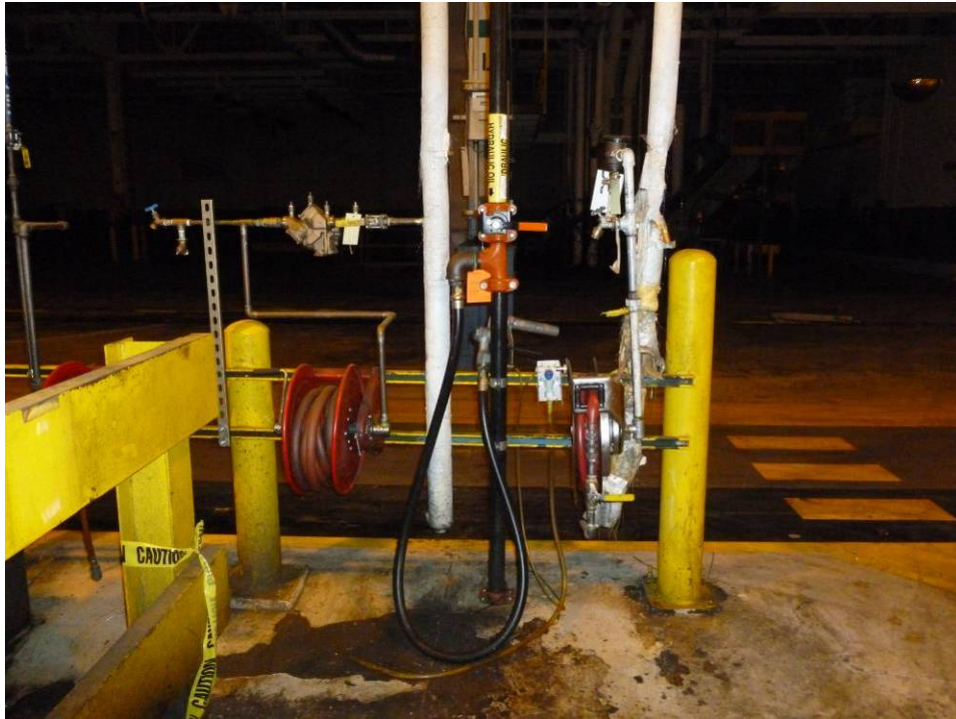
Photograph 93. (AOI-15) Clean / Dump Station near Column L14. Hot and cold water lines, compressed air lines, and a hydraulic oil dispensing unit were observed at this station.
