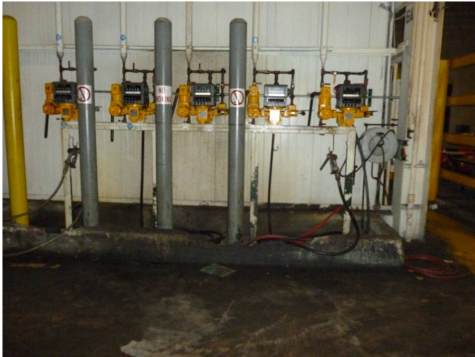
Photograph 66. (AOI-19) Oil Pump Station located adjacent to trash compactor area along east wall of Plant. Note dark staining / oily residue on concrete berm and floor. Five dispensing units.
