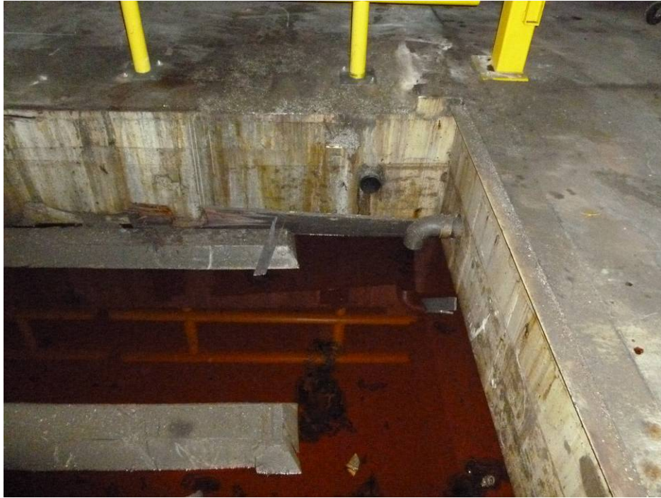
Photograph 35. (AOI-41) Equipment Pit near Columns A7/A6. South end of pit. Note outfalls in southeast corner and several inches of oily/coolant water.
