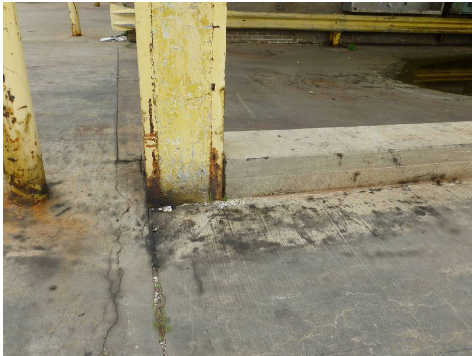
Photograph 23. (AOI-33) Wash pad located exterior to WWTP, north. Note staining.
