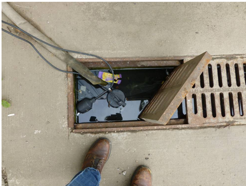
Photograph 58. (AOI-20) Orange dock exterior. Blind trench beneath truck bays contained water. Negligible amount of sheen observed.
