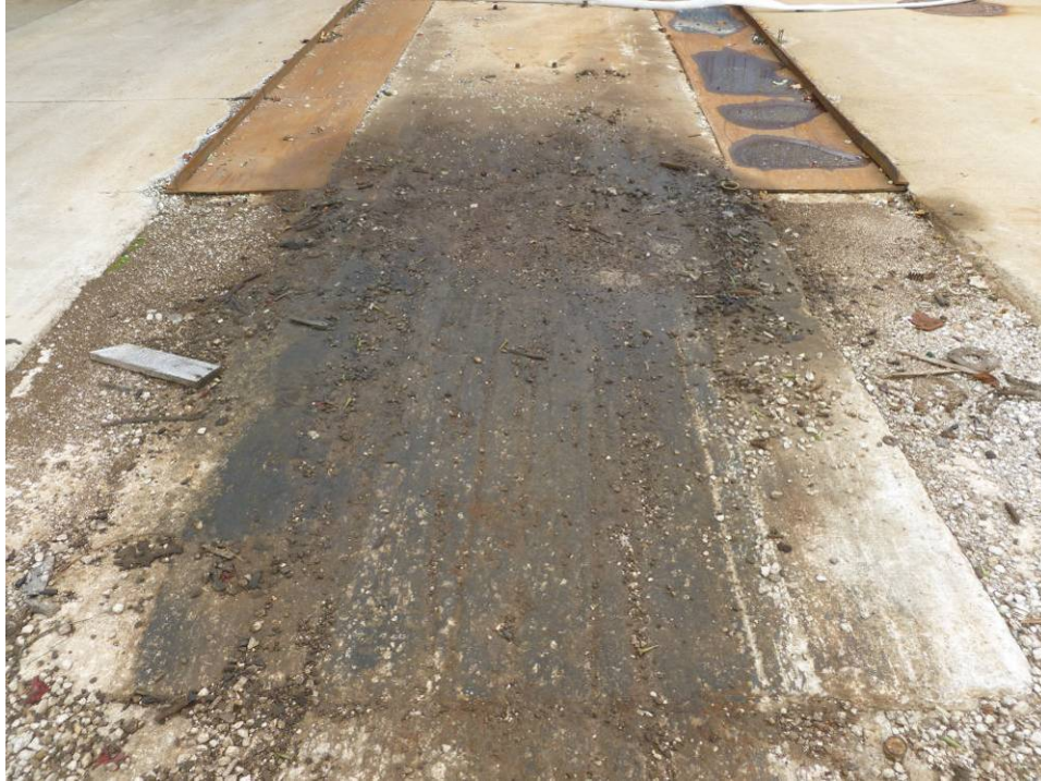
Photograph 61. (AOI-19) Trash compactor area exterior. Close-up of dark staining / oily residue. Pools of liquid on metal rails are likely result of recent precipitation event. No sheen was observed on the water.
