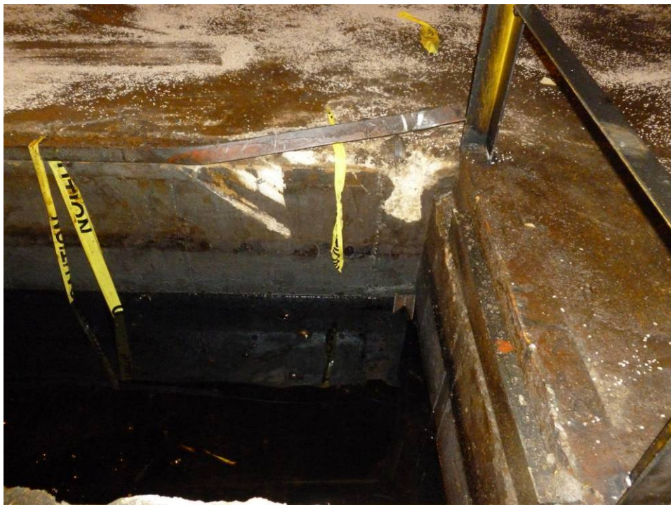
Photograph 82. (AOI-12) Oil-filled pit near Column G4.
