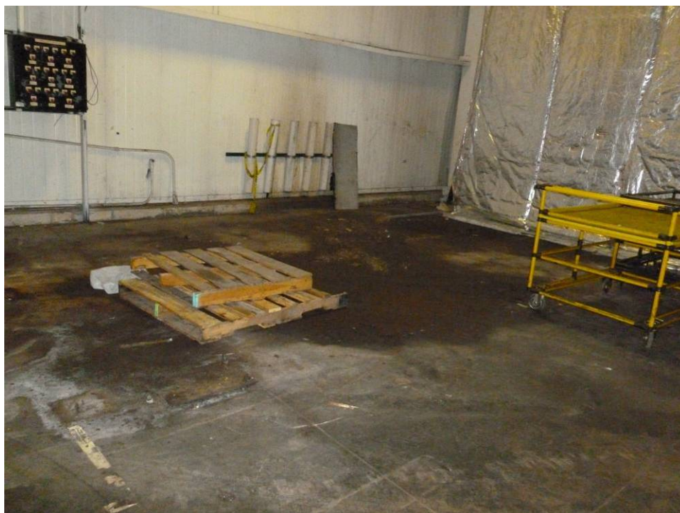
Photograph 64. (AOI-19) Trash compactor area interior. Note dark staining / oily residue. Photo taken facing northeast.
