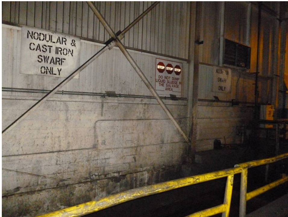
Photograph 103. (AOI-01) Truck Bay. Photo taken facing south wall of Plant. Note dark staining on wall. Dark staining was also observed on the floor of the Truck Bay.
