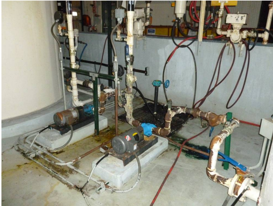
Photograph 117. (AOI-36) Oil Storage Building. Photo taken from inside area of secondary containment, facing north. Note sump and evidence of release (blue colored material on/beneath pipes east of sump).
