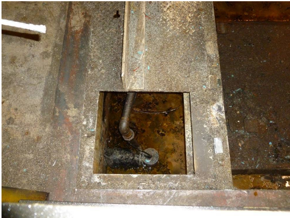
Photograph 78. (AOI-12) Oil-filled trench / flume system, may be associated with equipment pit.
