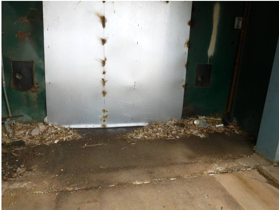
Photograph 62. (AOI-19) Trash compactor area exterior. Bay entrance to building. Photo taken exterior to bay, facing west. Note dark staining / oily residue on concrete pad.
