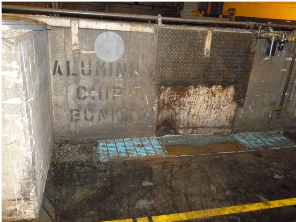
Photograph 100. (AOI-01) Chip Bunkers. Close-up of aluminum chip bunker. Photo taken facing south.
