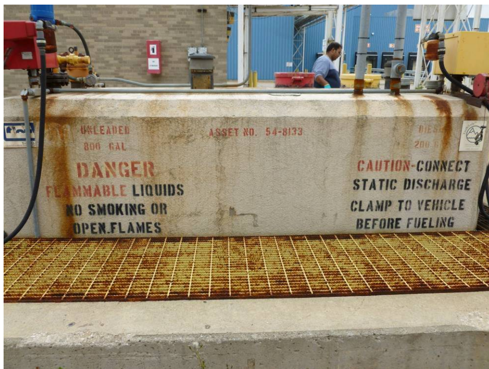
Photograph 108. (AOI-37) Two Aboveground Storage Tanks. Photo taken facing west.
