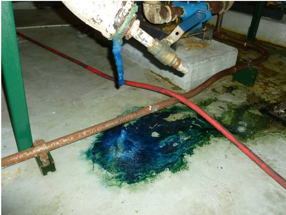
Photograph 118. (AOI-36) Oil Storage Building. Evidence of release from caustic product tank.
