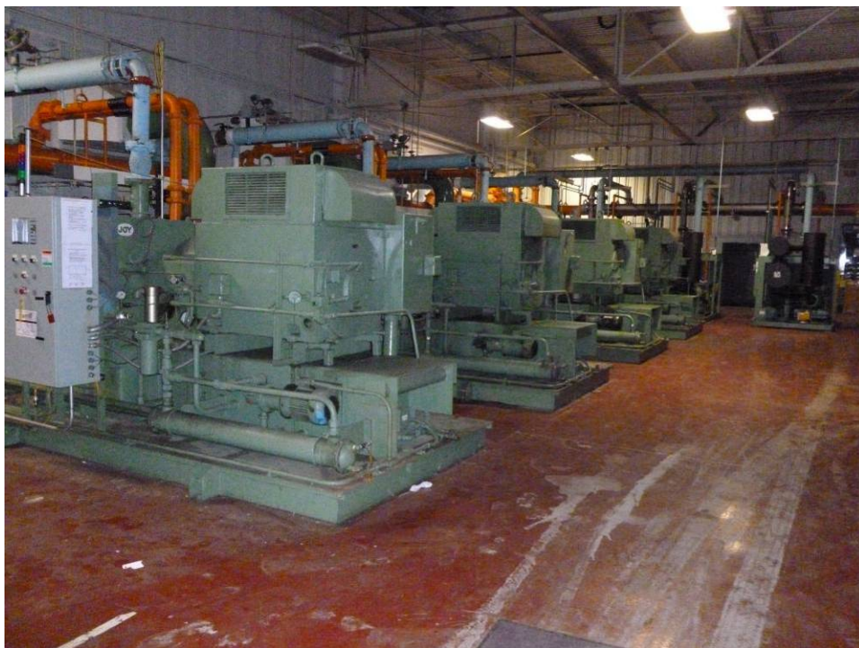
Photograph 112. (AOI-35) Equipment in Air Compressor Building. Photo taken facing northeast.
