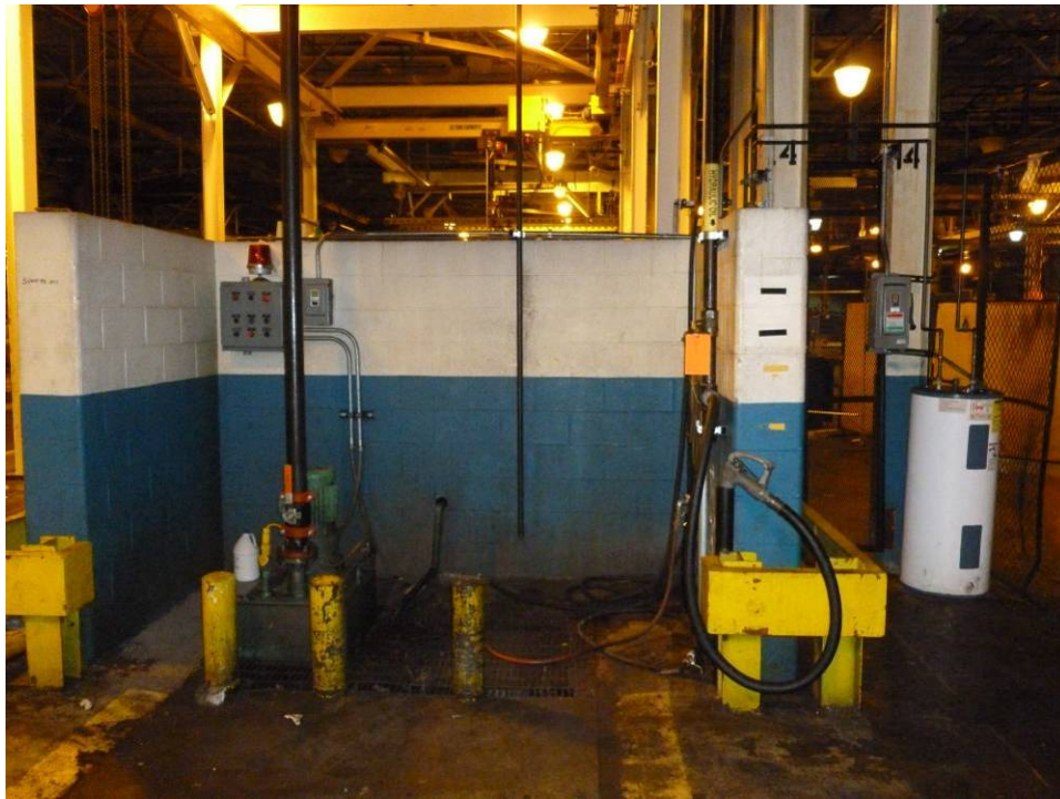
Photograph 105. (AOI-07) Dump Station near Column E14. Note hydraulic oil distribution line. Oily material was observed in the pit at the time of the site reconnaissance.
