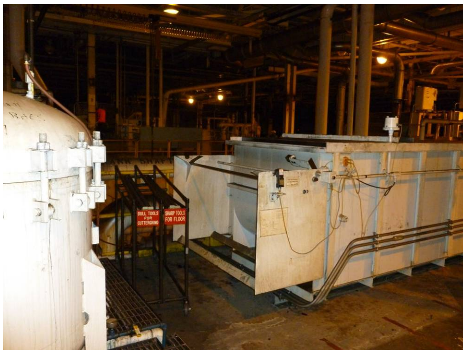
Photograph 16. (AOI-06) Equipment in West Gallery.
