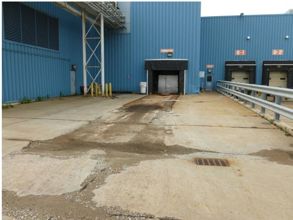
Photograph 60. (AOI-19) Trash compactor area exterior. Note storm drain in northeast area of compactor bay. Note deteriorated condition of concrete.
