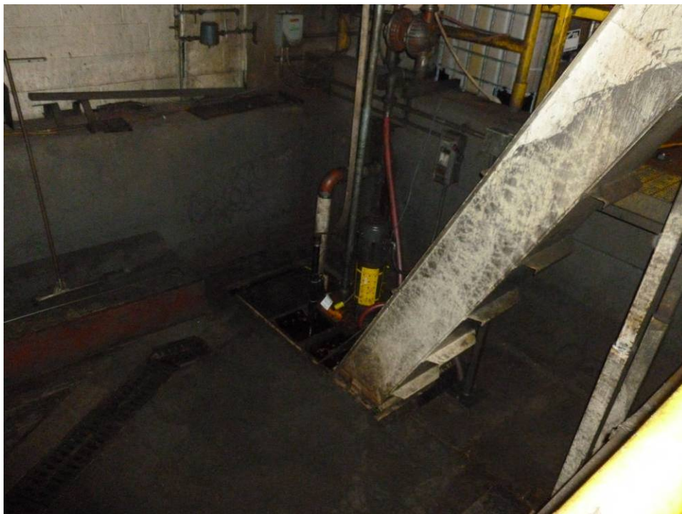
Photograph 102. (AOI-01) Chip Management Area. Conveyance is located at the west end of the Truck Bay. Note sump and pump. Photo taken facing south wall of Plant.
