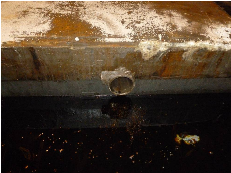
Photograph 80. (AOI-12) Oil-filled pit near Column G4.
