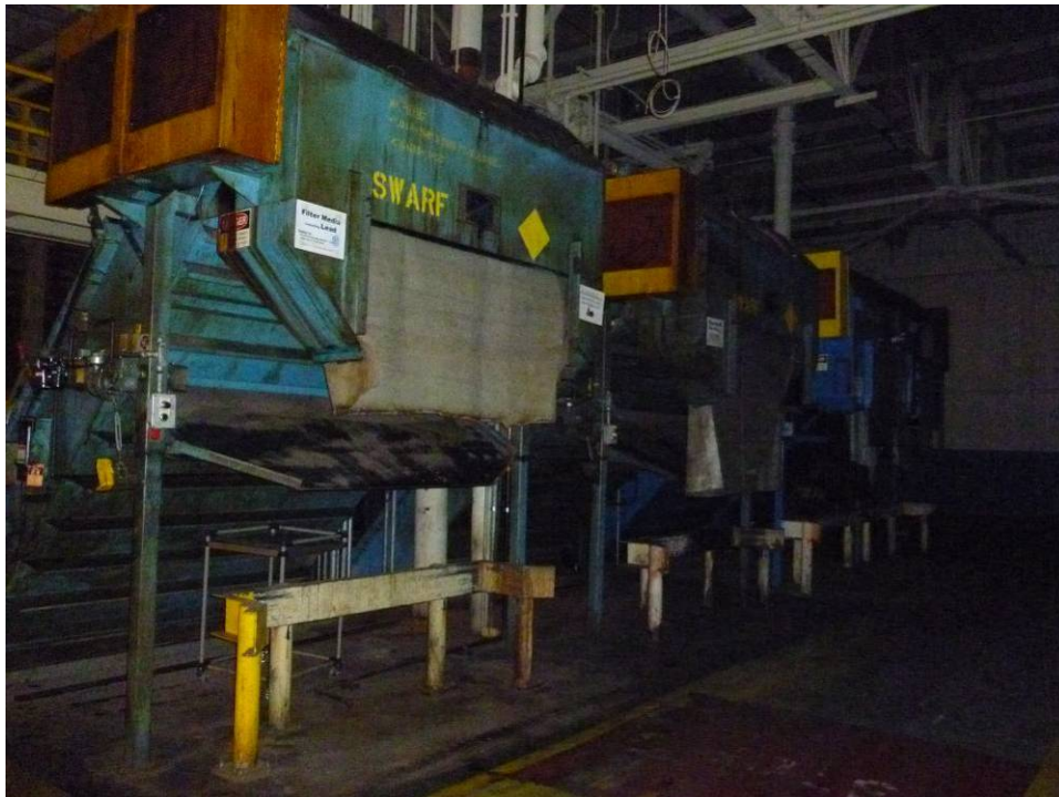
Photograph 90. (AOI-04) Swarf management associated with East Gallery (AOI-04). Located on main level of Plant. Note signage: "Filter Media Contains Lead."
