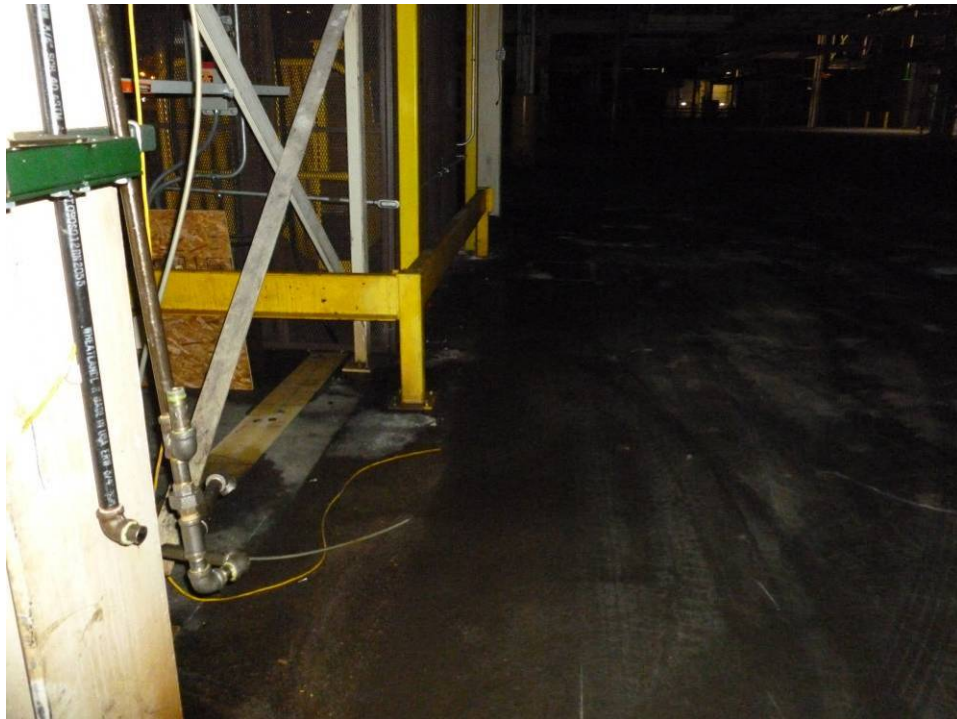
Photograph 53. (AOI-21) Oily staining near oil dispensing ports at heavy equipment lift. Near Columns 6A/K.
