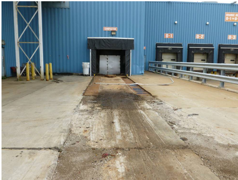
Photograph 59. (AOI-19) Trash compactor area exterior. Photo taken facing west. Note dark staining / oily residue at east end of trash compactor bay. Note deteriorated condition of concrete.
