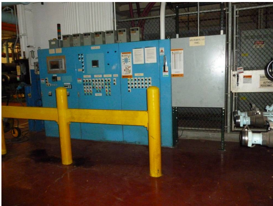
Photograph 114. (AOI-35) Substation located between Air Compressor Building and Wastewater Treatment Plant.
