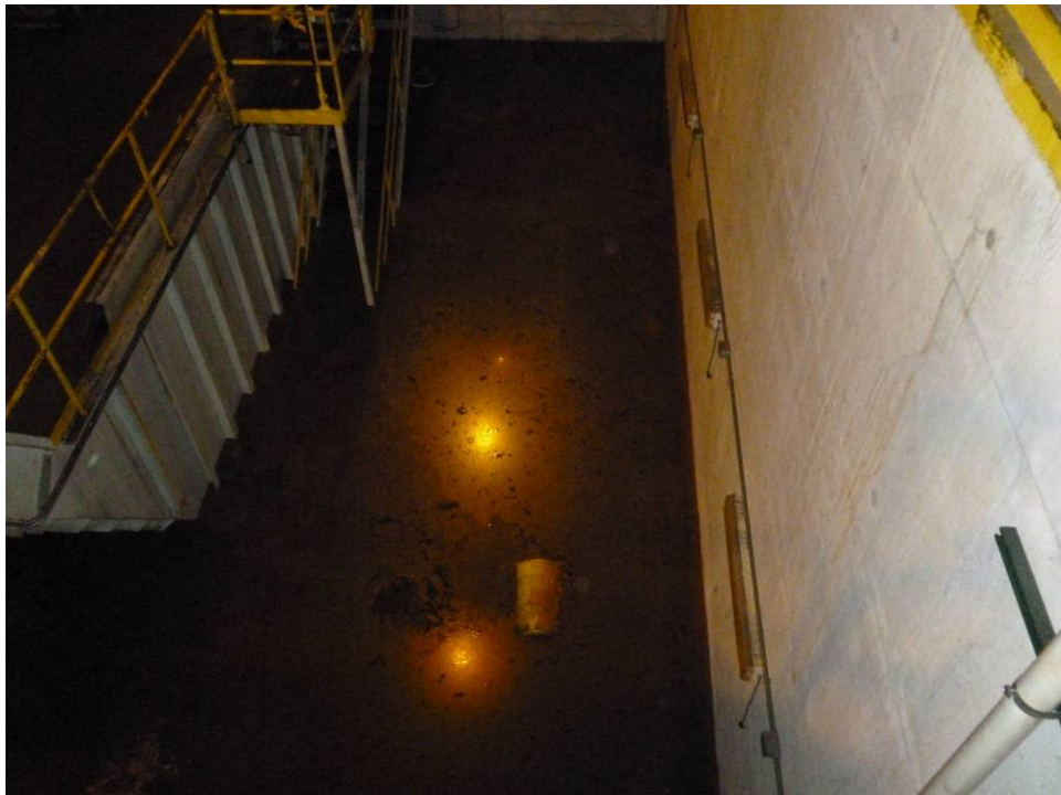
Photograph 12. (AOI-06) West Gallery. Note accumulation of water, possibly containing oil and coolants.
