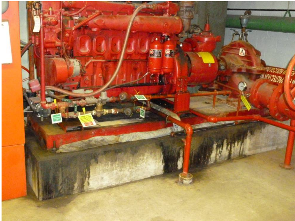
Photograph 40. (AOI-31) Fire Pump House. Diesel fire pump engine #3. Note oily staining beneath engine and blow down/condensate drain in foreground.
