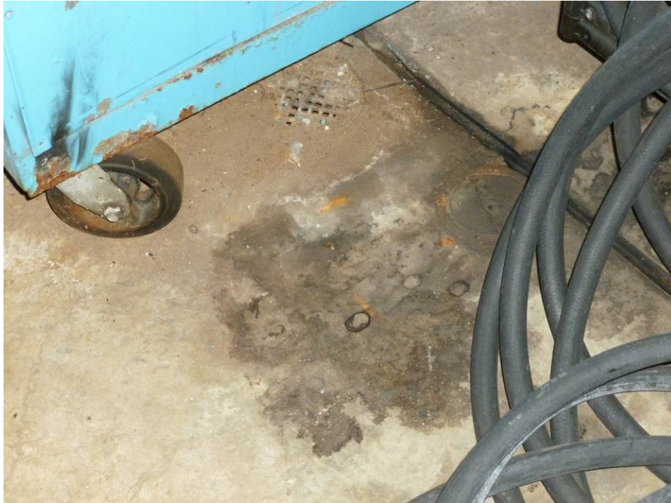
Photograph 39. (AOI-31) Fire Pump House. Oily staining on concrete floor near floor drain, located in northwest area of building.
