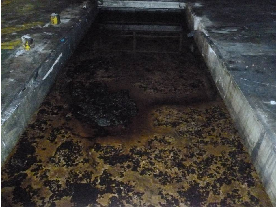
Photograph 85. (AOI-10) Equipment Pit. Note pit contains approximately 3 feet of oily / coolant water.
