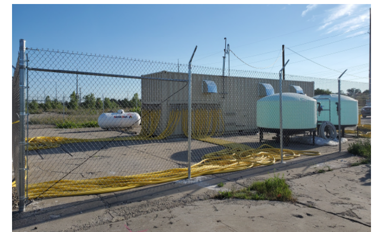
Plant 2 Biosparge Unit and Nutrient Injection Tanks
